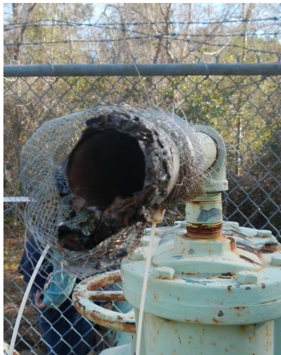
Photograph 10: Well 6 - Blowoff pipe corrosion
