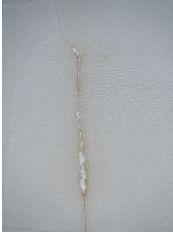
Photograph 15: Ground storage tank with cracked exterior
