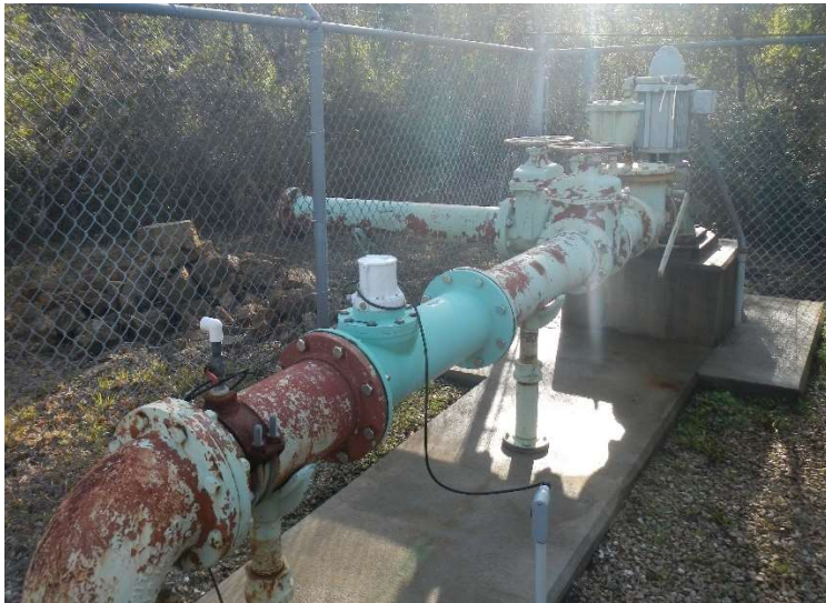
Photograph 12: Well 7 – Water accumulation on pad
