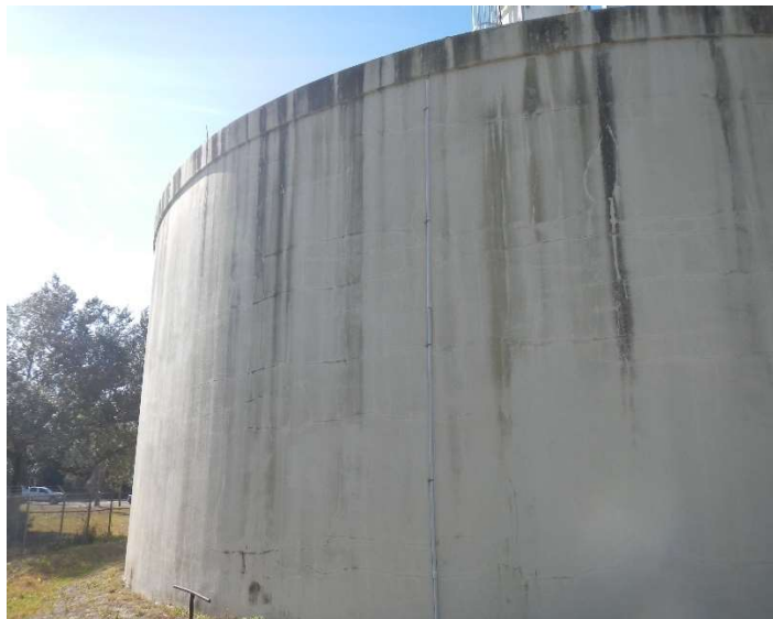
Photograph 14: Ground storage tank with cracked exterior
