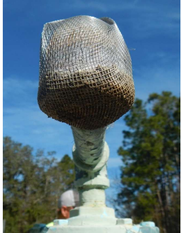
Photograph 9: Well 5 Blowoff pipe corrosion
