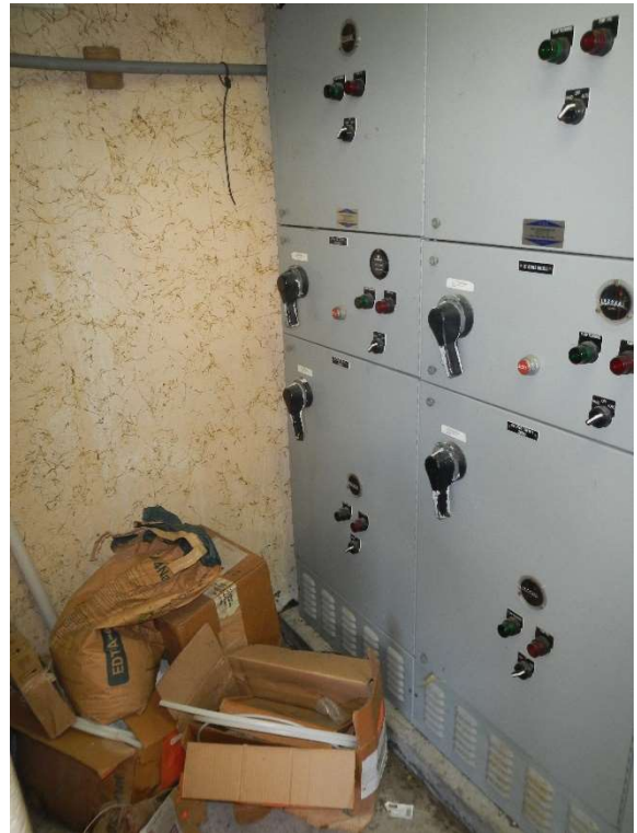
Photograph 2: Water Treatment Plant Control Room
