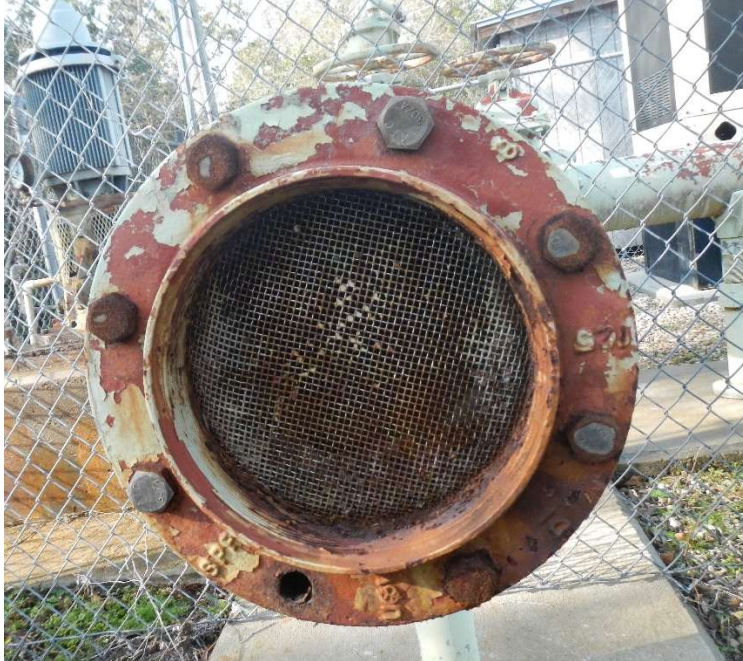
Photograph 11: Well 6 - Overflow pipe connecting plate
