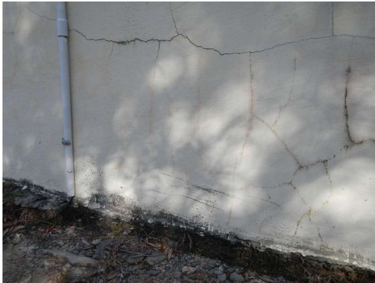
Photograph 16: Ground storage tank deteriorated concrete base
