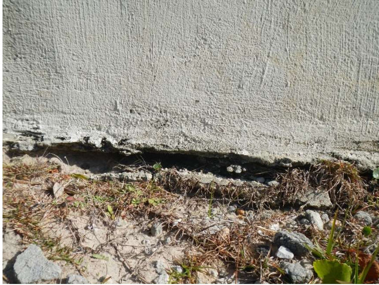
Photograph 17: Ground storage tank concrete base lacking seal
