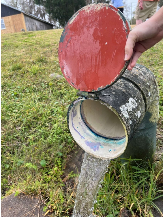
Photograph 8: Overflow pipe at Elevated Storage Tank Provided by FDEP staff – taken on February 3, 2022
