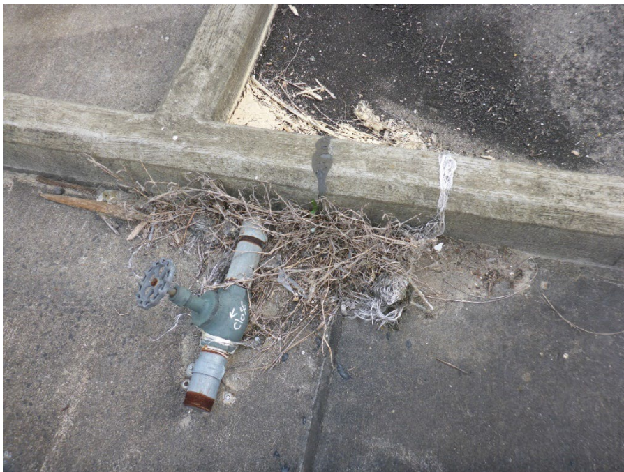
Photo 3: Grass observed growing in a crack on the DLA Pad.
