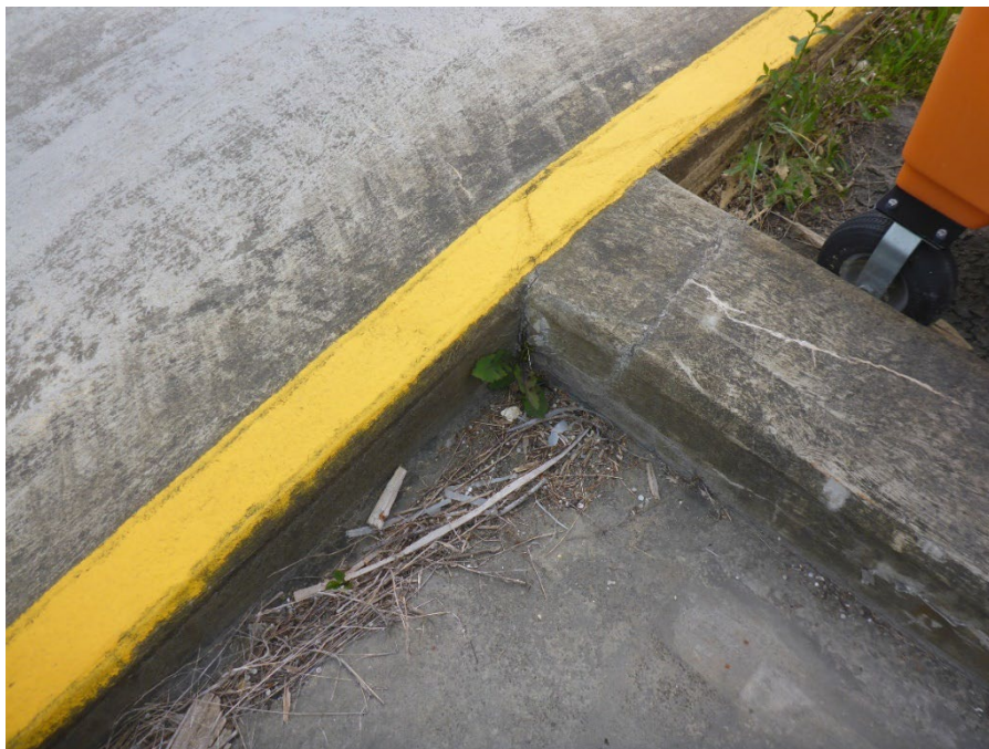
Photo 6: Grass observed growing in a crack on the DLA Pad.
