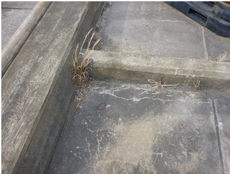
Photo 2: Grass observed growing in a crack on the DLA Pad.
