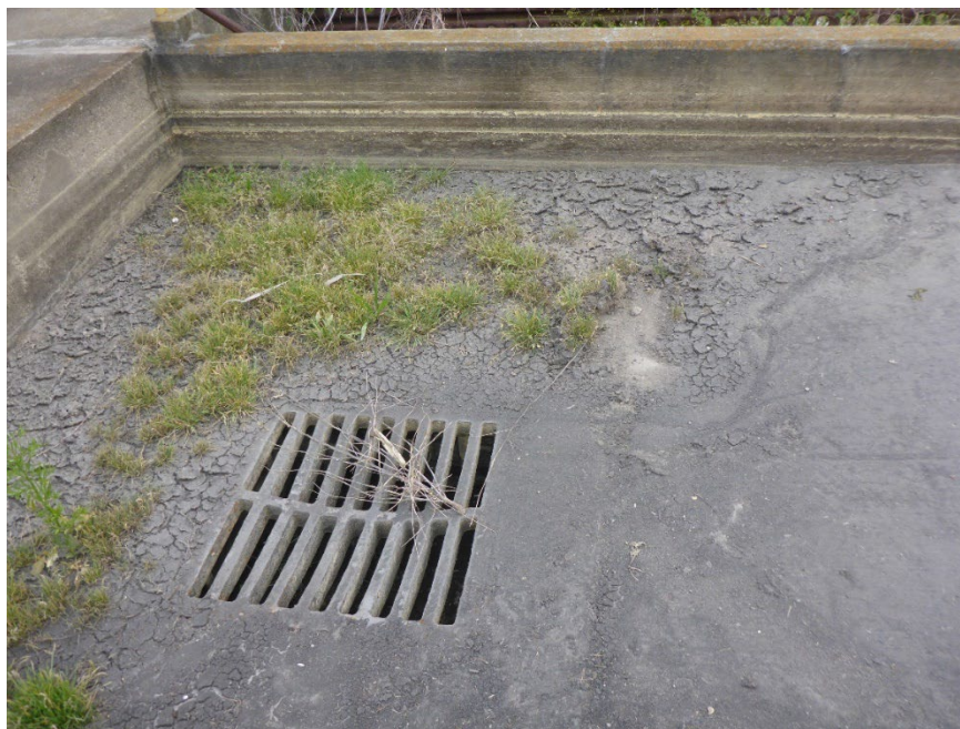
Photo 9: Accumulation of dirt and weeds observed on the concrete at the DLA Pad. Scuff mark to verify that concrete is beneath the dirt.
