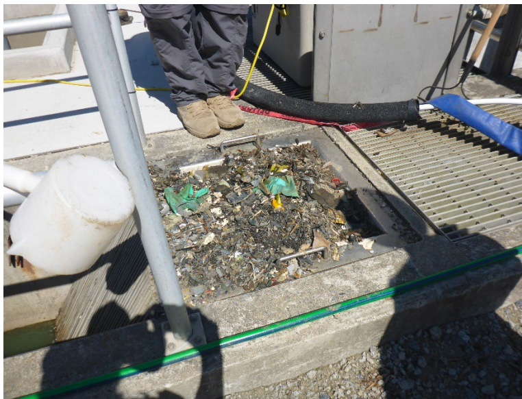
Photo 16: F002 / F003 / F006 / F009 / F019 hazardous waste debris accumulating on a metal grate at the IWTP headworks rather than in a container.
