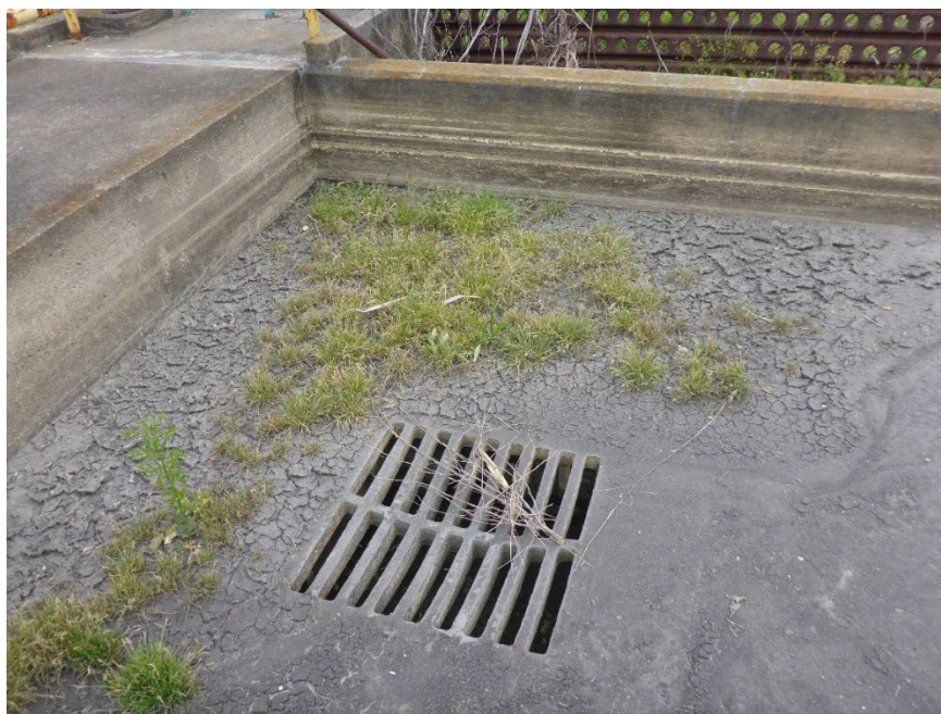
Photo 8: Accumulation of dirt and weeds observed on the concrete at the DLA Pad.
