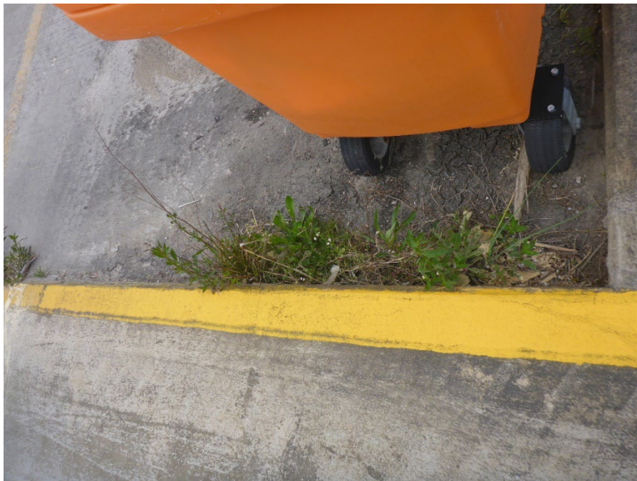
Photo 7: Grass observed growing in a crack on the DLA Pad.
