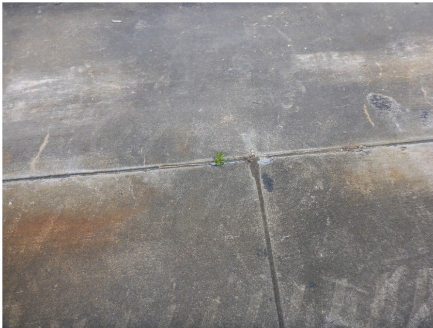
Photo 4: Grass observed growing in a crack on the DLA Pad.
