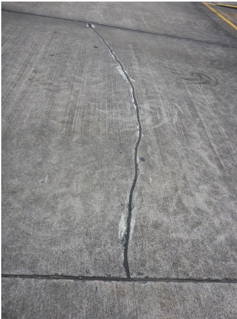
Photo 5: Crack observed on the DLA Pad.
