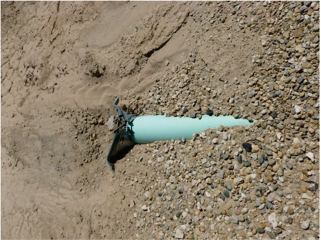
Photo 2 / P1000865 – Detention Pond Inlet
