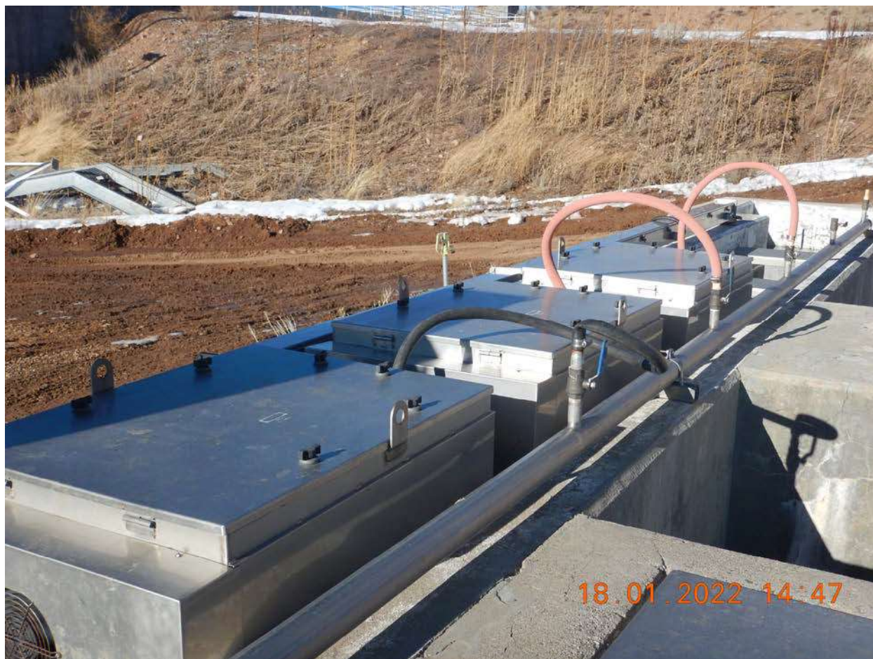
Another view of the UV disinfection system. (DSCN2089). Photographed by D. Esparza
