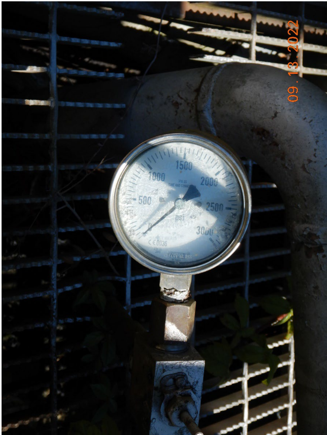
Photograph 3: Looking north, closeup view of surface casing pressure gauge. Pressure reading is 0 psi.
