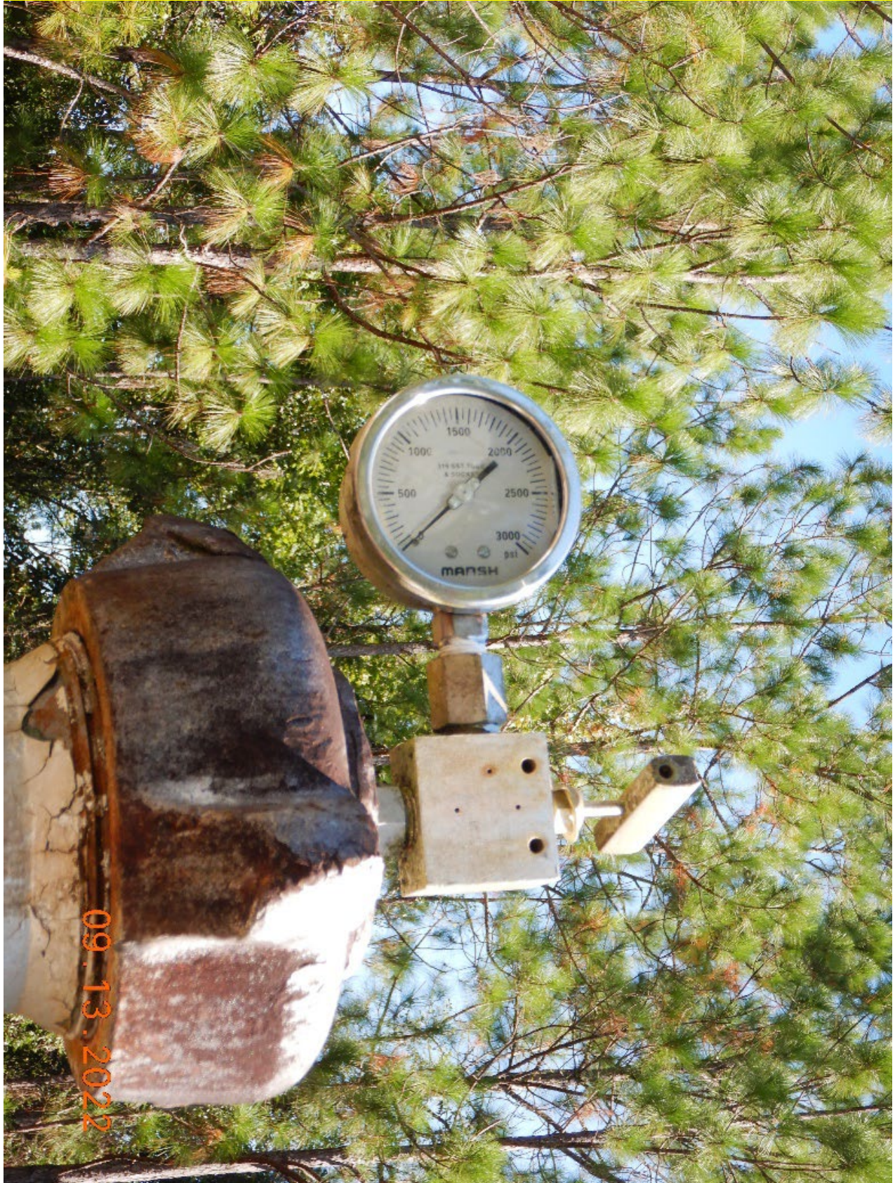
Photograph 5: Looking north, closeup view of internal pressure gauge reading 0 psi.
