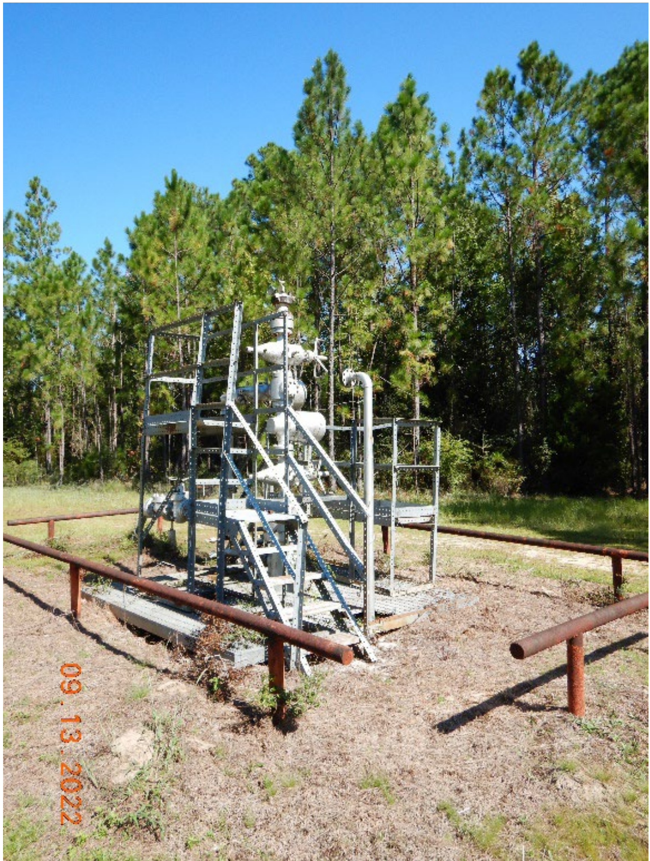
Photograph 2: Looking west, site overview, including well head, pressure gauges, valves, and access stairs.
