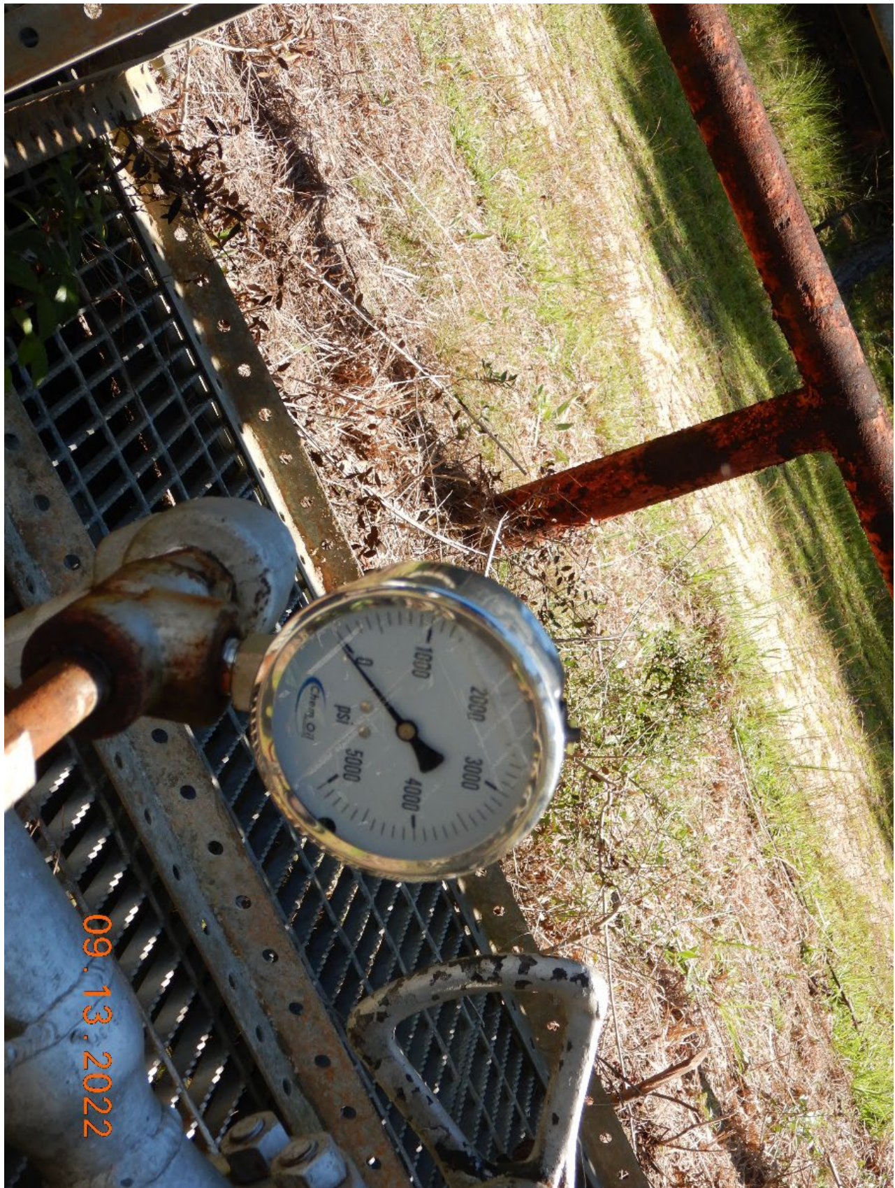
Photograph 4: Looking north, closeup view of production casing pressure gauge reading 0 psi.
