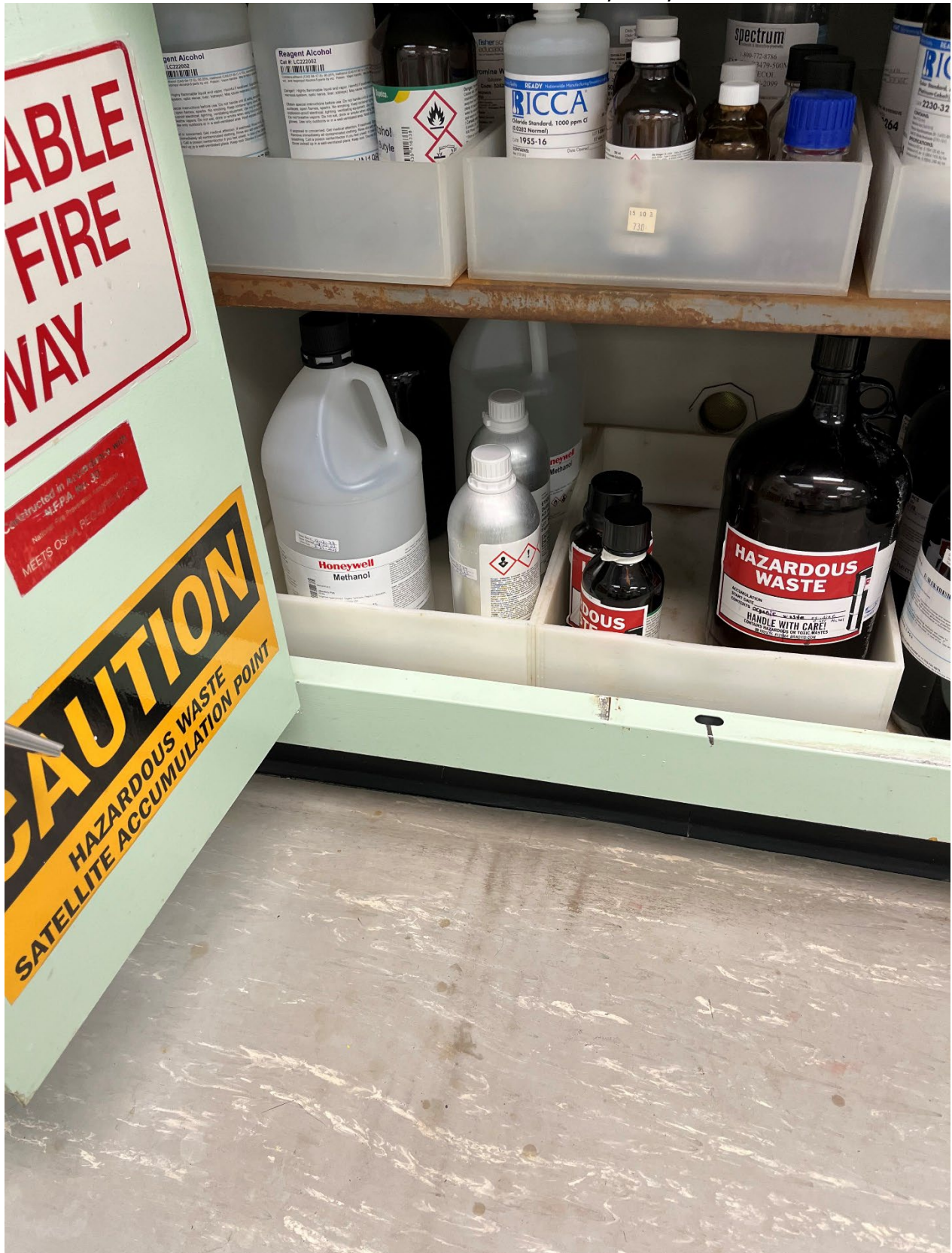
Photo #1: View of a satellite accumulation area in the Quality Analytical Lab.
