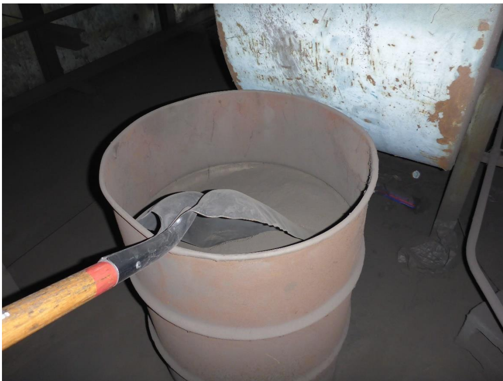
Photo I: 55-gallon drum under Wheelabrator Baghouse. The drum is not closed or labeled.
