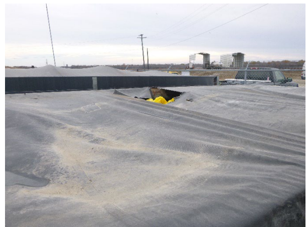
Photograph 5: Non-hazardous 10-day transfer container with ripped tarp.
