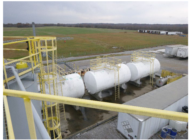
Photograph 43: Non-hazardous tank farm.
