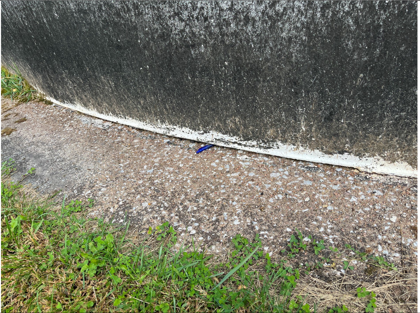
Ground Storage Tank showing missing caulk at base of tank.
