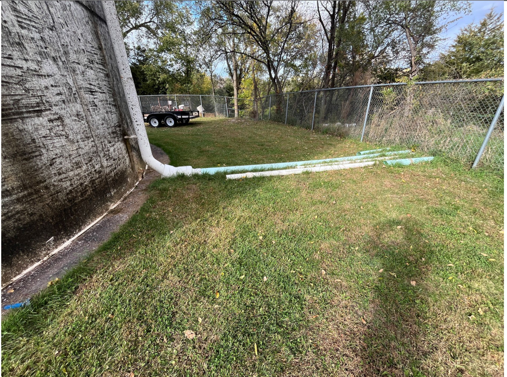
Ground Storage Tank showing overflow discharge pipes.
