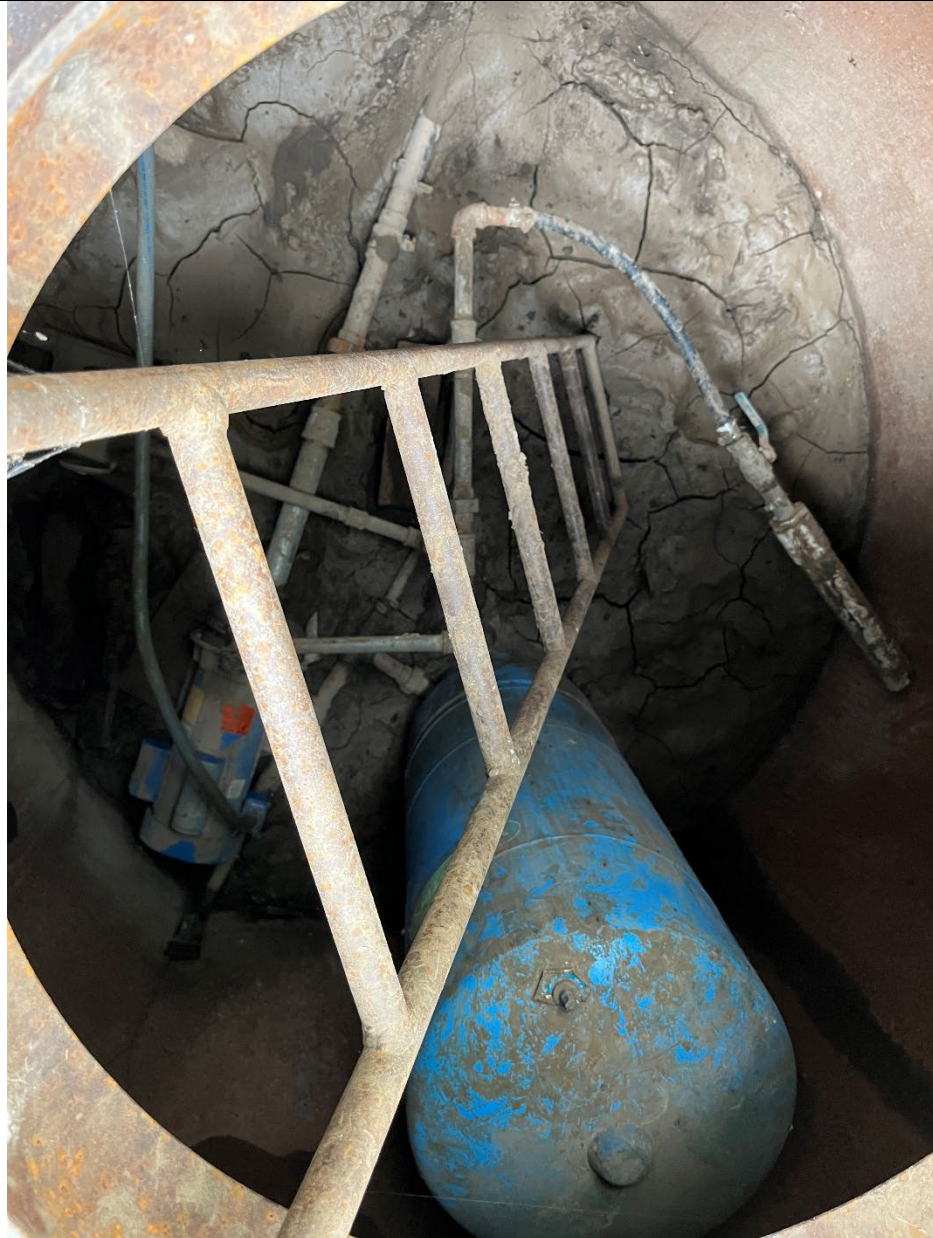
North Commercial Booster Station showing signs of flowing and with connected pressure tank.
