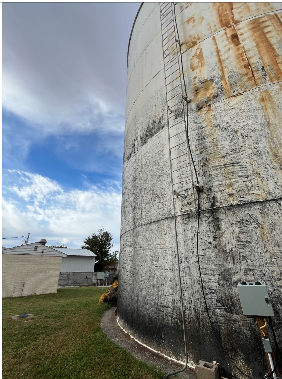
Ground Storage Tank showing no ladder guard at base of ladder.
