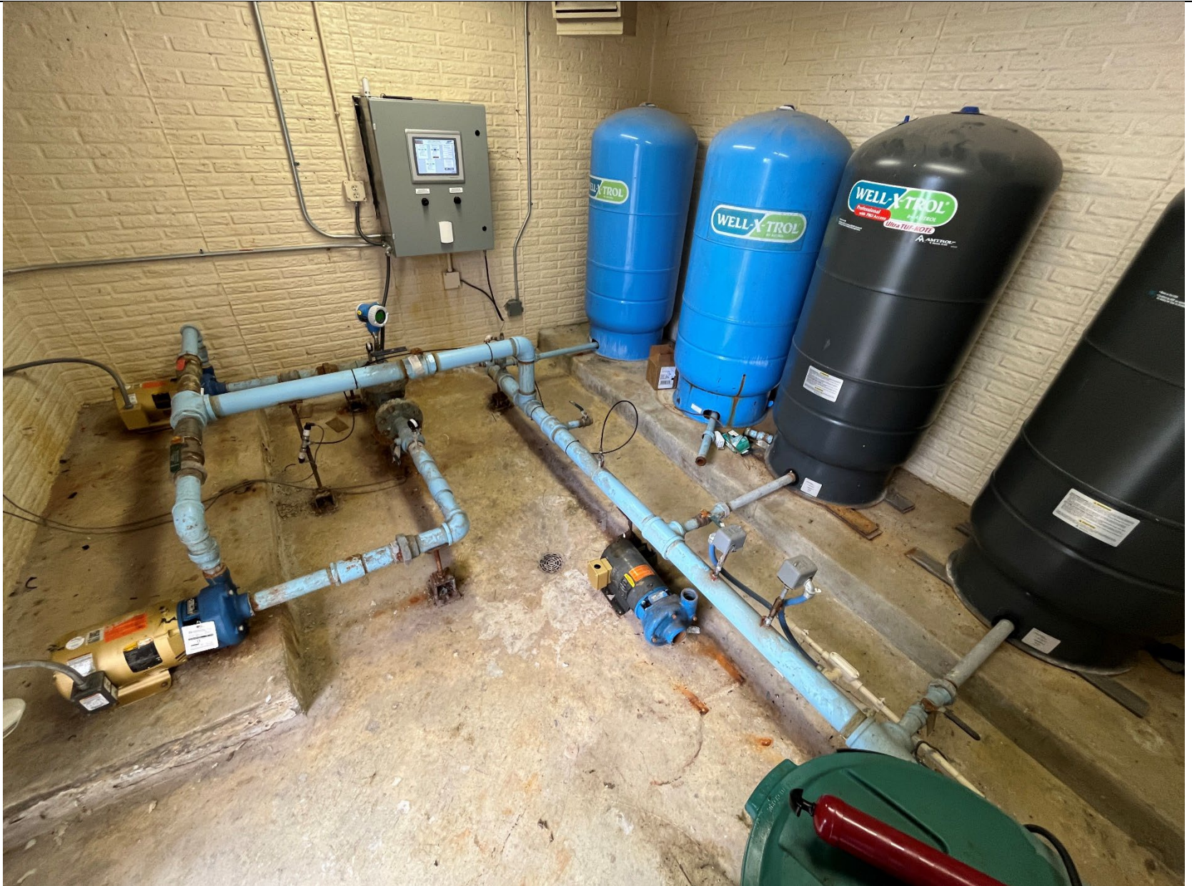
Booster station with connected pressure tank.
