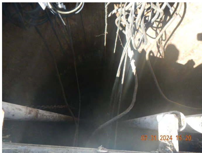
Photo #:17 (DSCN3871) Description: Photo within Lift Station 1.
