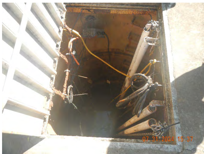
Photo #:19 (DSCN3873) Description: Photo within Lift Station 2.
