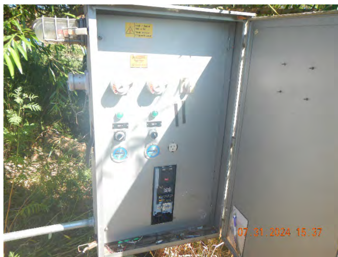
Photo #:20 (DSCN3874) Description: Photo of pump meter display for Lift Station 2.
