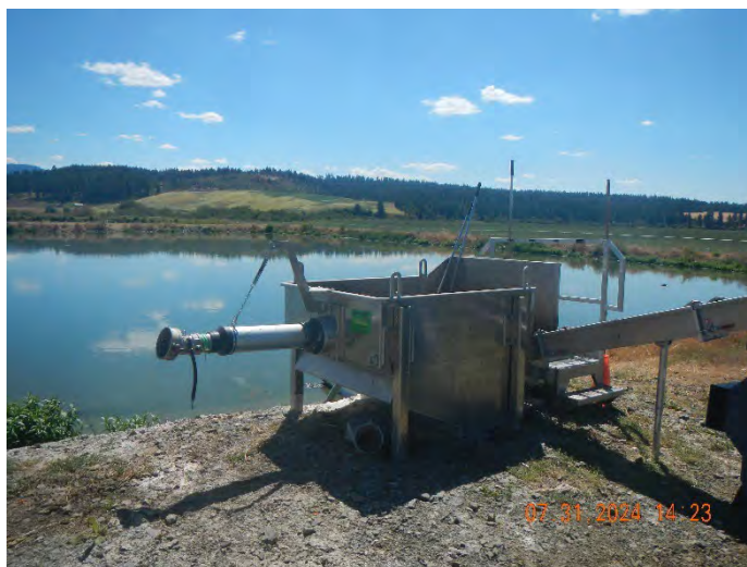
Photo #:02 (DSCN3856) Description: Facing south, photo of septage receiving station along north end of Lagoon 1.
