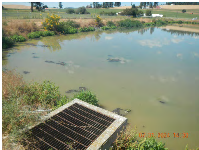
Photo #:03 (DSCN3857) Description: Facing north, photo of lagoon transfer structure along the south side of Lagoon 1.
