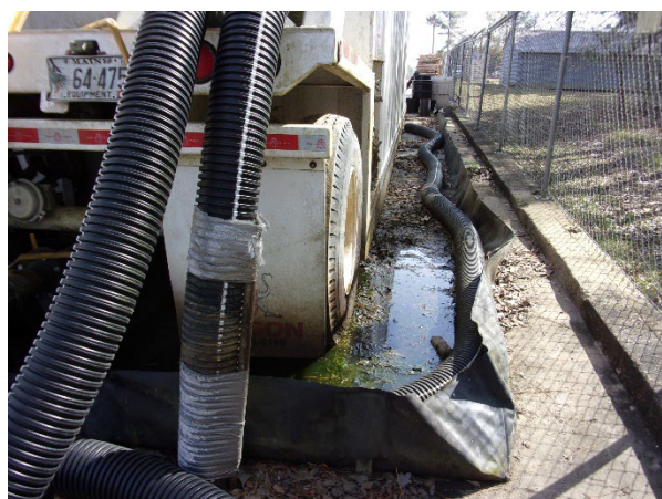
Figure 29: 10:17 AM Non-Hazardous Waste Frac Tank Area
