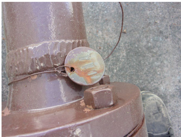
Figure 20: 10:40 AM Tank Farm
