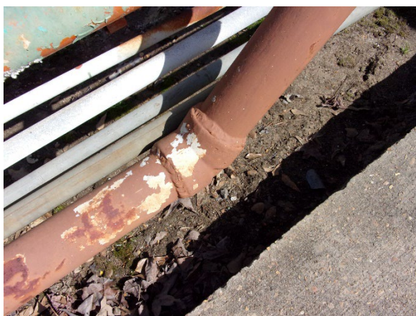
Figure 22: 10:37 AM Tank Farm
