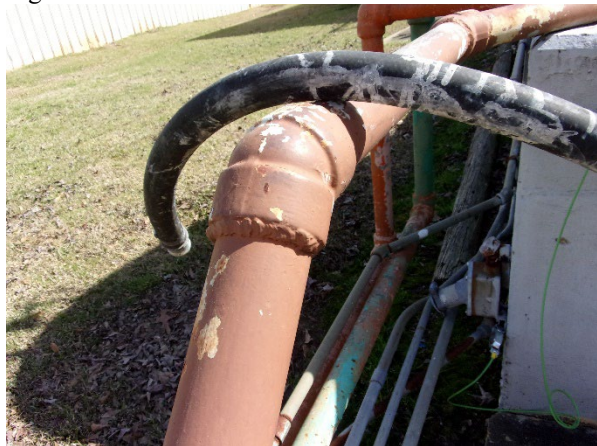
Figure 23: 10:38 AM Tank Farm
