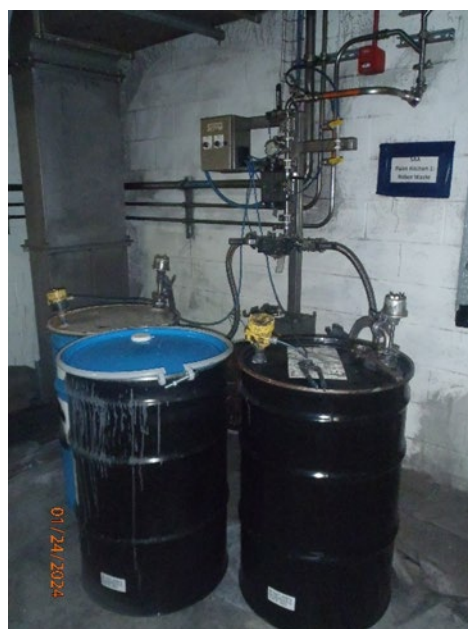
Picture 4 – Paint Kitchen 2 non-hazardous waste drums
