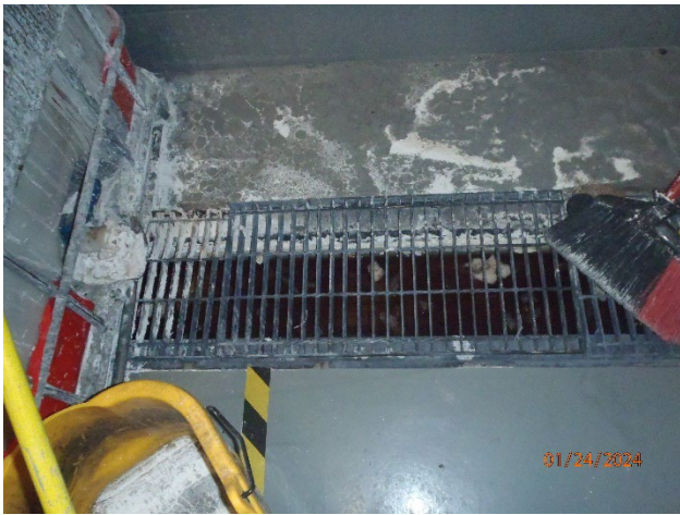
Picture 12 – Electro Clean Storage floor drain grate full
