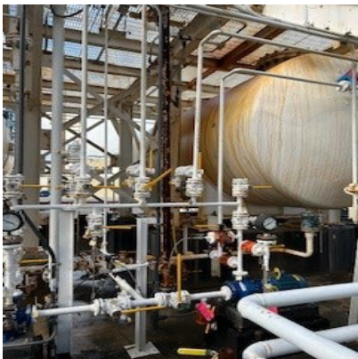
Photo-3 Rust and Signs of Corrosion on the tank's ancillary equipment
