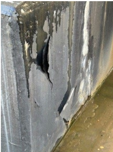
Photo-4 Disrepair saddle on which one of the hazardous waste tank was mounted
