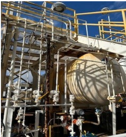
Photo-2 Rust and Signs of Corrosion on Tank's Ancillary Equipment
