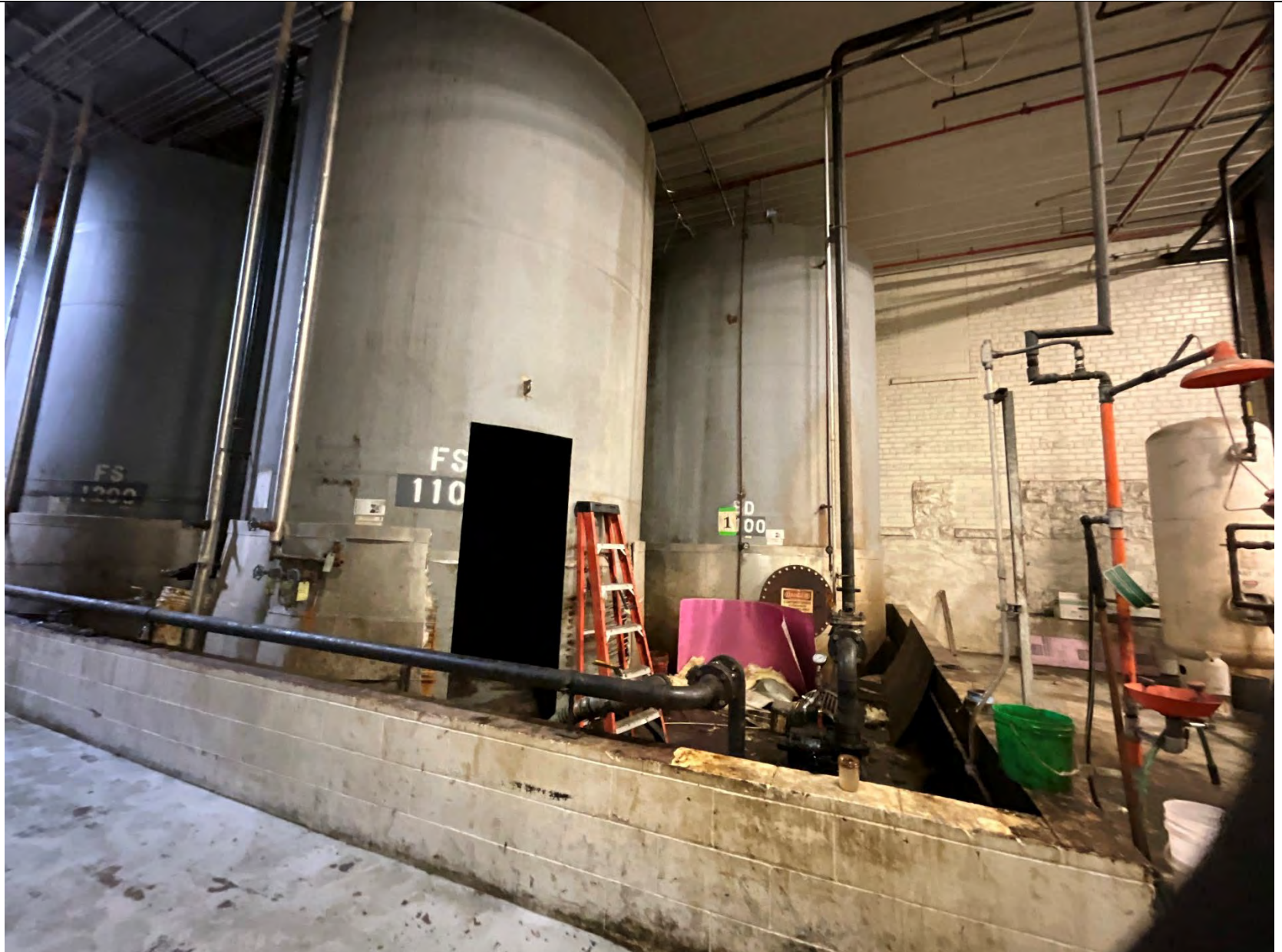
Tank 1 in the background behind Tank 11. All tanks are in a containment area.
