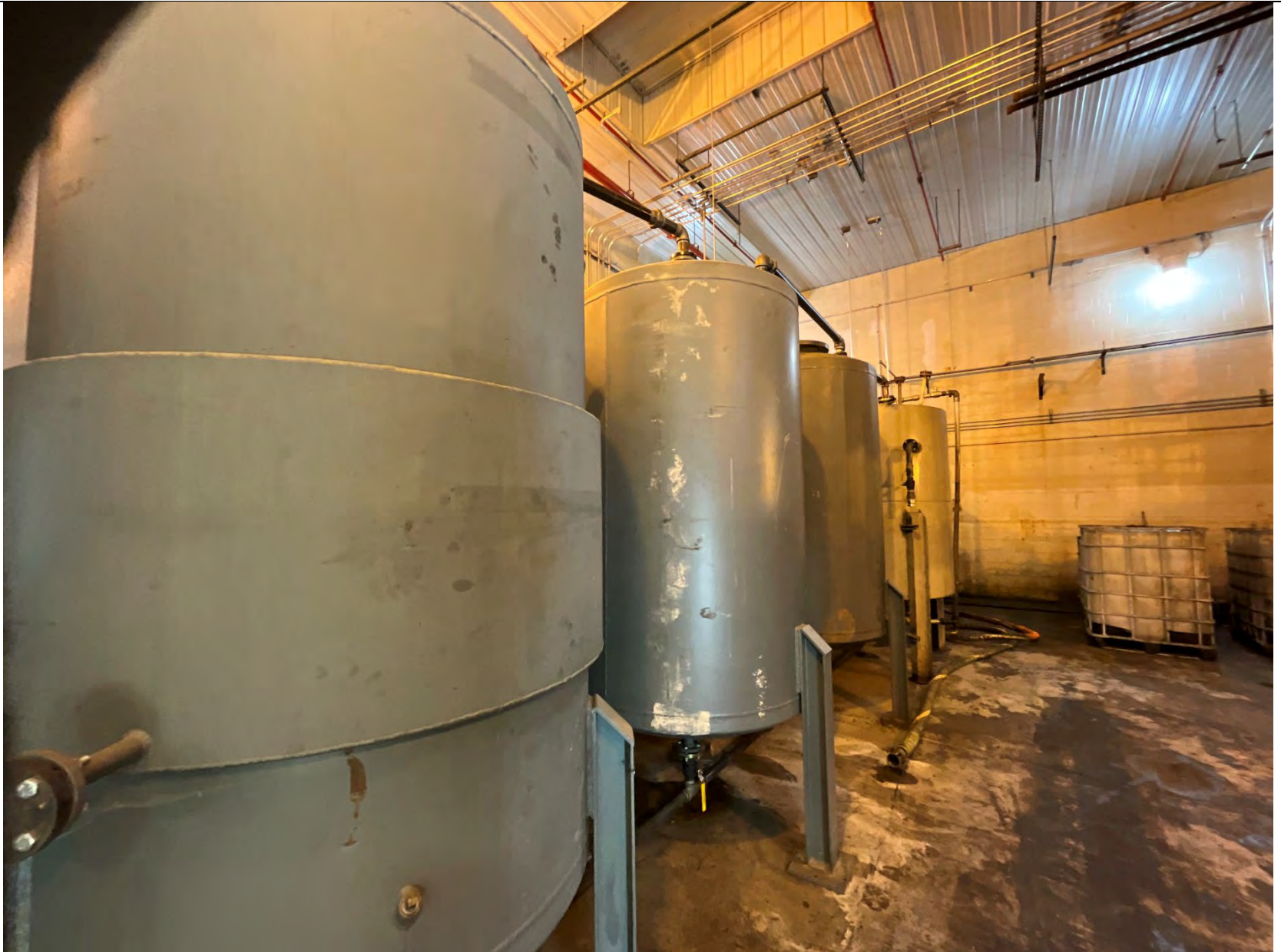
Wet methanol storage tanks.
