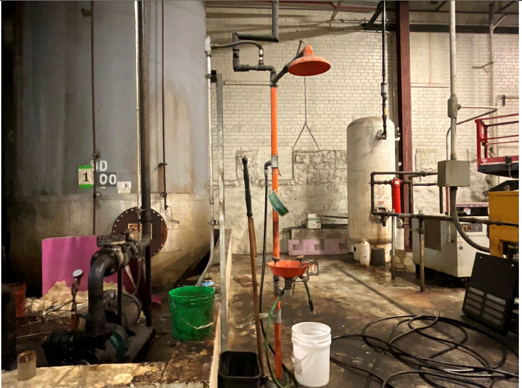
Emergency shower and eyewash station that is functional.
