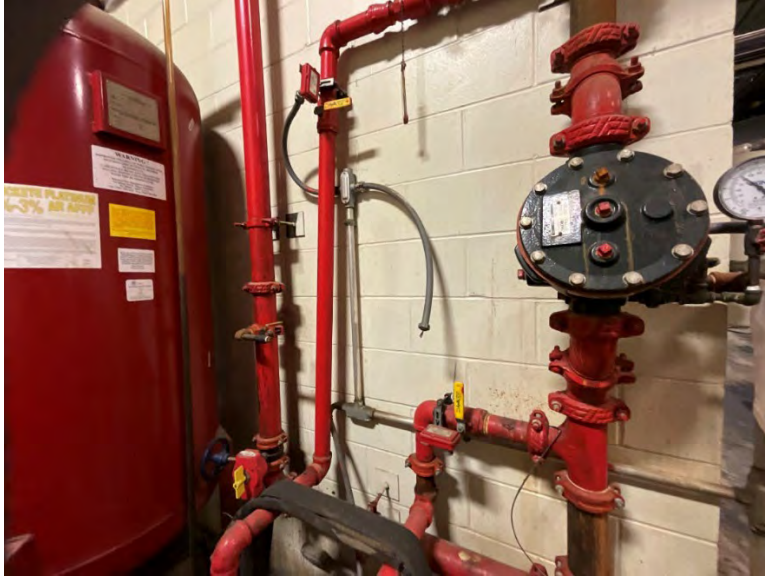
IMG_0497.JPG: Close-up of system – electrical is disconnected and hanging with exposed wires, valves along the water line in closed positions. Water pressure gauge indicates pressure however, part of the system has been disabled and was told that the foam tank is not used.
