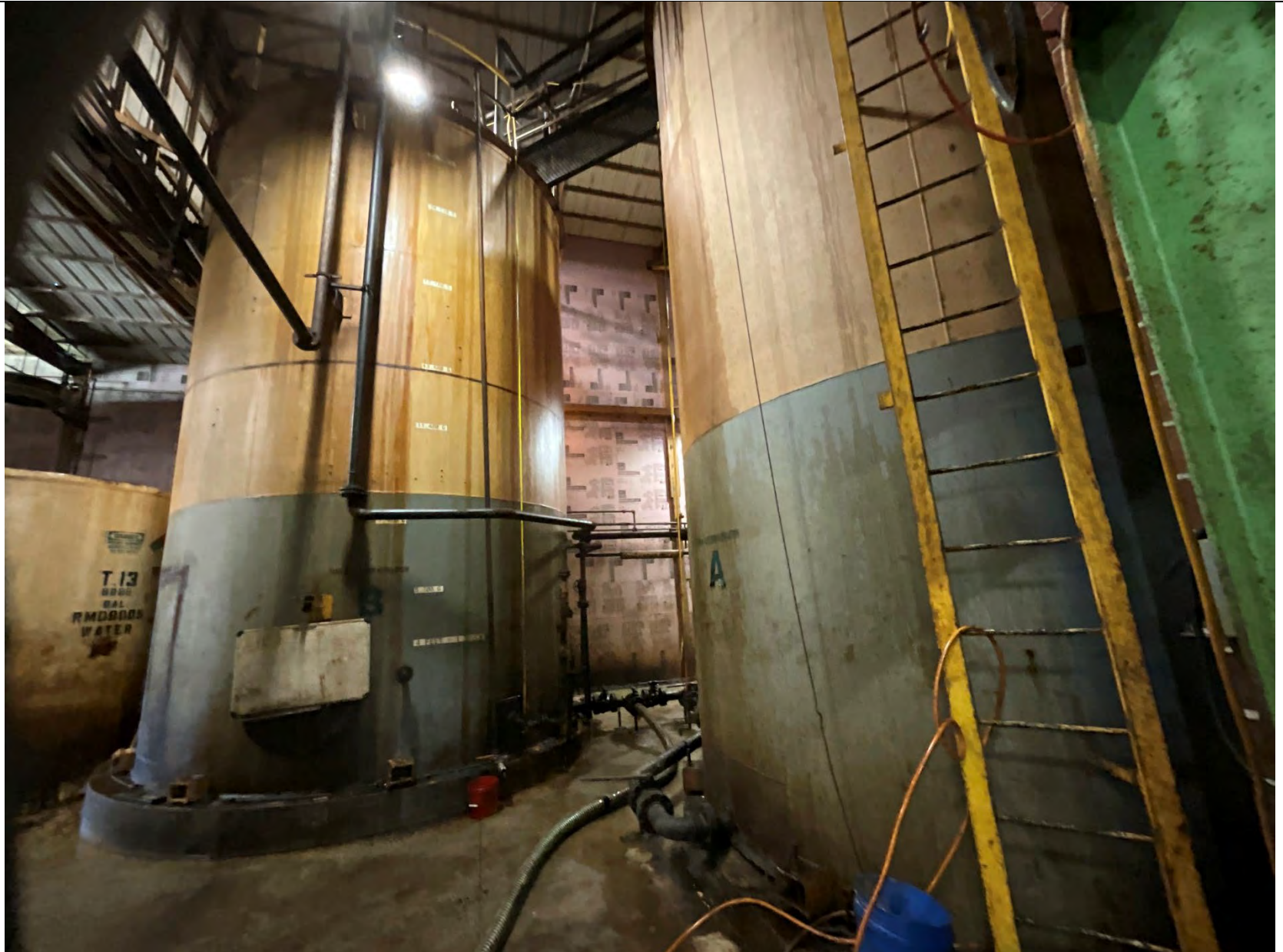
Raw Glycerin tank farm View of Tank A and B. Both are 21,000-gallon capacity.
