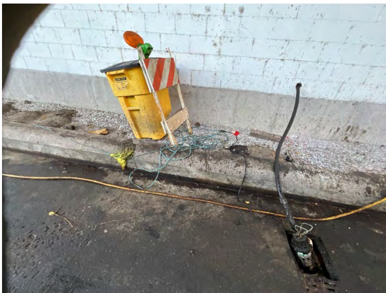
IMG_0515.JPG: Image of sump pump, extension cord, and hose going through a hole in the facility wall to the pit that is located on the other side of the wall.
