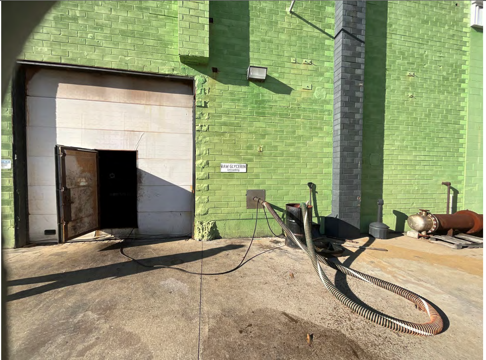
Raw Glycerin unloading truck unloading area. Trucks back in from Exchange Street which is on the south side of the plant complex. Evidence of spills that occur during unloading. East side of the south tank farm and warehouse building.
