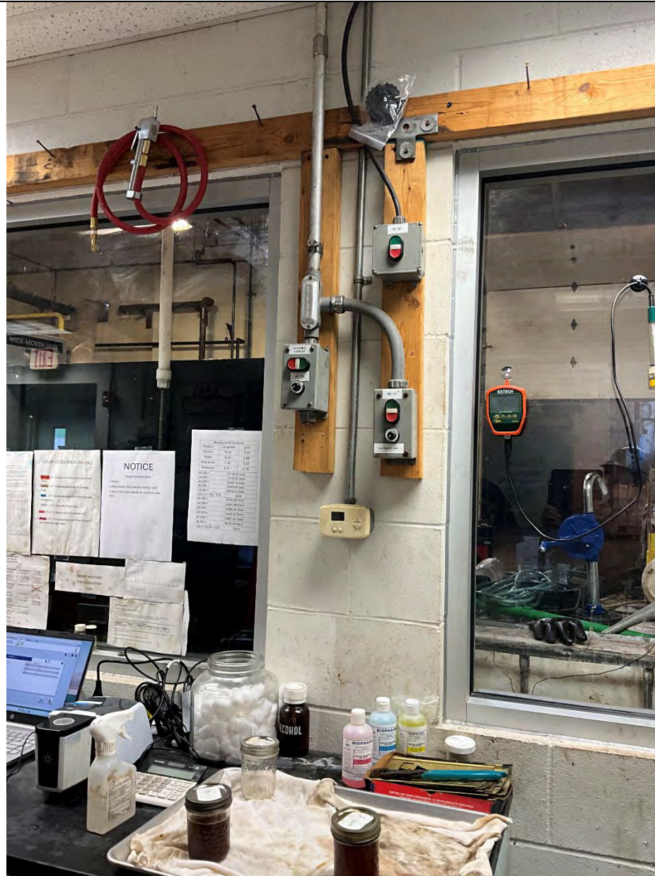
Pump controls include wastewater and methanol loadout.
