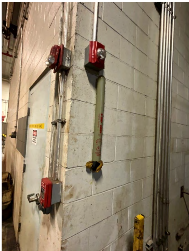
IMG_0493.JPG: Side view of fire alarms in the area around the methanol room. Alarm to the left was said to be functional but appears to be broken.
