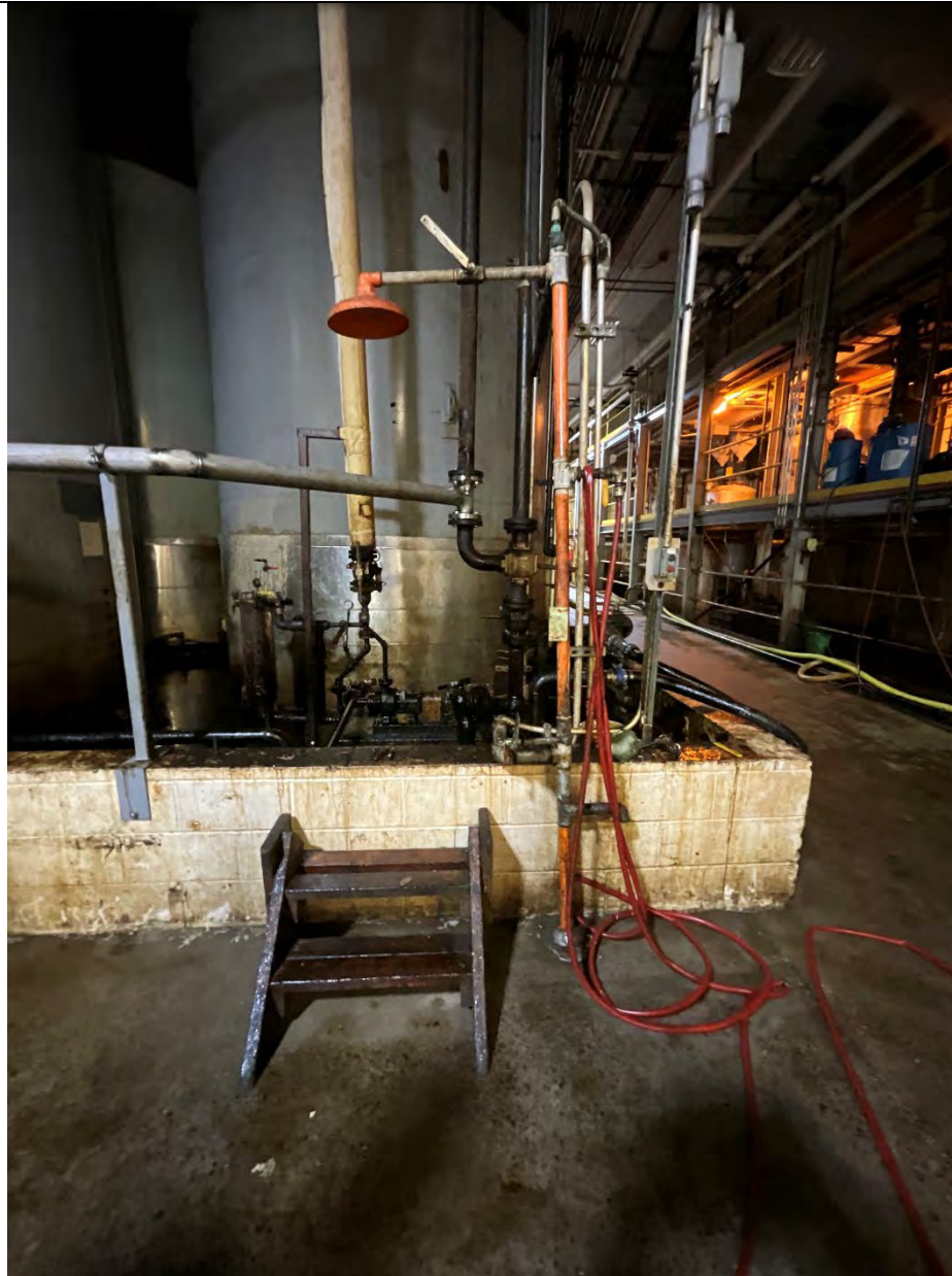
View looking at the front of the tank where the release had occurred.
