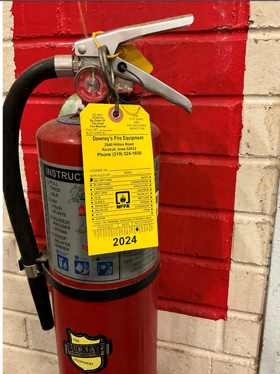
Fire Extinguisher in the Methanol Area.
