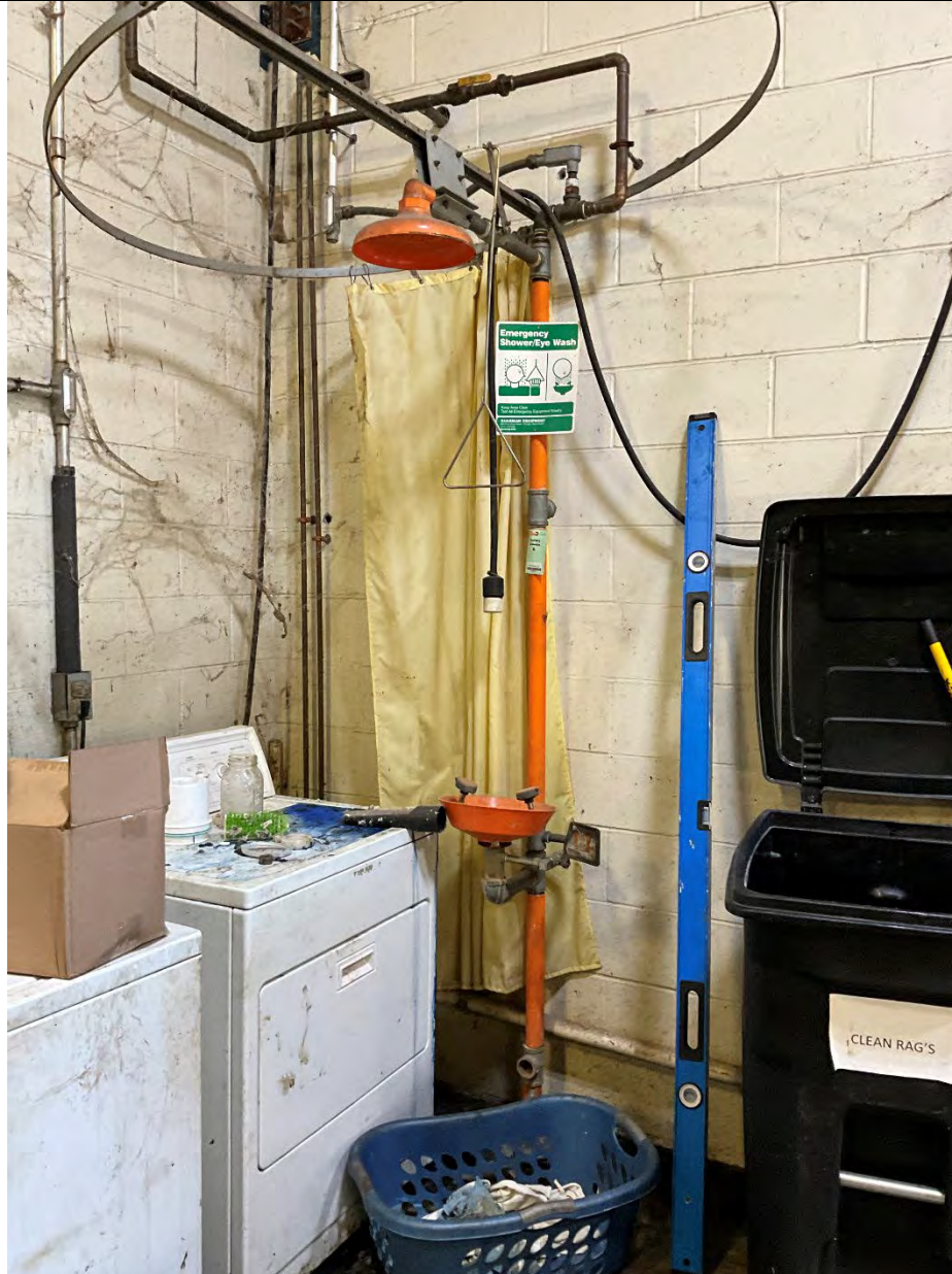
Emergency Eyewash and Shower outside of distillation area.
