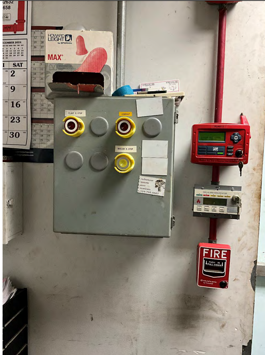
Inside the operations control room. Emergency stops for truck loadout pumps, full plant E-stop and boiler E-stop.
