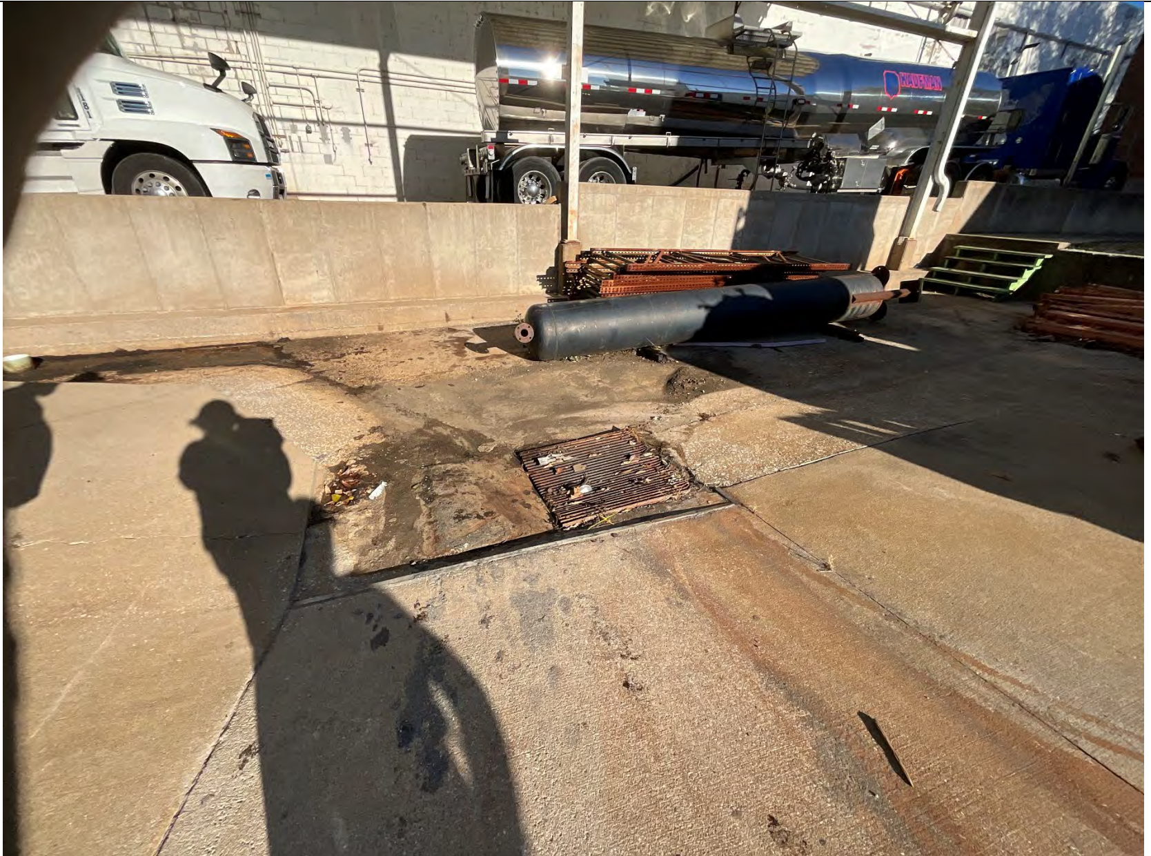
Stormwater Drain – Goes directly to city stormwater system
