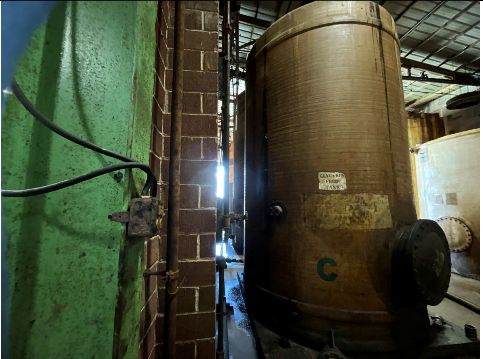
Tank C. Said to contain 5,000 gallons of raw glycerin. And Tank I – 5,500 gallons of raw glycerin, at the very east end.
