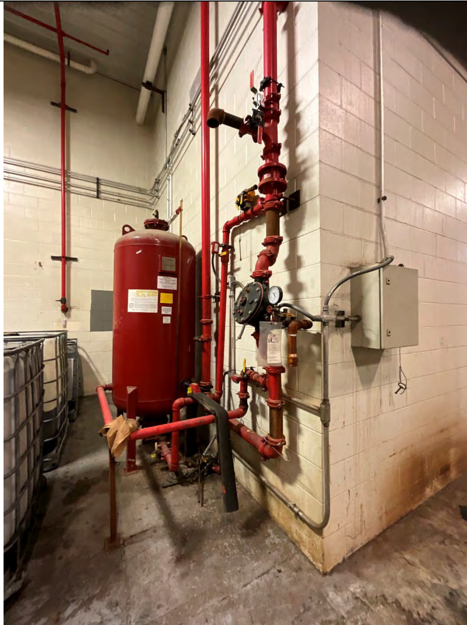
Foam Fire Suppressant System for the methanol tank room and facility.
