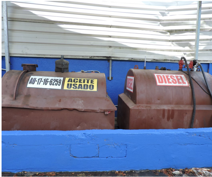
Picture 29 - DCN RECYCLING, CORP. - As observed, the Fuel and Used Oil Storage Area consisted of a metal shed with a ceiling and a secondary containment system and housed two (2) 500-gallon above ground-doble wall tanks to store used oils and diesel clearly labeled.
