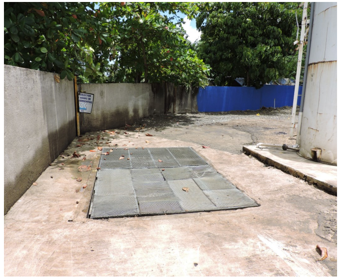
Picture 26 - DCN RECYCLING, CORP. - At the Ferrous Metal Collection Areas, there was one water tower and seep collection sump to control and manage stormwater run-on and run-off of the property. The water tower was out of service and the sump was fully filled with sediments and heavily impacted with used oils.
