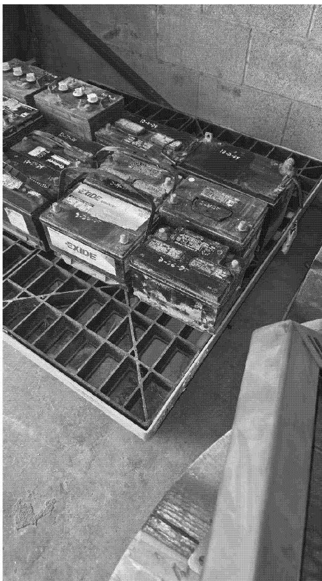
Batteries with Removed Dates
