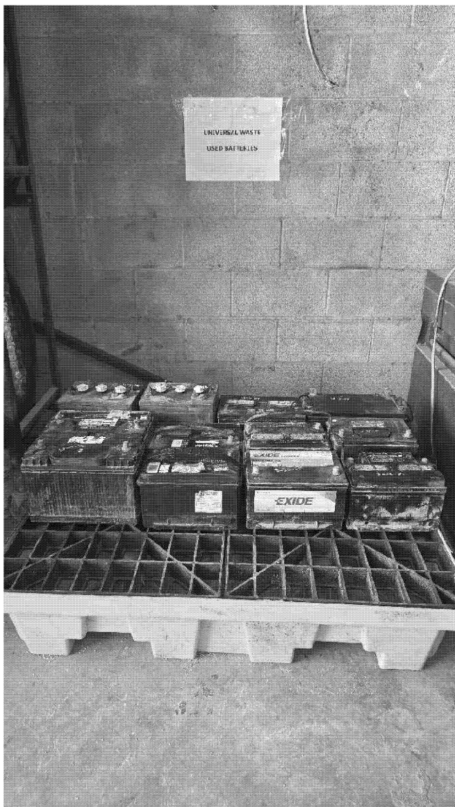
Designated Used Battery Storage Area
