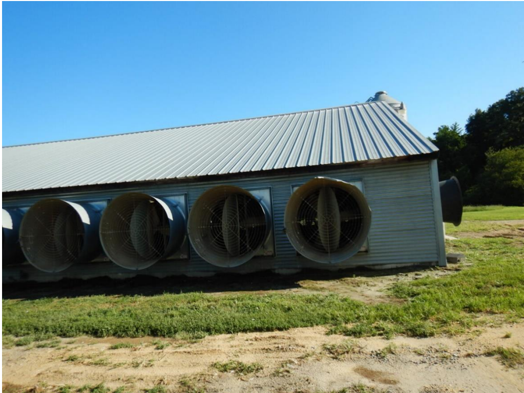
Photograph 13. Exhaust fans on the southeast corner of Poultry Barn 2. Note the feathers on the ground beneath the fans.
