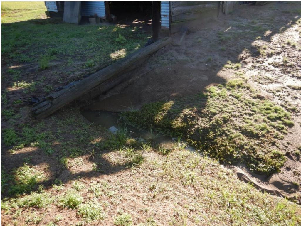
Photograph 6. View of the swale shown in Photographs 4 and 5, near the northern edge of the production area. The swale appeared to continue under the wood framework supporting the sloped building entrance, visible in the upper left part of the photo. The photographer is standing on the west side of the swale.
