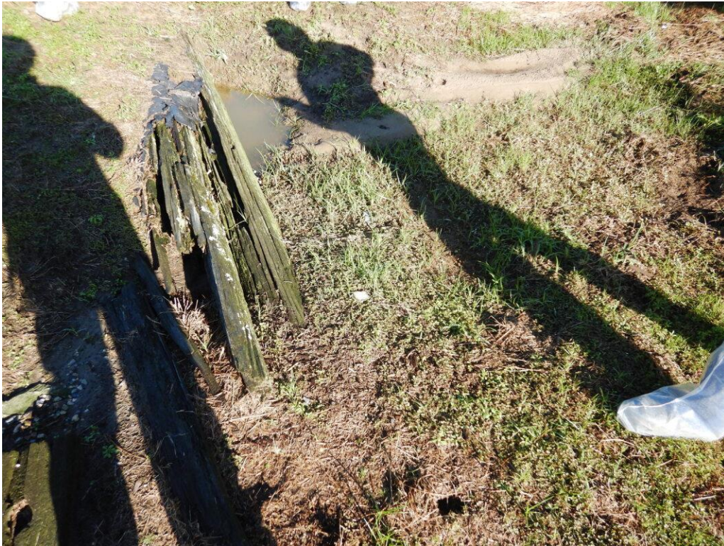
Photograph 7. View of the north side of the sloped building entrance. Note the standing water in the swale and the sediment deposition in the top right portion of the photograph which would appear to indicate flows continue away from the location of standing water, north towards the tree line at the north side of the production area. The photographer is standing on the east side of the swale.
