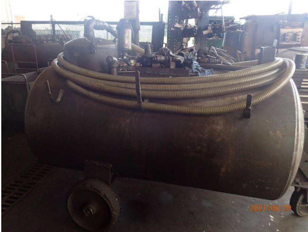
Photo 10: One (1) mobile used oil tank, not labeled “Used Oil”.
