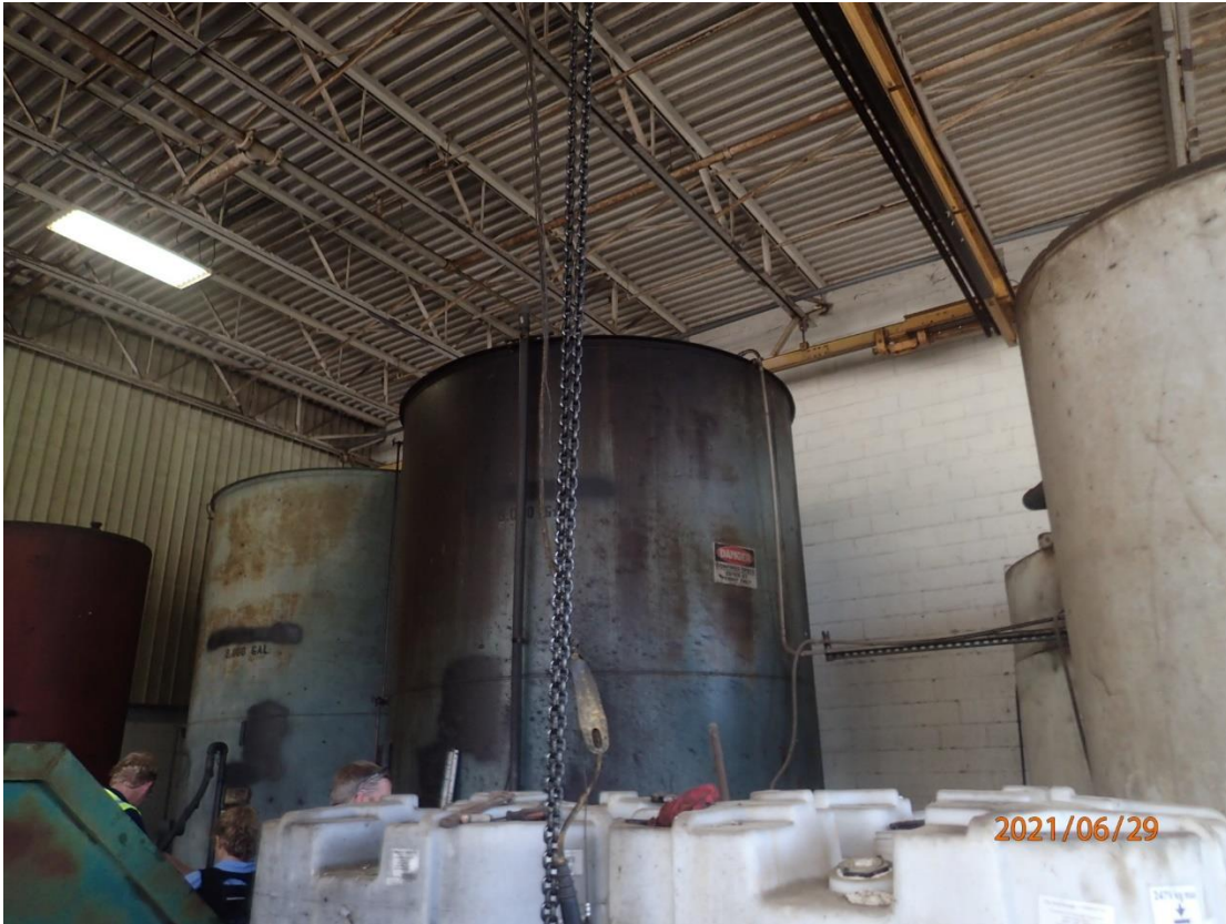
Photo 9: 8,000-gallon above ground storage tanks used to store used oil, not labeled “Used Oil”.
