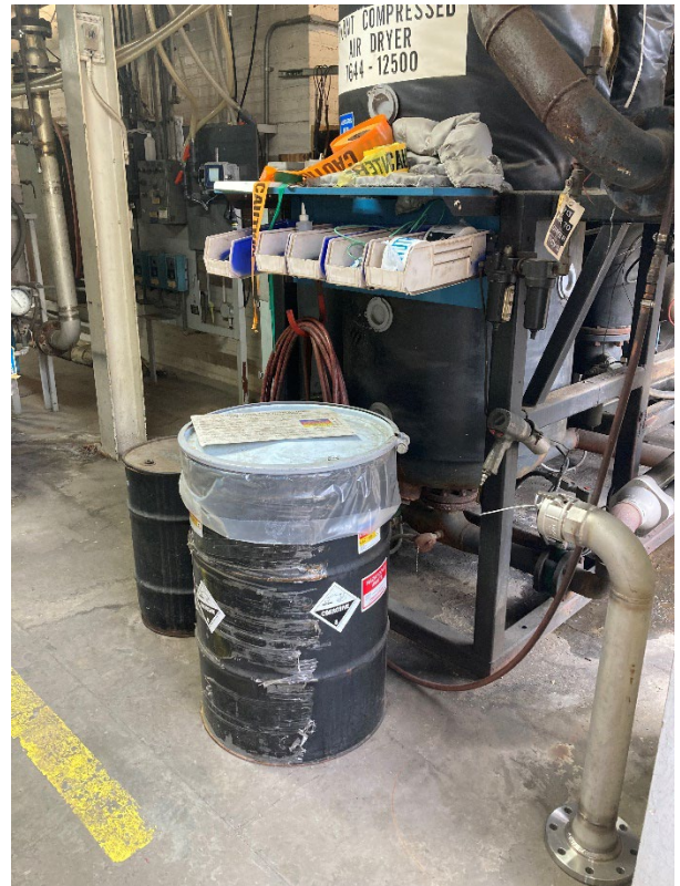
Photograph 19: SAA Scrubber Area.
