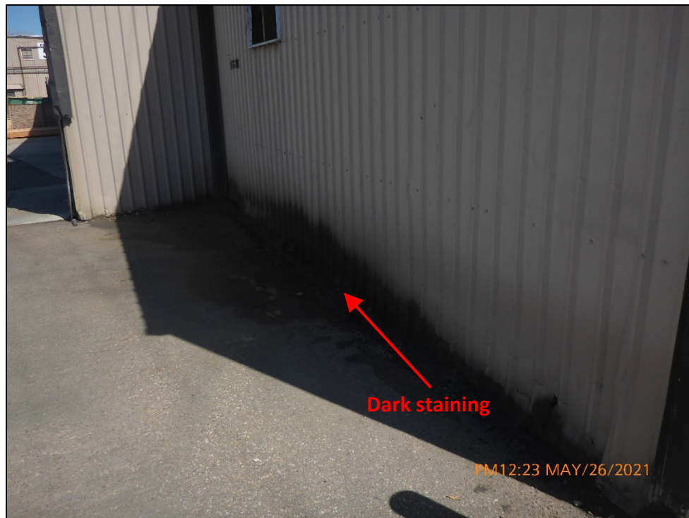
Photograph 24. View of dark residual staining on the pavement surface immediately outside of a warehouse building in the central portion of the northern parcel. Facility representatives stated this staining was from a generator located inside the warehouse building wall.
