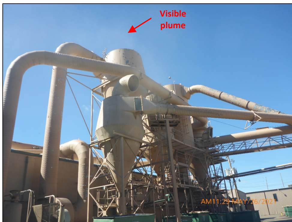
Photograph 20. View of the baghouse shown in Photograph 17, upgradient of the unnamed open pipe stormwater discharge point (shown in Photographs 6 and 7) south of Outfall SW1. Note the visible plume of emissions from the baghouse.
