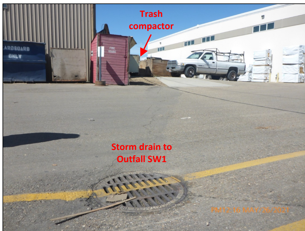
Photograph 5. Additional view of the storm drain located in the central portion of the northern parcel, as shown in Photograph 4. Note the trash compactor located upgradient of this storm drain was not identified on the site map.
