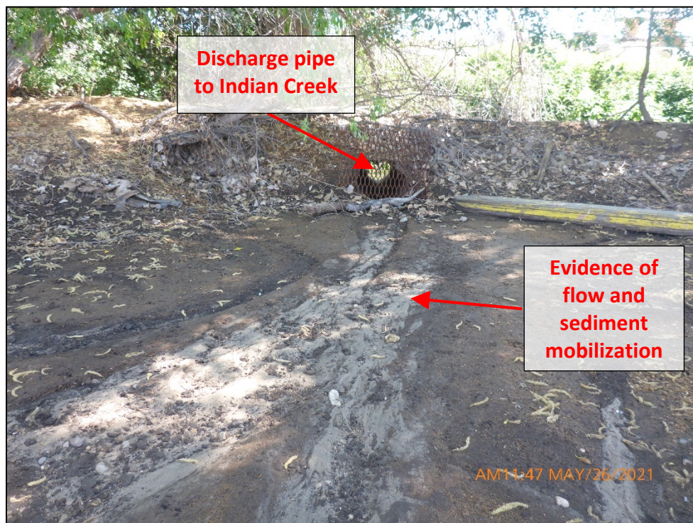
Photograph 8. View of the unnamed open pipe stormwater discharge point north of Outfall SW1. With the exception of a metal screen, no other BMPs were deployed at this discharge point. Note the evidence of flow and sediment mobilization to the outfall.
