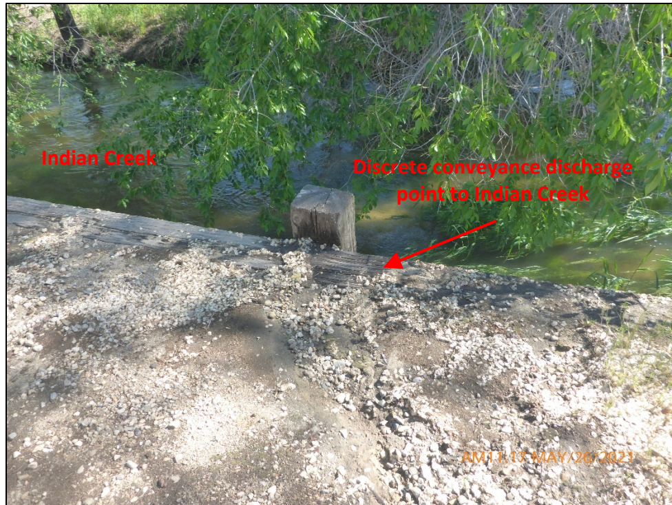
Photograph 13. Close-up view of the discrete overland conveyance discharge point shown in Photograph 12.
