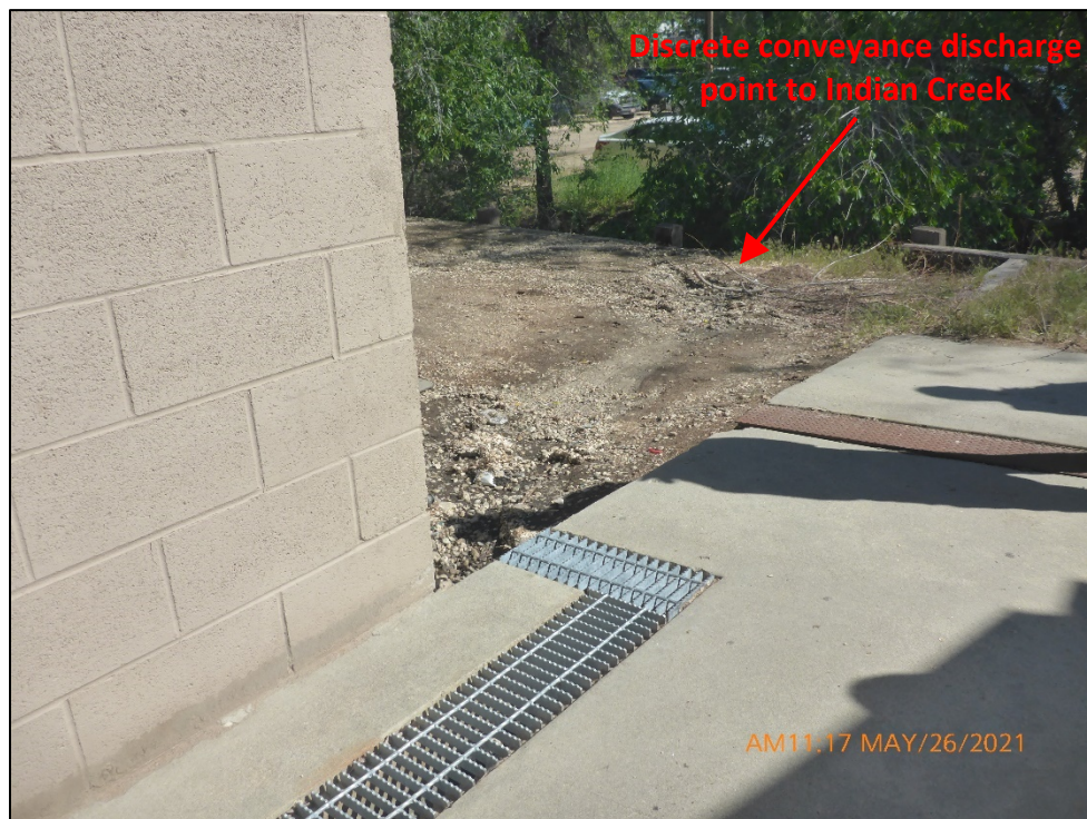
Photograph 12. View of a discrete overland conveyance discharge point to Indian Creek from the southeastern portion of the northern parcel.
