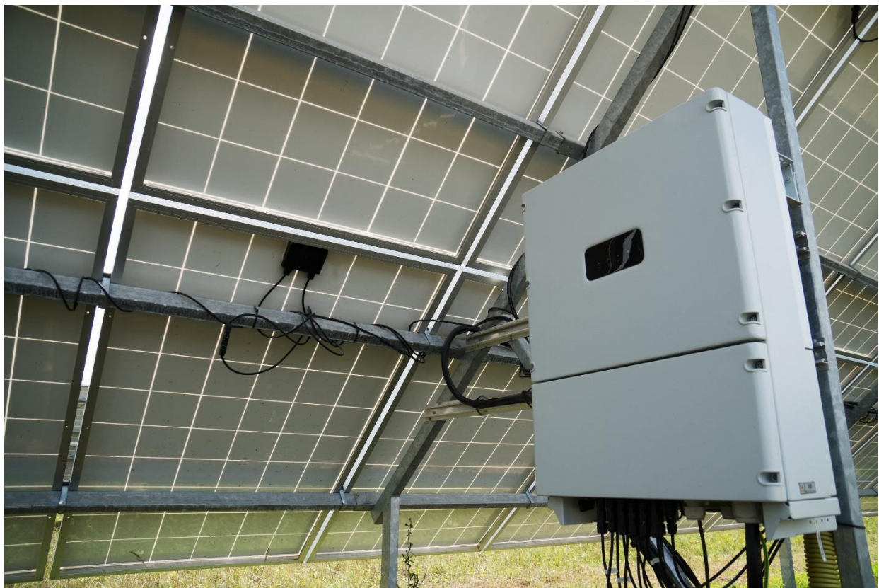
Inverter (Grey Box, Foreground) Behind PV Panels, with Junction Box, Connectors and Wiring
