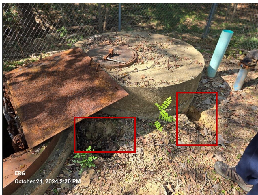
Photograph 3. Library lift station with erosion, outlined in red, by the wet well.
