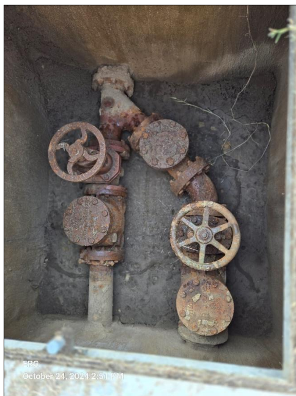
Photograph 12. Trailer Park lift station valve pit.
