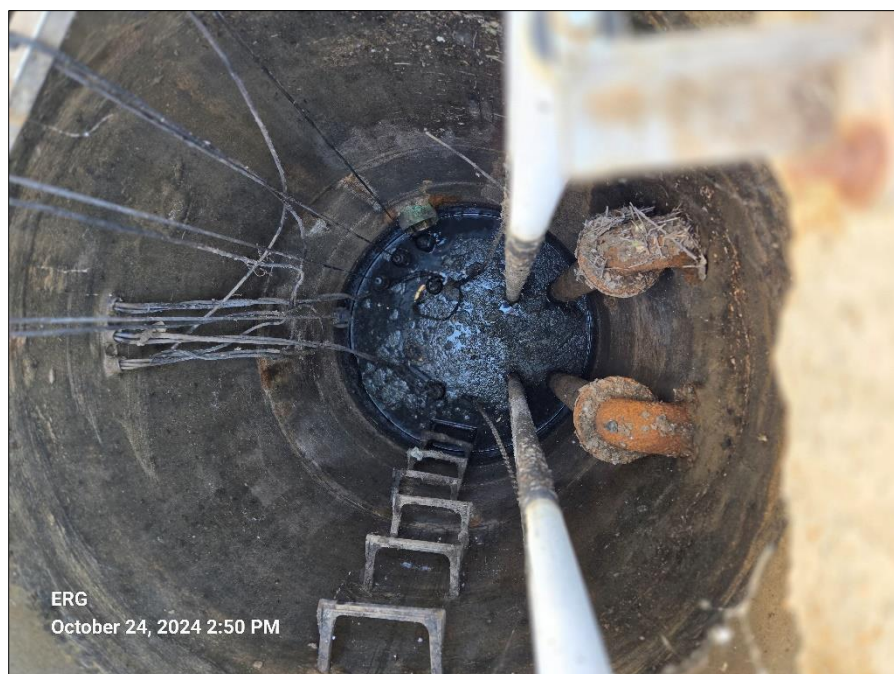
Photograph 11. Trailer Park lift station wet well.
