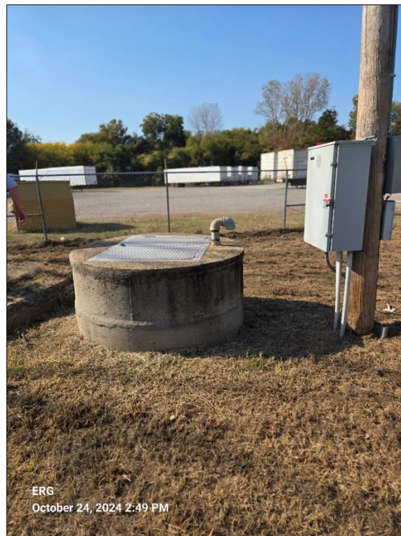
Photograph 10. Trailer Park lift station.
