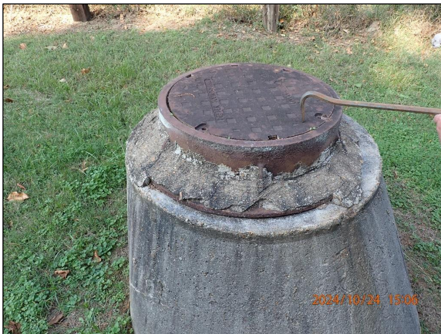
Photograph 17. Exterior of the Railroad manhole. Note the gaps/cracks in the grout and concrete exterior of the manhole.
