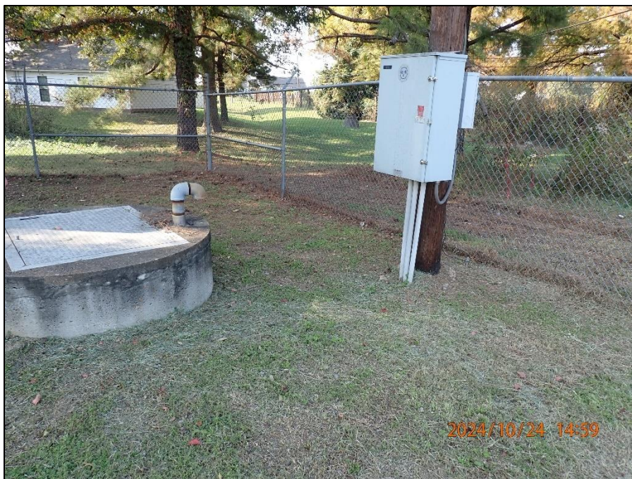
Photograph 13. Railroad lift station.
