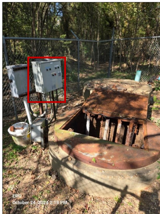
Photograph 2. Library lift station. The pump control panel is outlined in red. Note the rust and corrosion on the wet well access.
