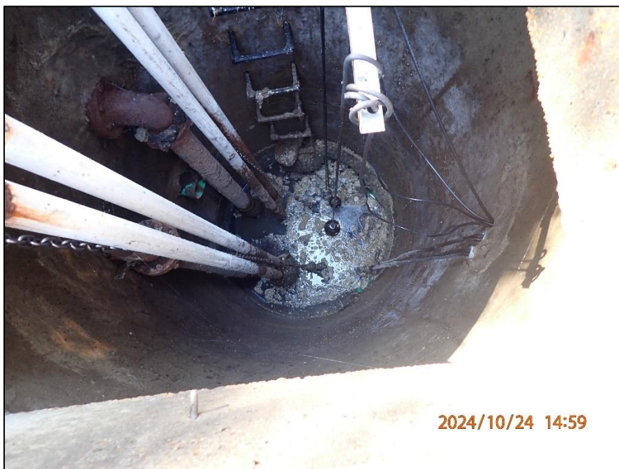
Photograph 14. Railroad lift station wet well. Note the grease accumulation in the wet well.
