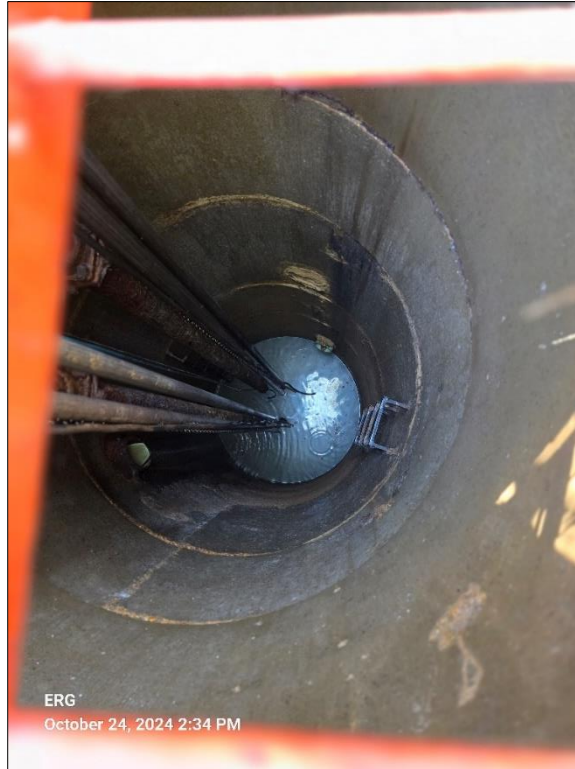
Photograph 7. Morningside lift station wet well.
