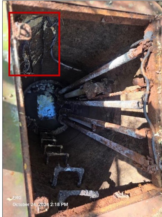
Photograph 1. Library lift station wet well. Note the rust and corrosion on the interior of the wet well and the float gauges. Also note evidence of high-water levels in the wet well, outlined in red.
