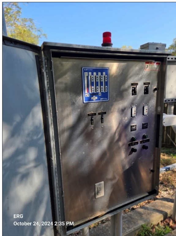
Photograph 8. Morningside lift station pump control panel.
