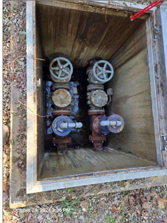
Photograph 9. Morningside lift station valve pit at the.
