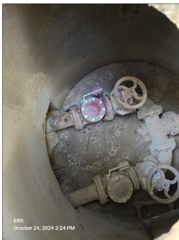
Photograph 4. Library lift station valve pit. Note evidence of flooding.
