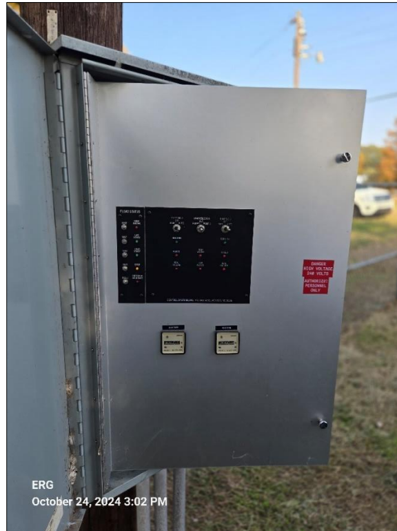
Photograph 15. Railroad lift station pump control panel.
