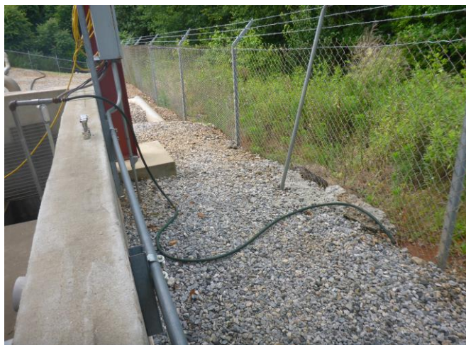
Photo 4 – Hazardous Waste Tank: Garden hose leading from the small sump in the secondary containment area of the hazardous waste tank to a nearby ditch.
