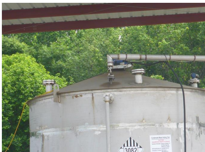
Photo 10 – Hazardous Waste Tank: Pipe on top of the tank is ancillary equipment used to transfer landfill gas condensate to the 6,000-gallon hazardous waste tank. The tank is open to the atmosphere through the overflow pipe down the front of the tank, through a port on the top of the tank used to measure the thickness of the oily liquid waste, and through a port on the top of the tank through which the floating level indicator line passes.
