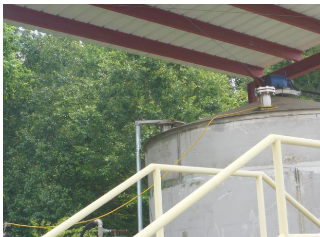
Photo 9 – Hazardous Waste Tank: Pipe on top of the tank is ancillary equipment used to transfer landfill gas condensate to the 6,000-gallon hazardous waste tank. The tank is open to the atmosphere through the port on the top of the tank through which the floating level indicator line passes.
