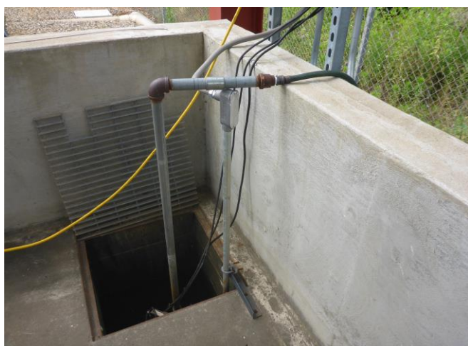
Photo 3 – Hazardous Waste Tank: Small sump in the secondary containment area of the hazardous waste tank.
