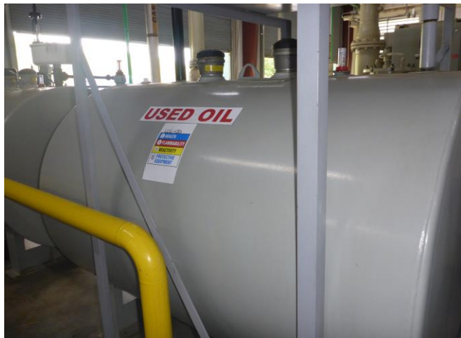
Photo 1 – Compressor Room: 600-gallon double walled tank for accumulating used oil from general maintenance activities.
