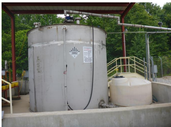
Photo 2 – Hazardous Waste Tank: 6000-gallon tank used to accumulate landfill gas condensate (D004, D027) and oily liquid waste (D001, D009, D027).
