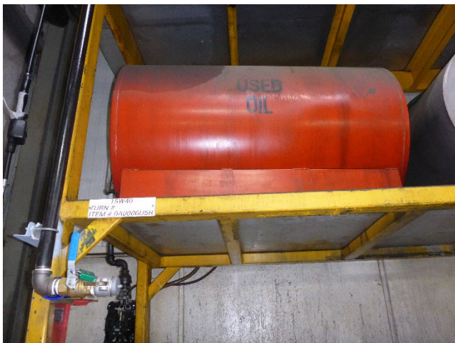
Photo 16: Red used oil tank on elevated shelf in the GSE Shop.
