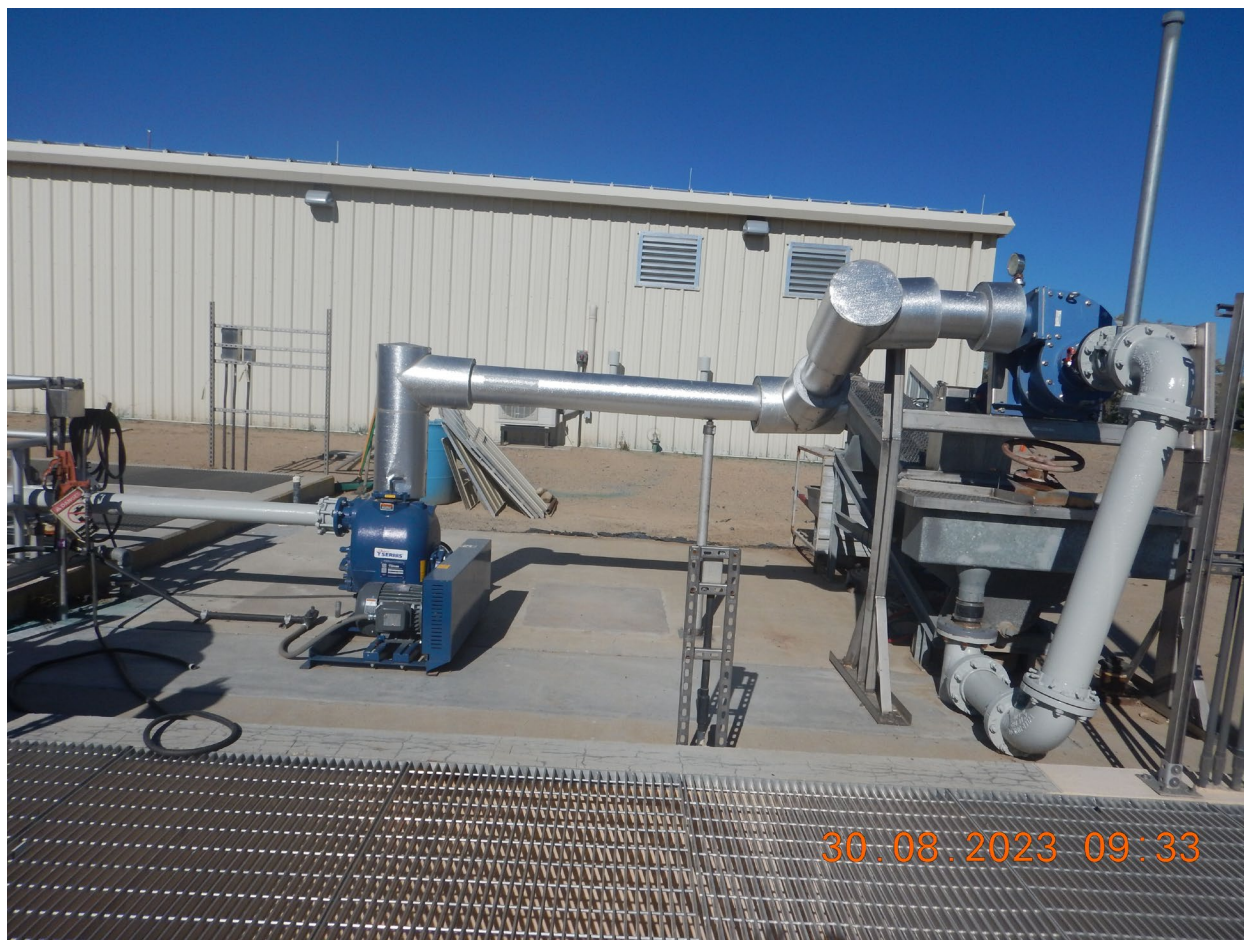
View new headworks at the WWTP. (DSCN2636). Photographed by D. Esparza
