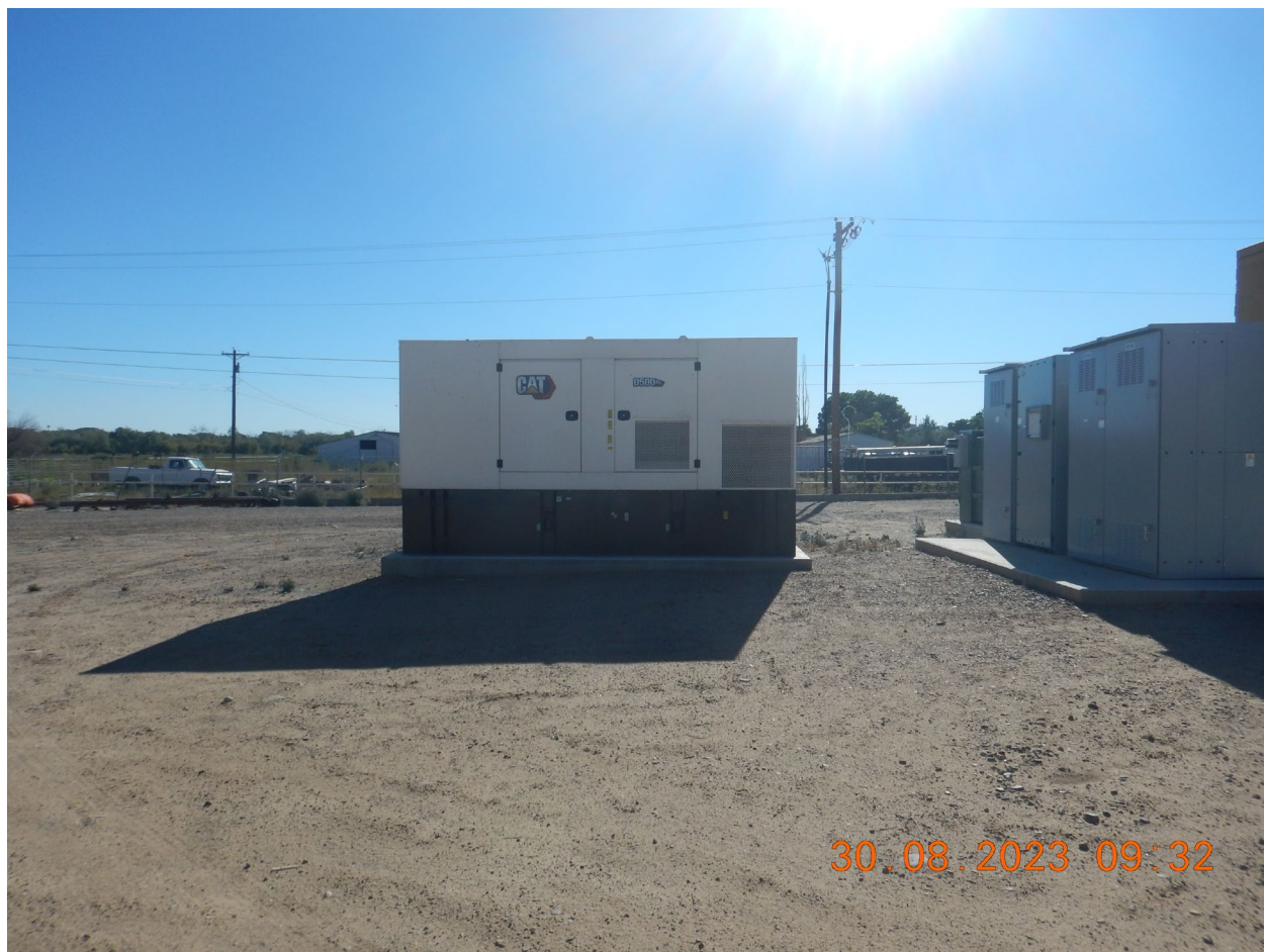
View of new WWTP back-up power generator. (DSCN2635). Photographed by D. Esparza
