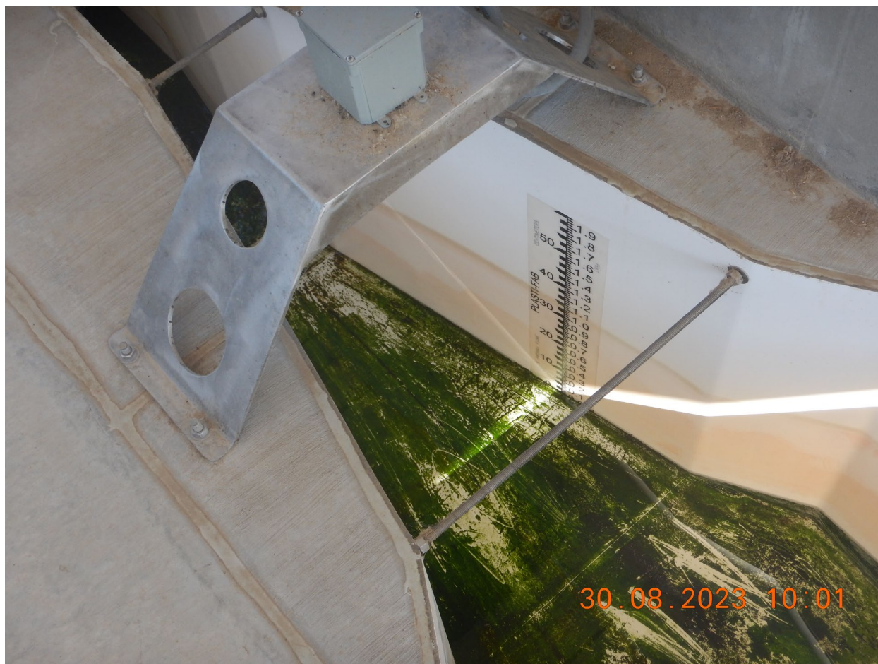
View of the new Parshall flume and the top side ultrasonic sensor. (DSCN2643). Photographed by D. Esparza
