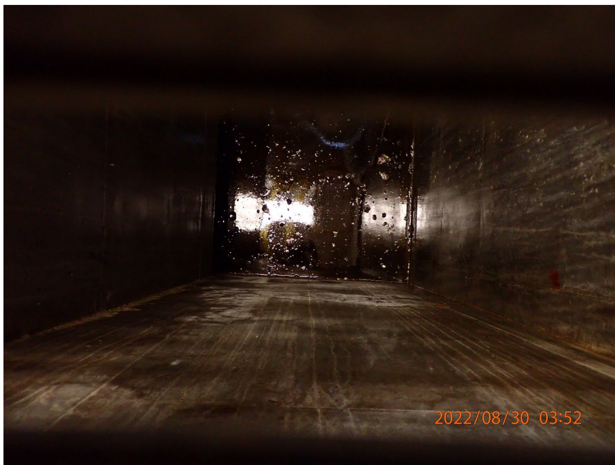
Photo 4 - Chlorine contact chamber
