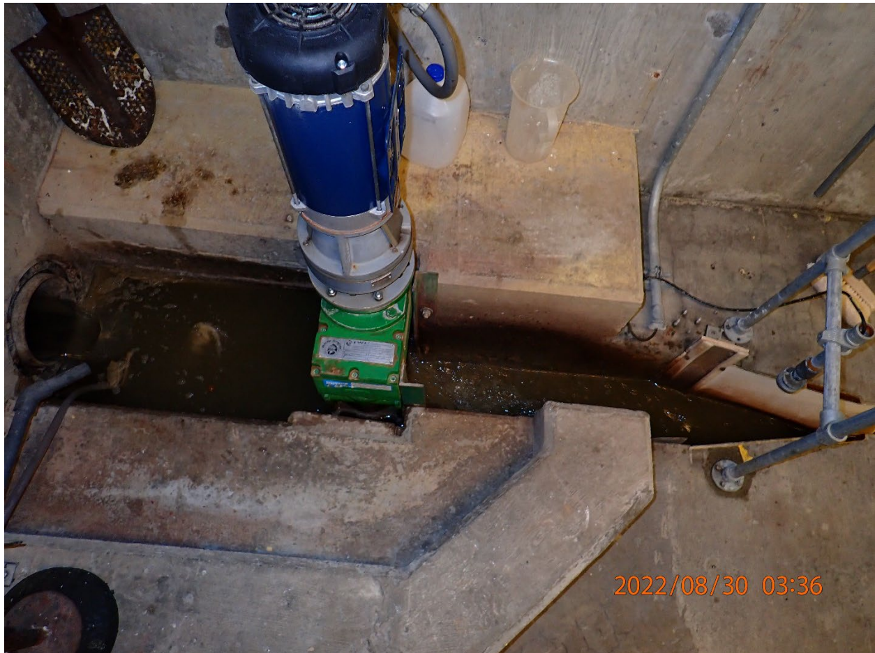
Photo 1 - Flow meter and flume
