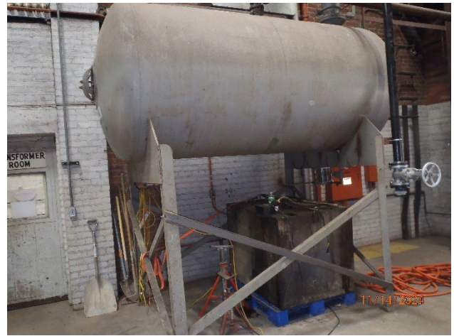
Picture 39 – Shop 2 Compressor Room condensate collection box
