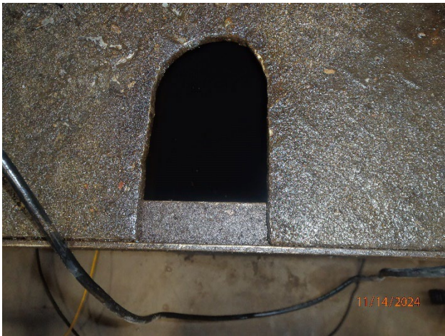
Picture 37 – Shop 2 Compressor Room condensate collection box oily water
