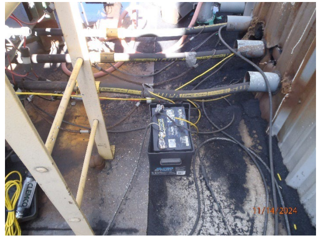
Picture 45 – Shop 2 Blaster Shop lead acid battery in water
