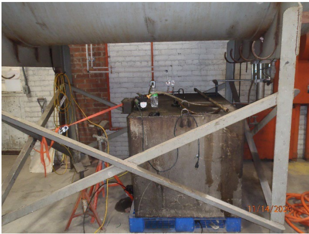
Picture 36 – Shop 2 Compressor Room condensate collection box
