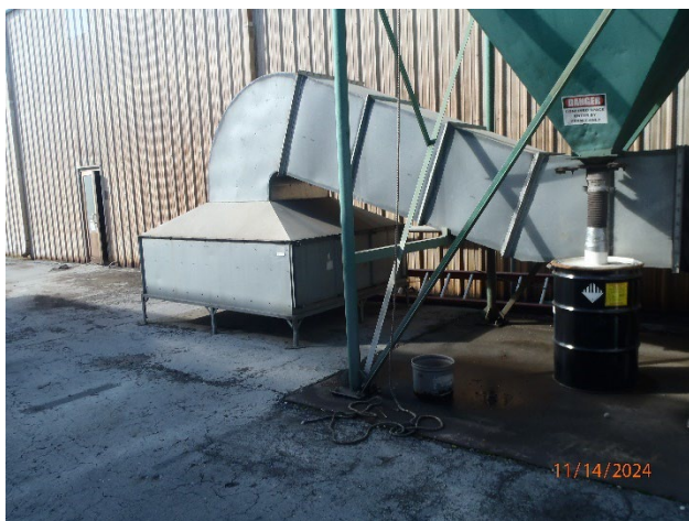
Picture 12 – Blast Media Booth CLEMCO dust collection system
