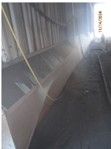
Picture 49 – Shop 2 Blaster Shop spent media from lead abatement
