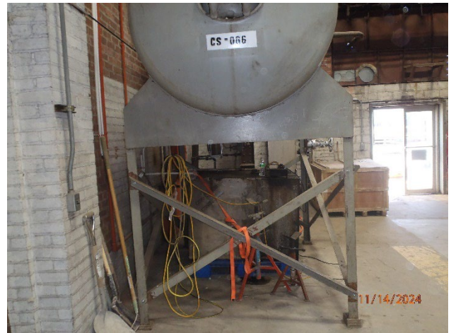
Picture 40 – Shop 2 Compressor Room condensate collection box
