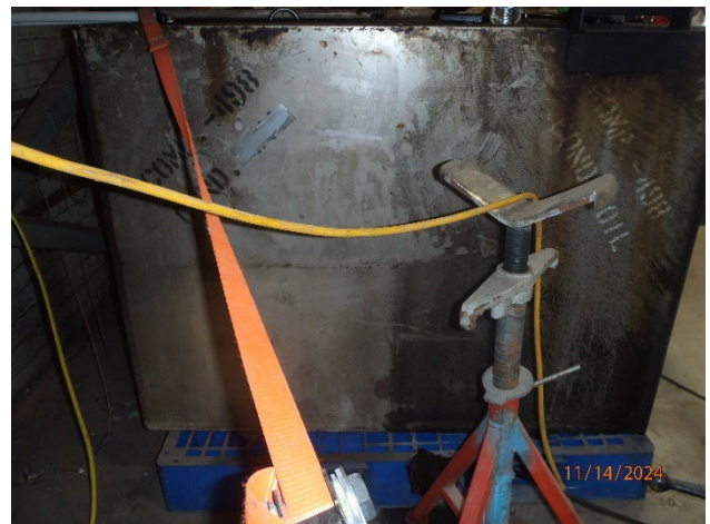
Picture 41 – Shop 2 Compressor Room condensate collection box
