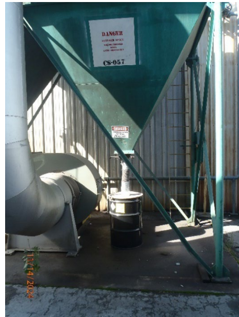
Picture 8 – Blast Media Booth CLEMCO baghouse
