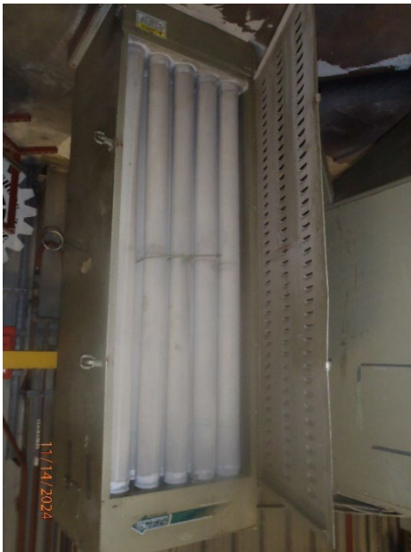
Picture 30 – Breaker Shop Zero Blast Cabinet filters
