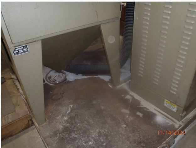
Picture 27 – Breaker Shop Zero Blast Cabinet spilled media
