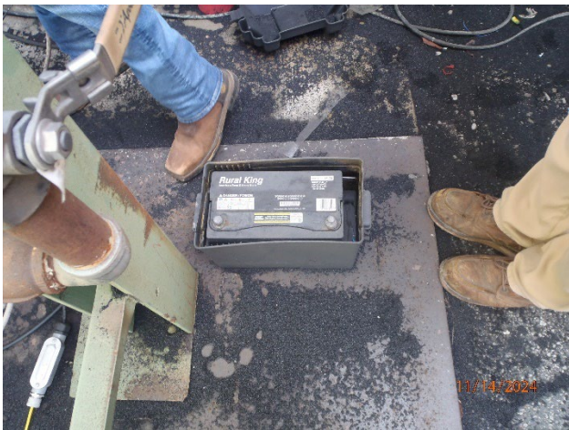
Picture 44 – Shop 2 Blaster Shop lead acid battery in water
