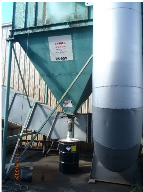
Picture 10 – Blast Media Booth CLEMCO baghouse
