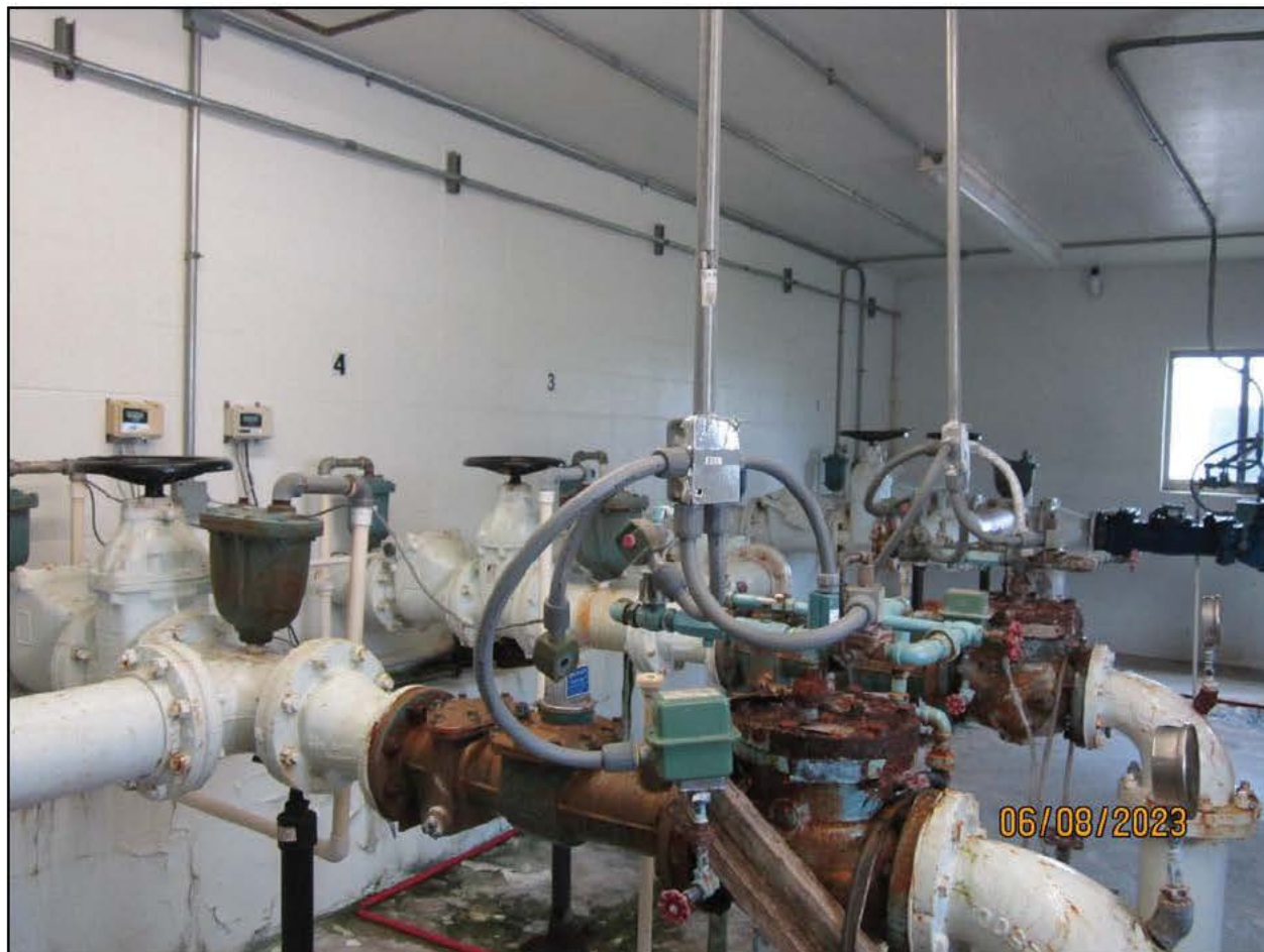
Photograph 19. Water Treatment Plant, Clear Well Pump Valve House View of the piping supporting the pumps delivery of finished water to the distribution system. One of the lines appeared to be supported by a wooden brace and a few assets had components that had lost their coatings and were rusting.
