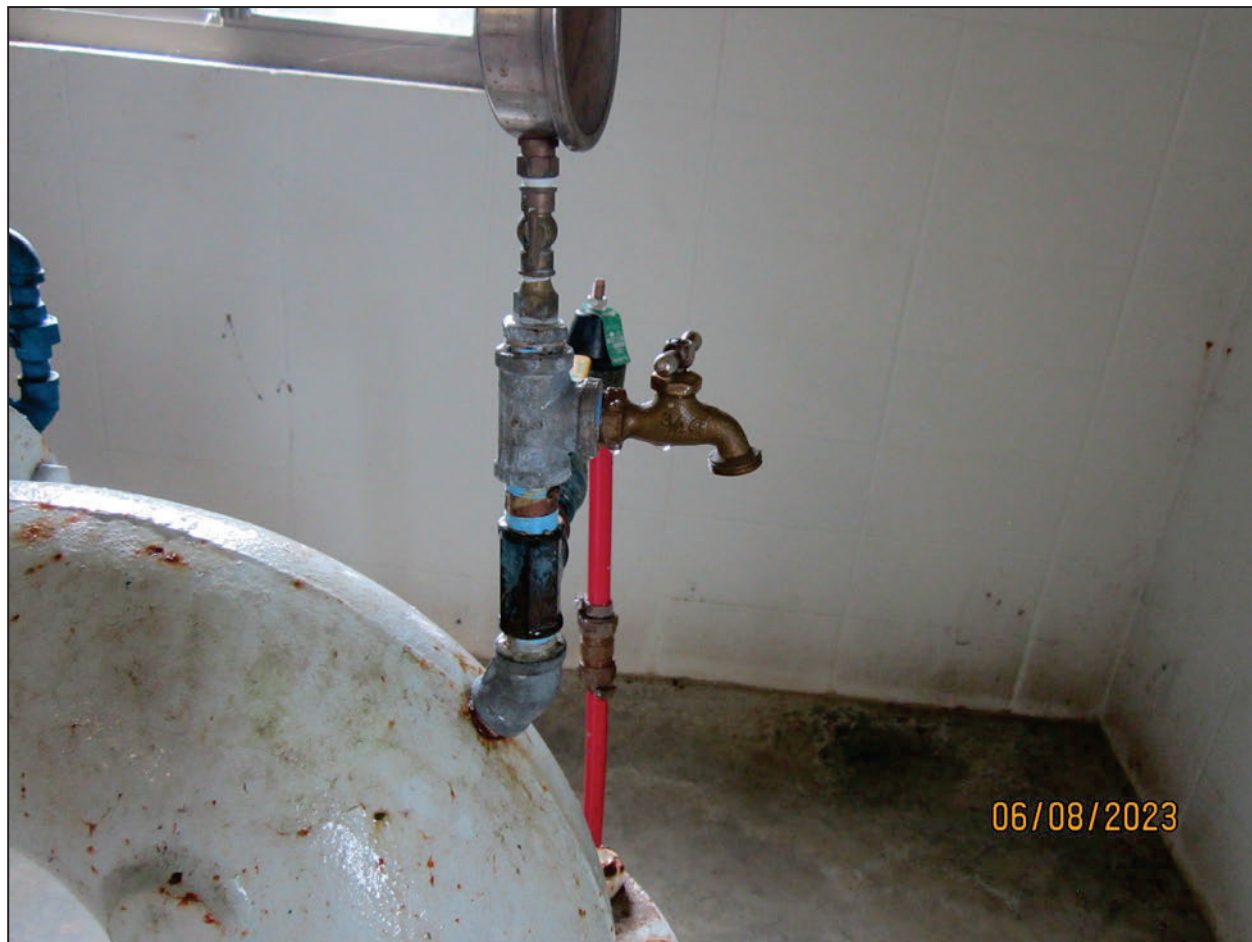
Photograph 20. Water Treatment Plant, Clear Well Pump Valve House View of a finished water line with a threaded hose tap without backflow protection.
