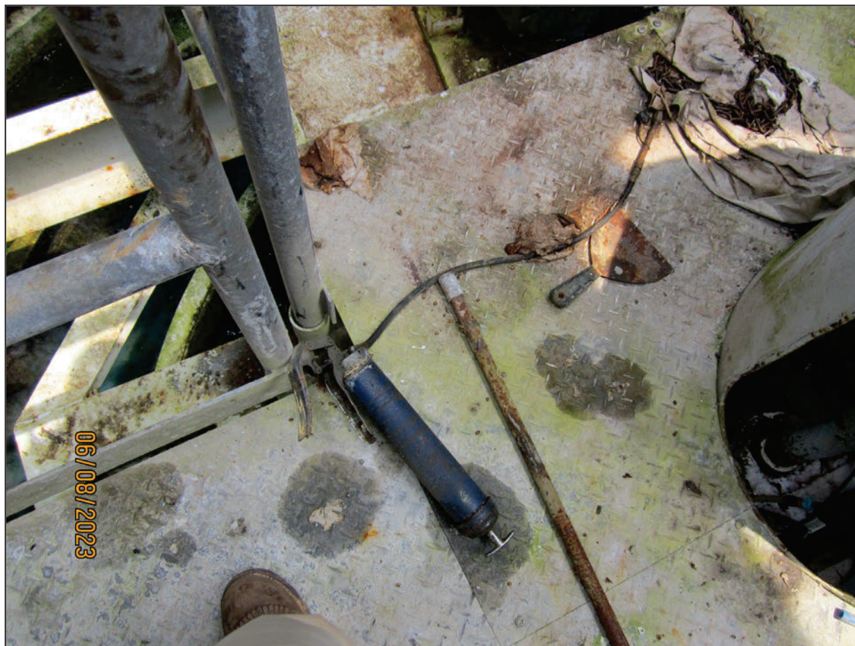
Photograph 12. Water Treatment Plant, Clarifier View of the center of clarifier operational deck. There were maintenance materials and debris, including a grease gun on the deck.
