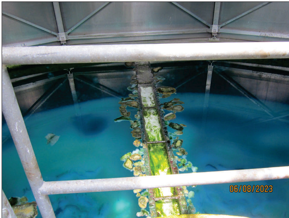
Photograph 11. Water Treatment Plant, Clarifier Alternate view of the top of the clarifier. There were heavy solids, bio-growth, and debris throughout the unit.
