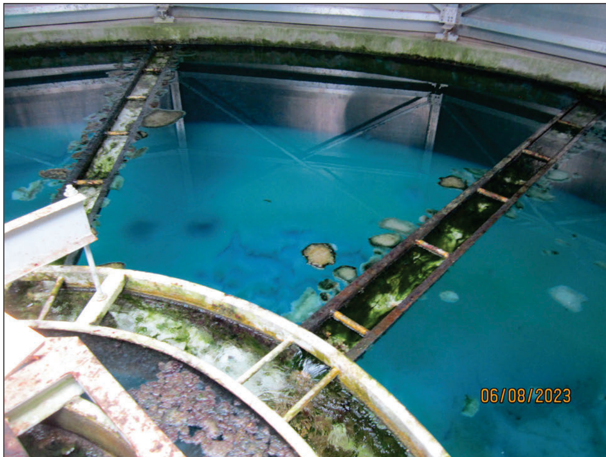
Photograph 9. Water Treatment Plant, Clarifier View of the top of the clarifier. There are heavy solids, bio-growth, and debris throughout the unit, including the troughs delivering produced water to the filters.
