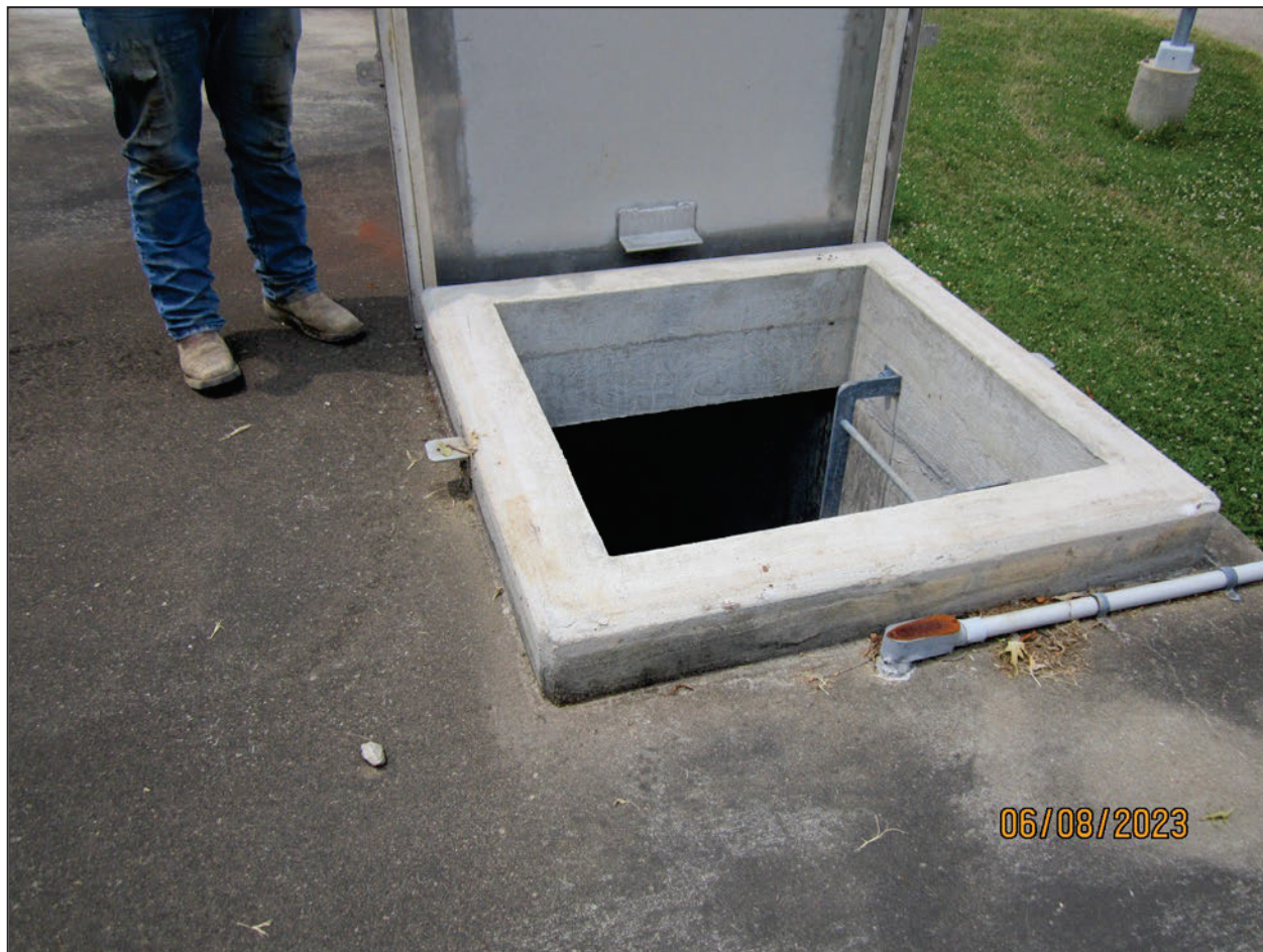
Photograph 17. Water Treatment Plant, Clear Well View of one of the hatchways to the clearwell. The hatch had a shoebox top cover and some seal tape on the cover. However, it is unclear if the tape maintained a sanitary seal.
