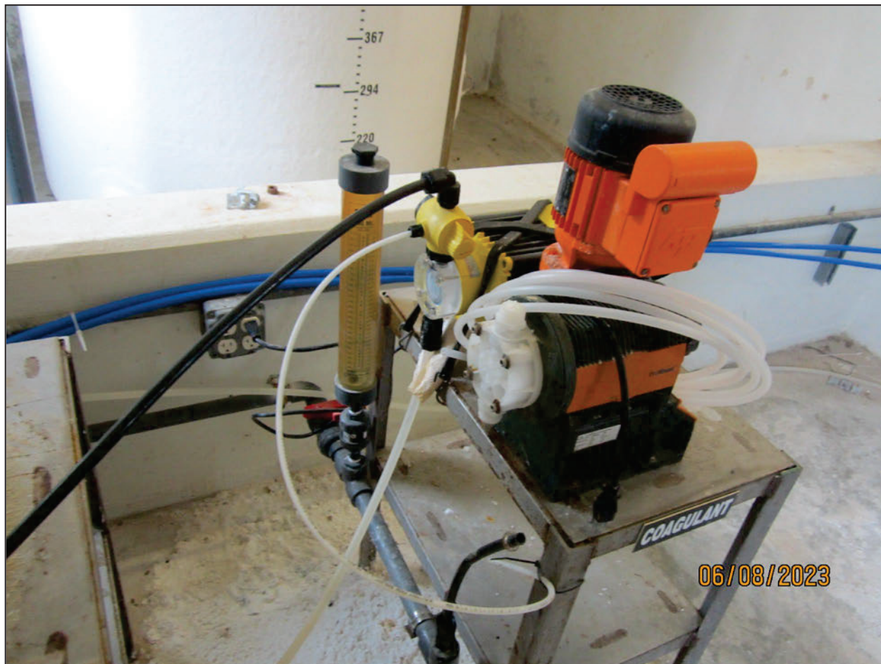
Photograph 14. Water Treatment Plant, Chemical Storage and Pump Area View of a replacement chemical pump positioned with bungee cords at one of the coagulant pump stations. Various tubing and piping systems in the chemical area were disconnected. What appeared to be a new PEX piping (blue) was cable-tied to the containment wall behind the pumping station.
