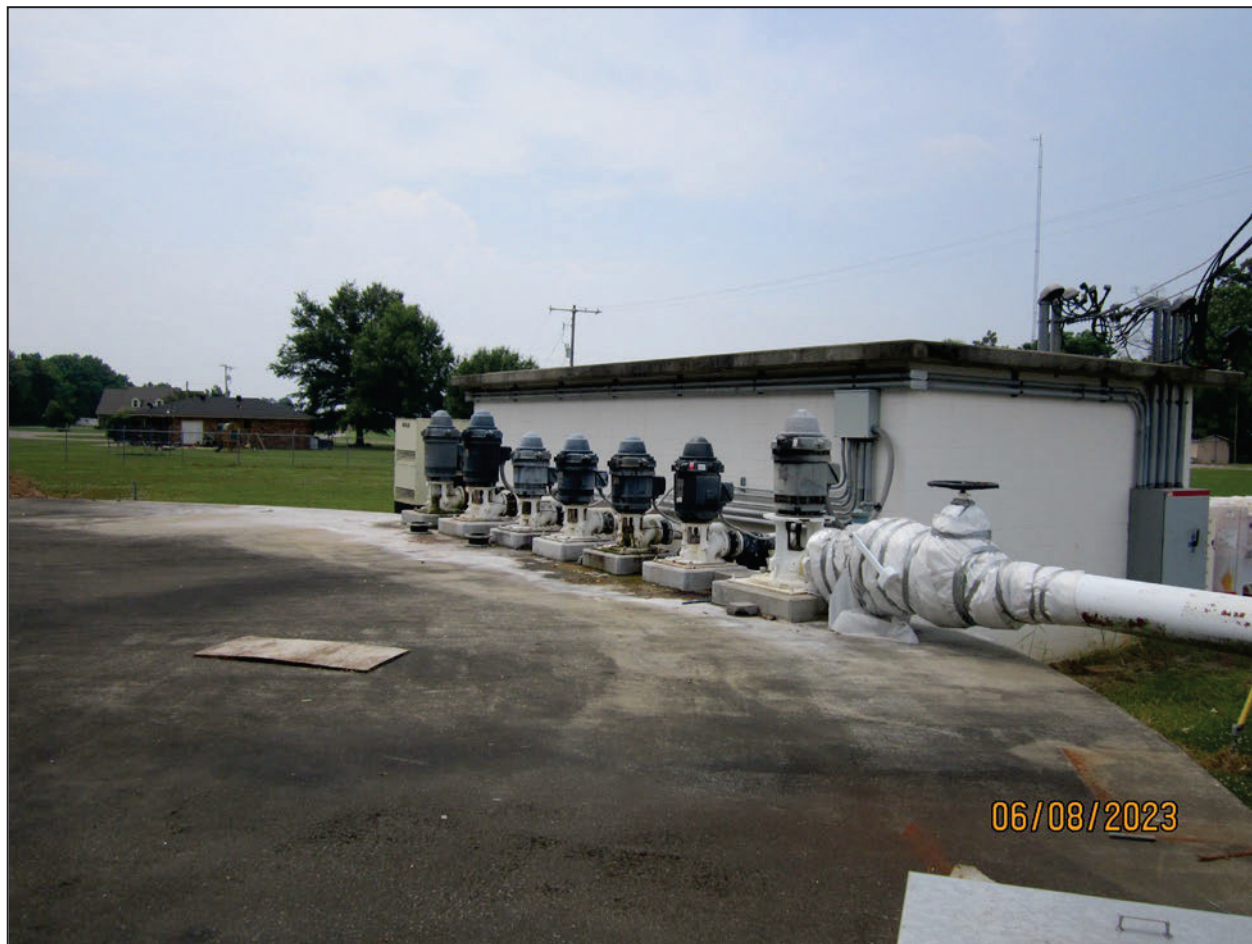
Photograph 18. Water Treatment Plant, Clear Well View of the top of the clearwell, finished water pumps, the area's backup generator, and the valve house supporting finished water supply to the distribution system. Only one of the pump discharges was still wrapped with insulation.
