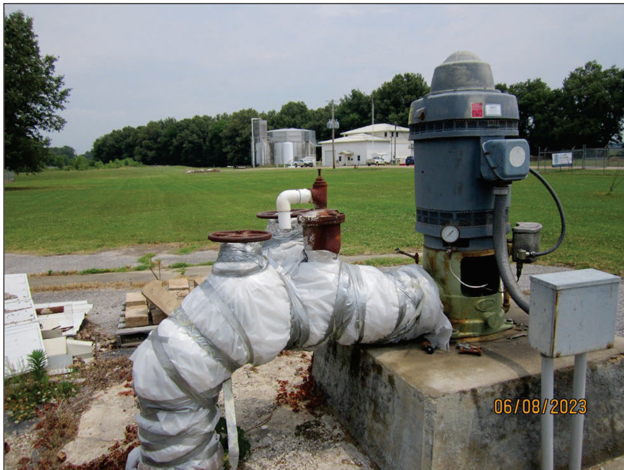
Photograph 4. Well #6 View of Well #6. The well pedestal was located on a concrete pad. Components of the raw water lines were wrapped in insulation. The PVC line from the air relief valve didn't have an external screen. It's unclear if there was an internal screen.
