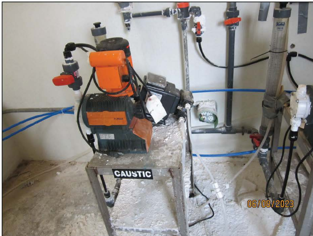
Photograph 15. Water Treatment Plant, Chemical Storage and Pump Area Alternate view of a replacement caustic chemical pump positioned behind failed pump at one of the stations. Dried chemical debris was observed on the floor, pump pedestals, tubing connections and electrical outlets. The caustic soda was a sodium hydroxide, 50% solution. What appeared to be new PEX piping (blue) was cable-tied to the wall behind the pumping station.
