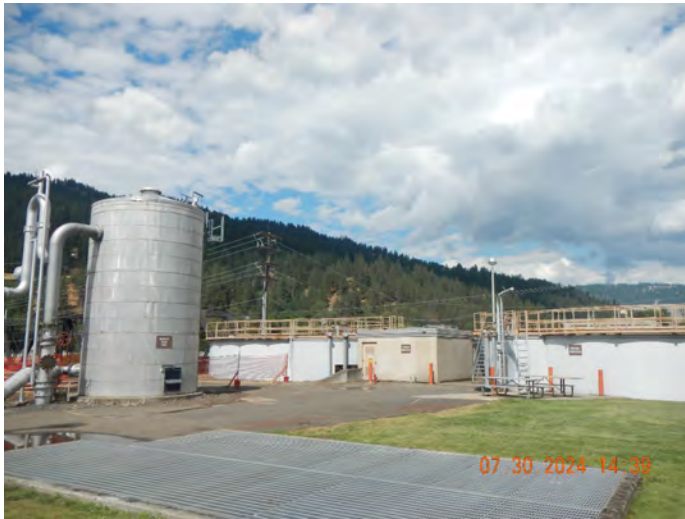
Photo #:03 (DSCN3825) Description: Facing north, photo of System I digesters and nursery head tank
