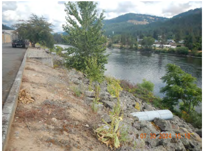
Photo #:12 (DSCN3834) Description: Facing east, photo of southern perimeter along mainstem Clearwater River. Overflow discharge pipes.
