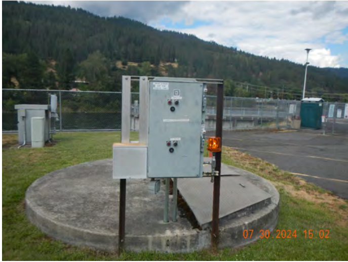
Photo #:09 (DSCN3831) Description: Facing north, photo of a sump pump utilized for the OLSB.
