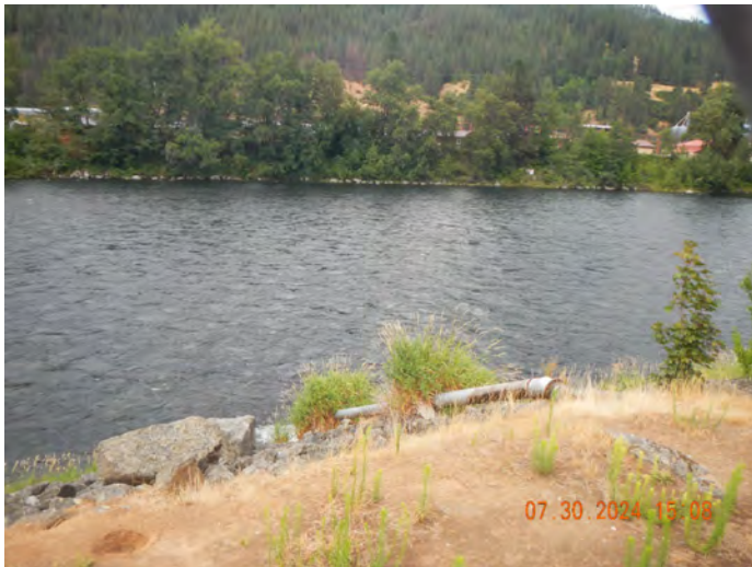
Photo #:11 (DSCN3833) Description: Facing north, photo of Outfall 003 from the OLSB to the North Fork Clearwater River.
