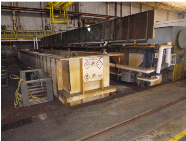
Photograph 30: Treatment and rinse tanks.
