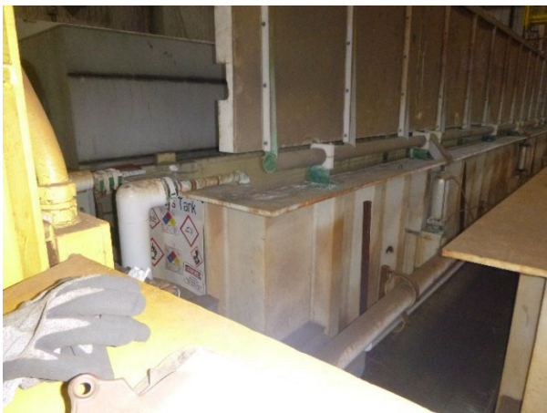
Photograph 31: Treatment and rinse tanks.
