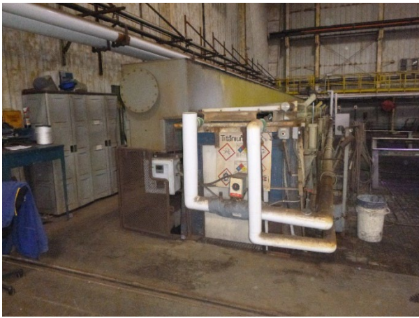
Photograph 29: Treatment and rinse tanks.
