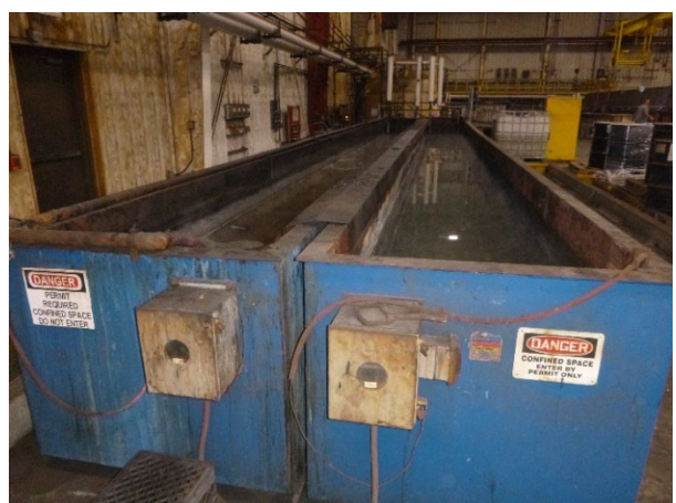
Photograph 28: Treatment and rinse tanks.
