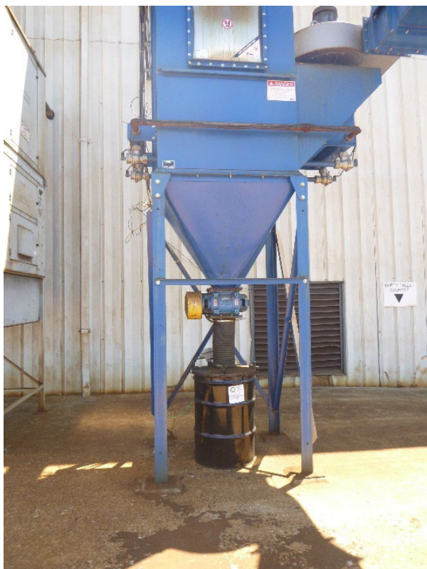
Photograph 38: Recyclable waste accumulation.
