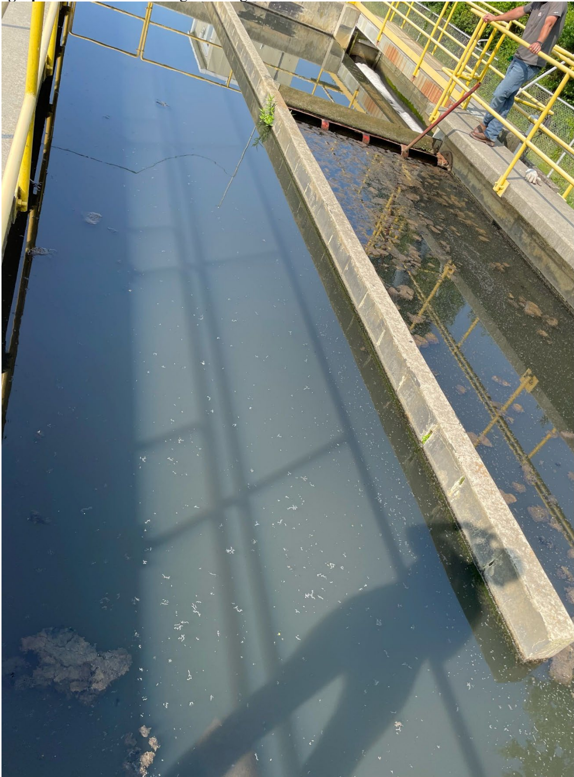
Photograph 5: Bubbles and sludge bulking was observed in the chlorine contact chamber.
