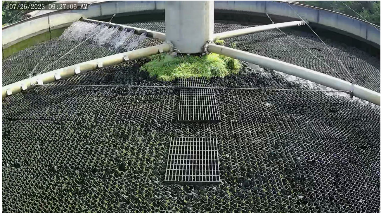
Photograph 4: Vegetative growth was observed on the trickling filter via the facility cameras.
