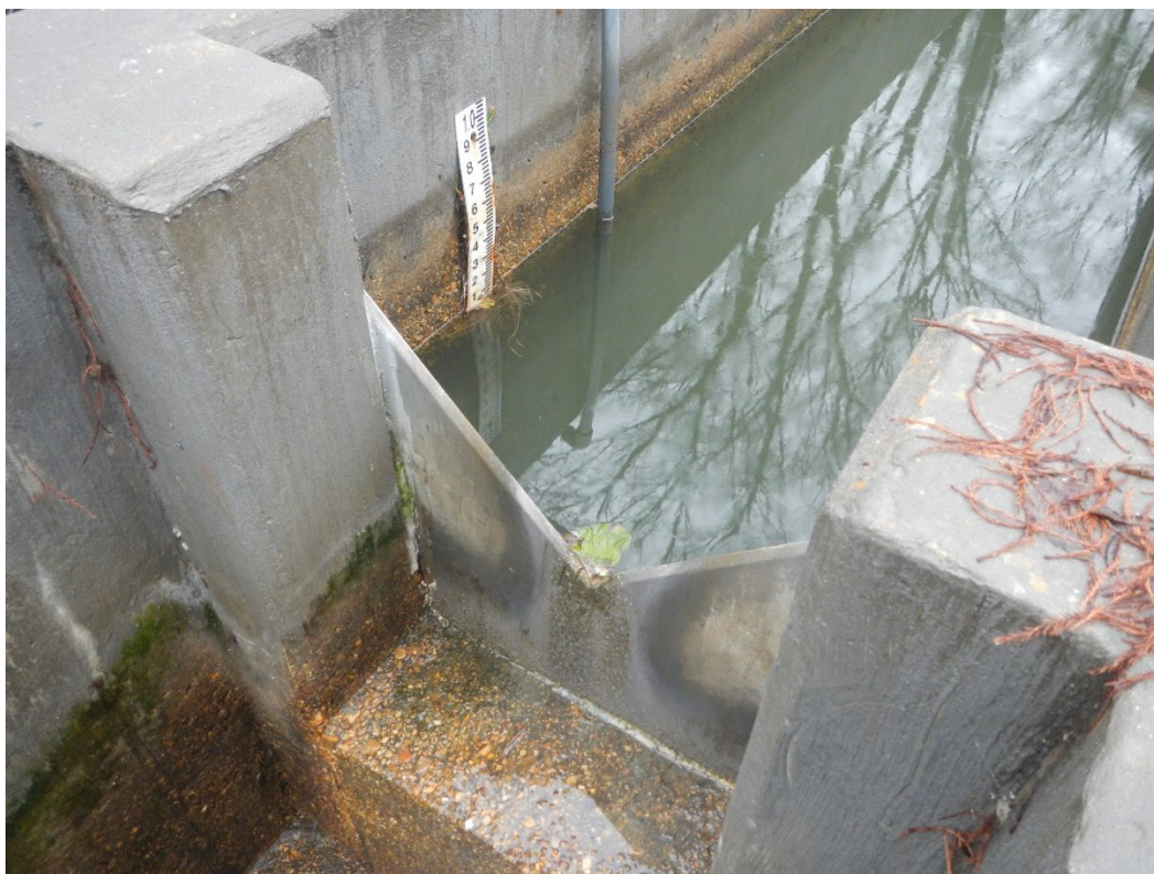
Figure 9: Effluent V-notch weir with staff gauge.
