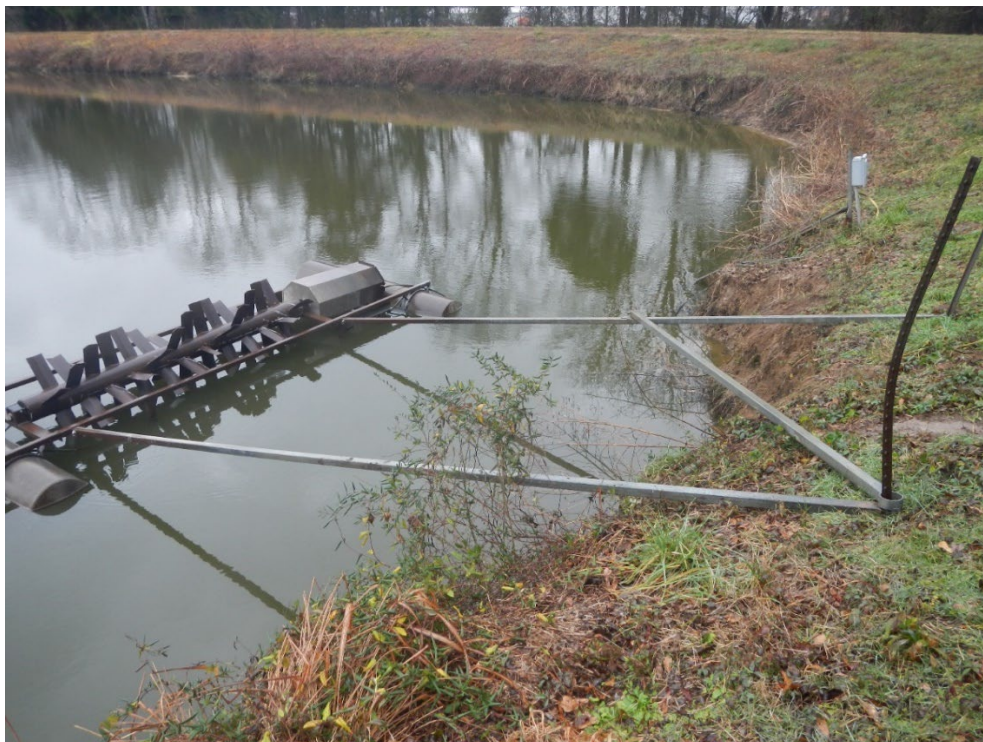
Figure 12: Lagoon aerator was not operational.
