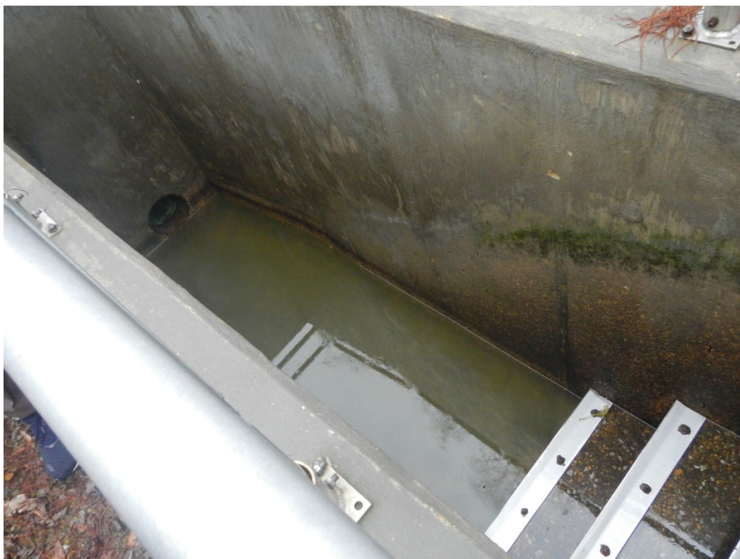
Figure 10: Effluent step aeration cascade where sample is taken.
