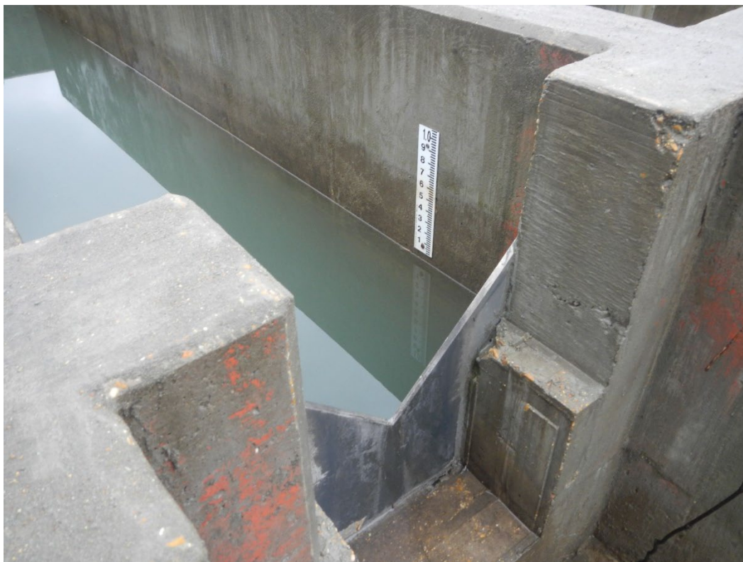
Figure 5: Effluent V-notch weir with staff gauge.
