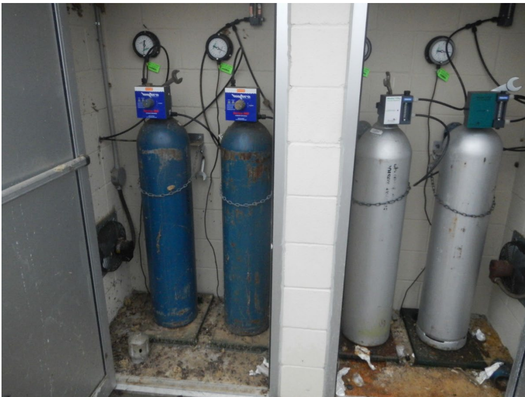
Figure 4: Chlorine (left) and sulfur dioxide gas (right) in shelter on site.
