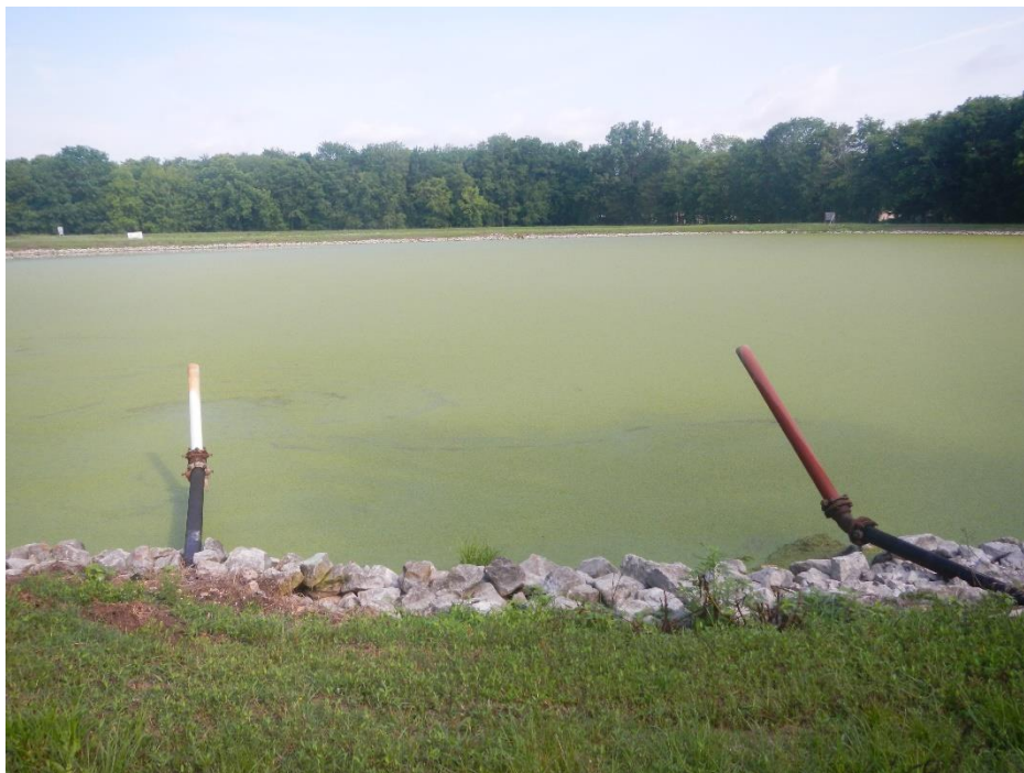
Photo 2. Inlet pipes to Lagoon 01. Lagoon is covered in duckweed.
