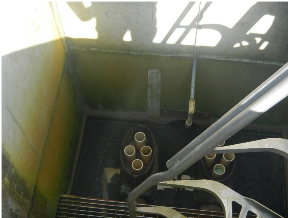
Photo 6. Dechlorinators and flow measurement devices at effluent outlet.
