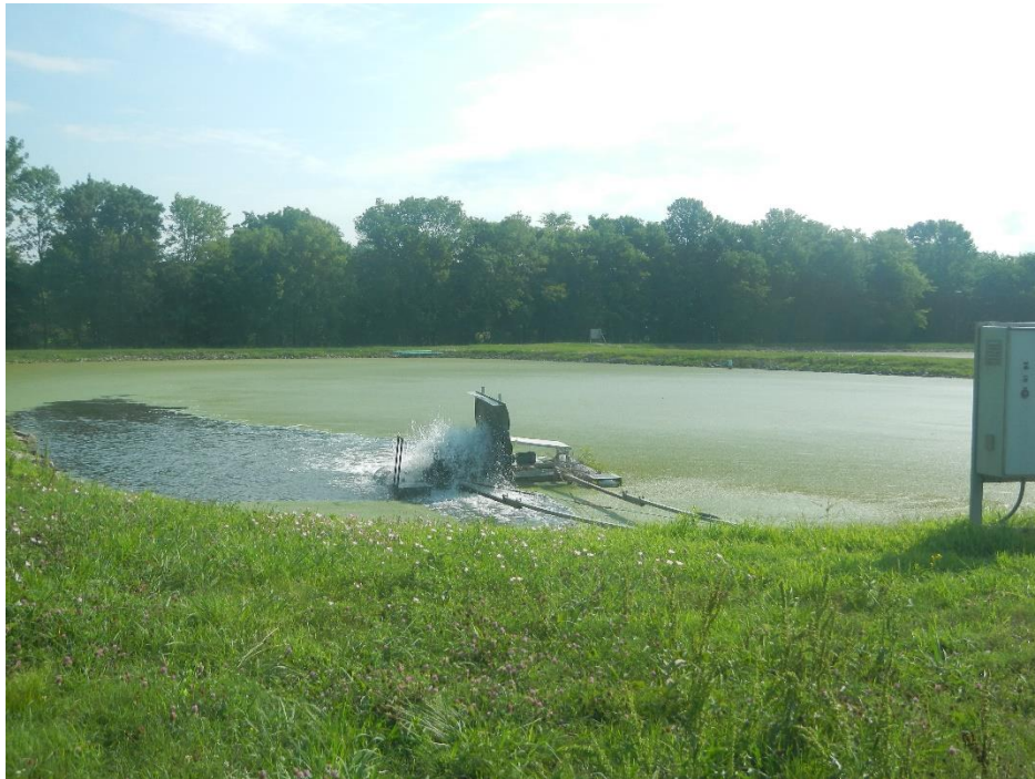
Photo 3. Lagoon 02. Air release for inlet pip seen on opposite shore. Aerator seen functioning in the foreground. Current layout causing possible short circuiting as evidenced by algae growth seen in back half of the lagoon.
