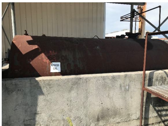
Picture 8: 1000 gallon Used Oil Tank with Secondary Containment (Terminal Plant #2)
