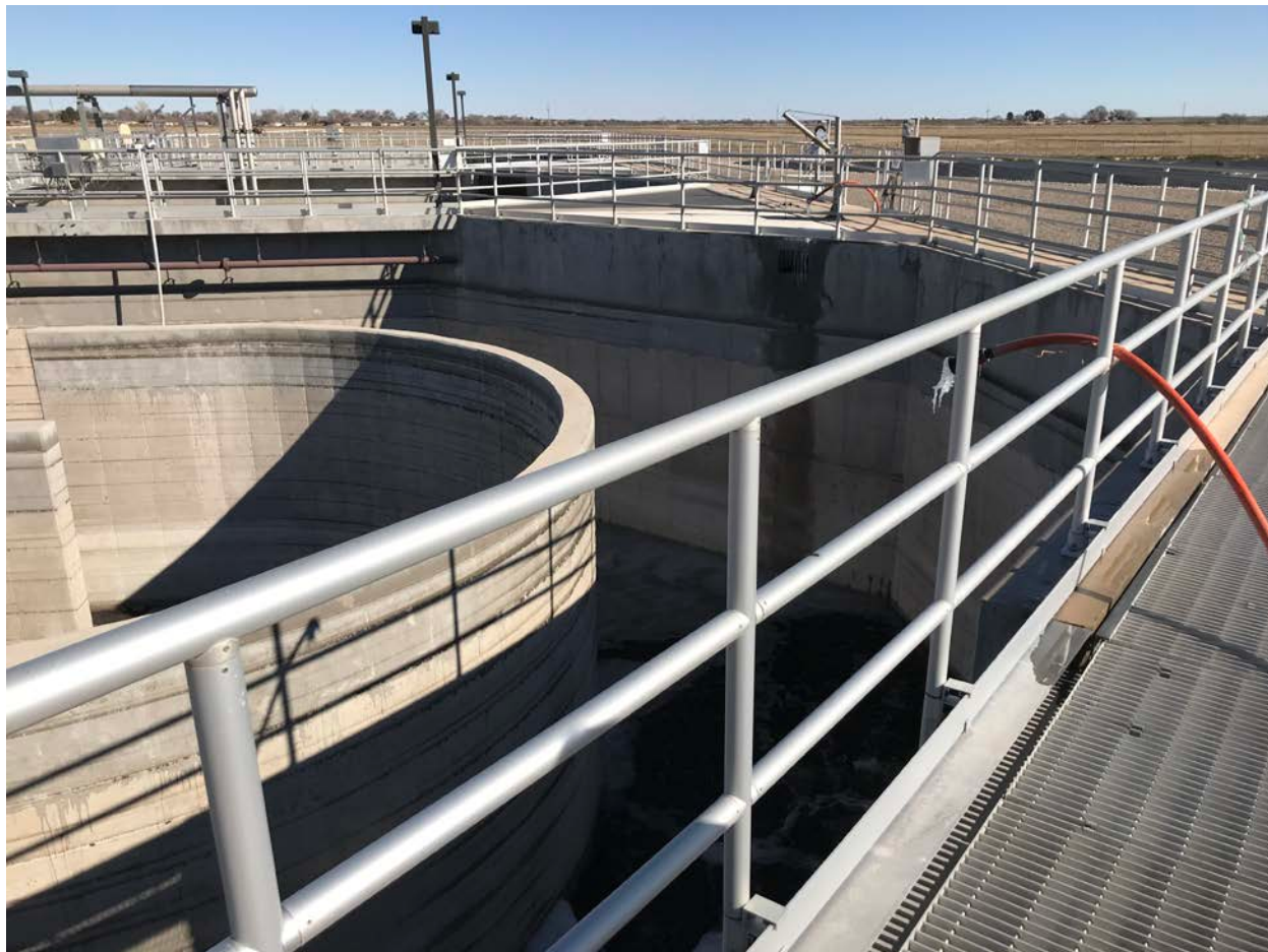
Partial interior view of the WWTP's #1 oxidation ditch or "racetrack" coming offline for cleaning and maintenance. February 26, 2020 9:00 AM (DSCN176) (Photographed by D Esparza).
