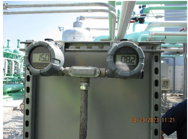
Photo 6: Tank level gauges.
