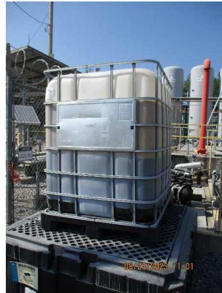
Photo 2: Oily water tote with no label.
