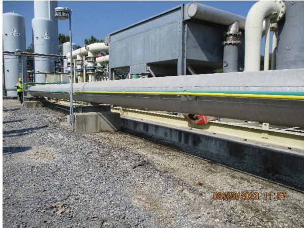
Photo 1: Skid system for turning landfill gas into clean natural gas.
