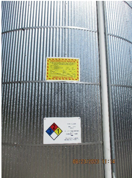
Photo 5: Hazardous waste labels, content information, and indication of the hazard of the contents posted on the tanks.
