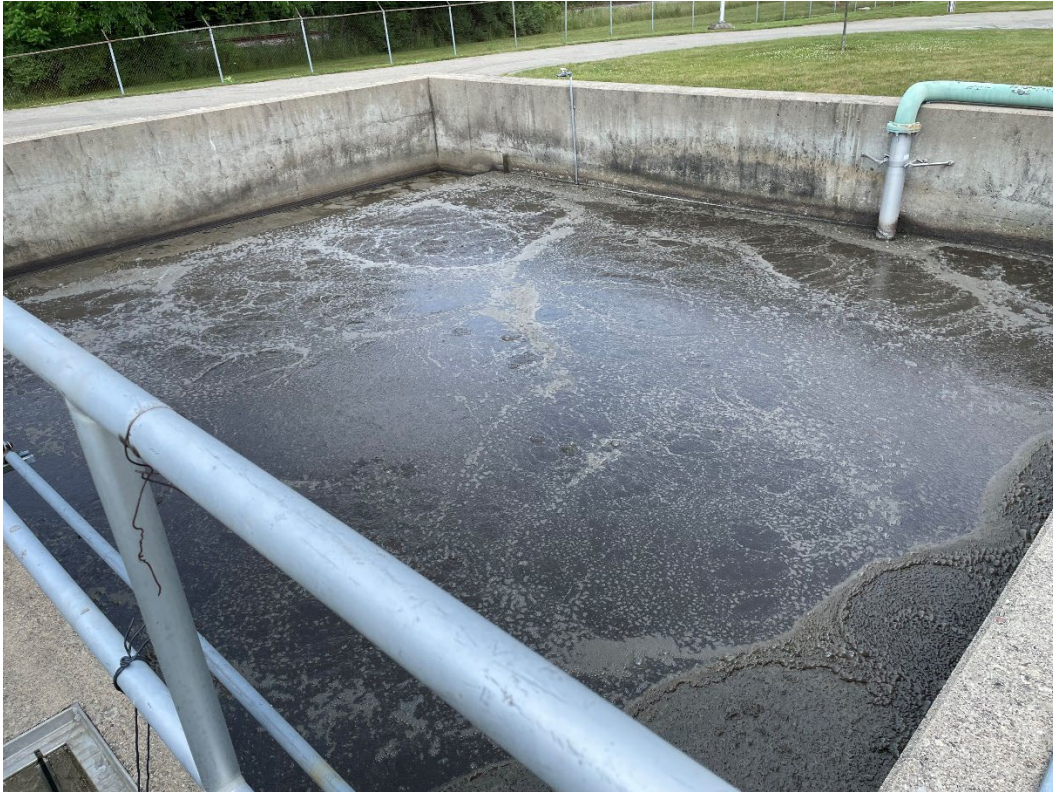
Photo #5. The color of the MLSS in the aeration tank was observed to be dark grey.
