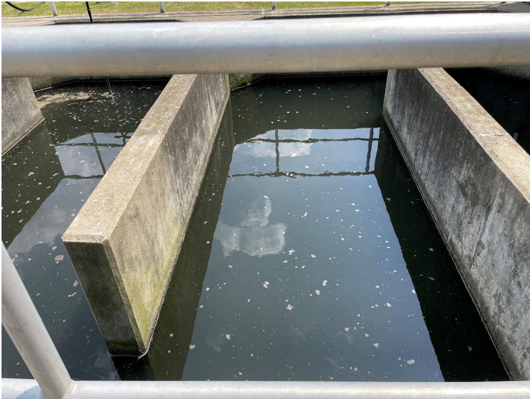
Photo #7. Solids were observed in the polishing chambers.
