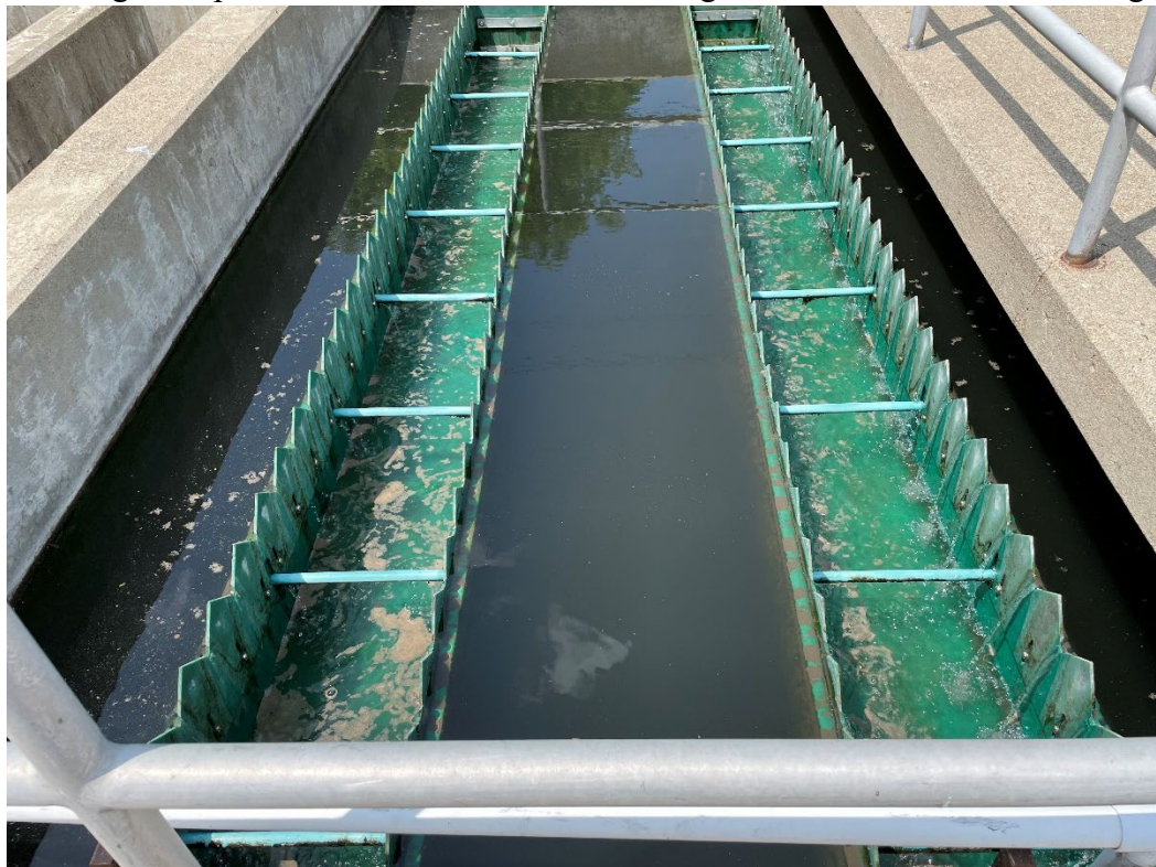
Photo #6. Sludge and pin floc were observed overflowing into the clarifier effluent trough.
