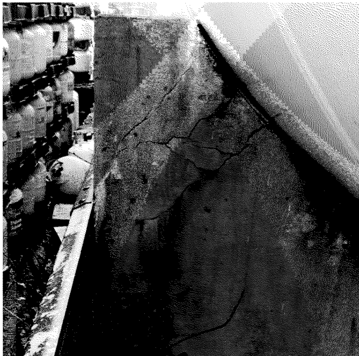
Tank support system in poor repair.
