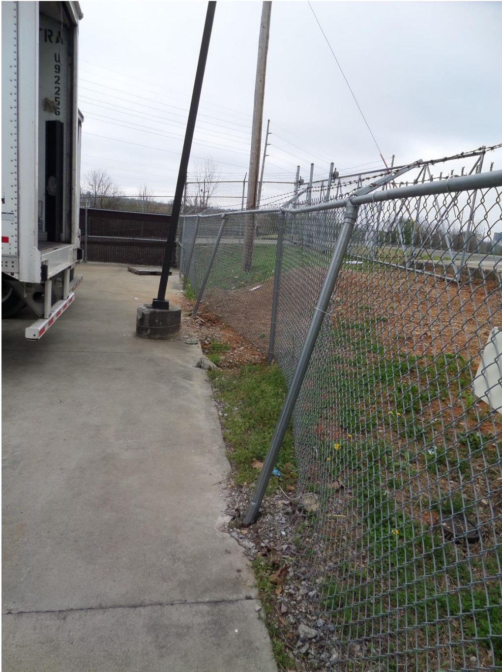
Photo 22: Fence in poor condition.
