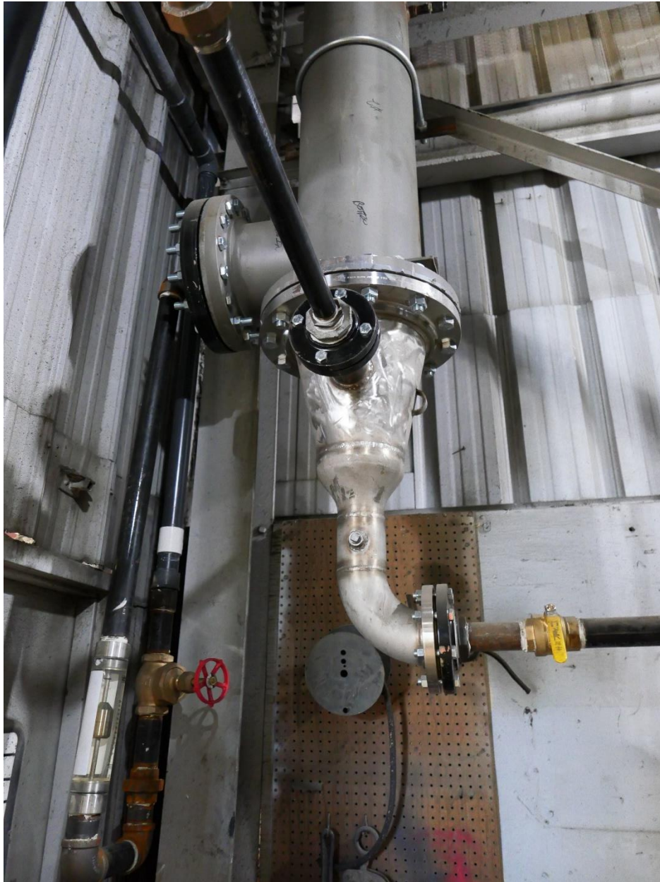
Photo 9: Luwa® Solvent Recovery Unit, missing tagging of connections, flanges, etc tags for equipment.
