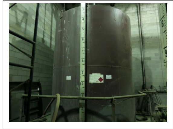
Metal Coaters. Solvent Storage Room. 90-day accumulation tank. Inspectors observed the tank labeled empty on 12/17/16. Photograph 18 taken at 12:08 p.m.
