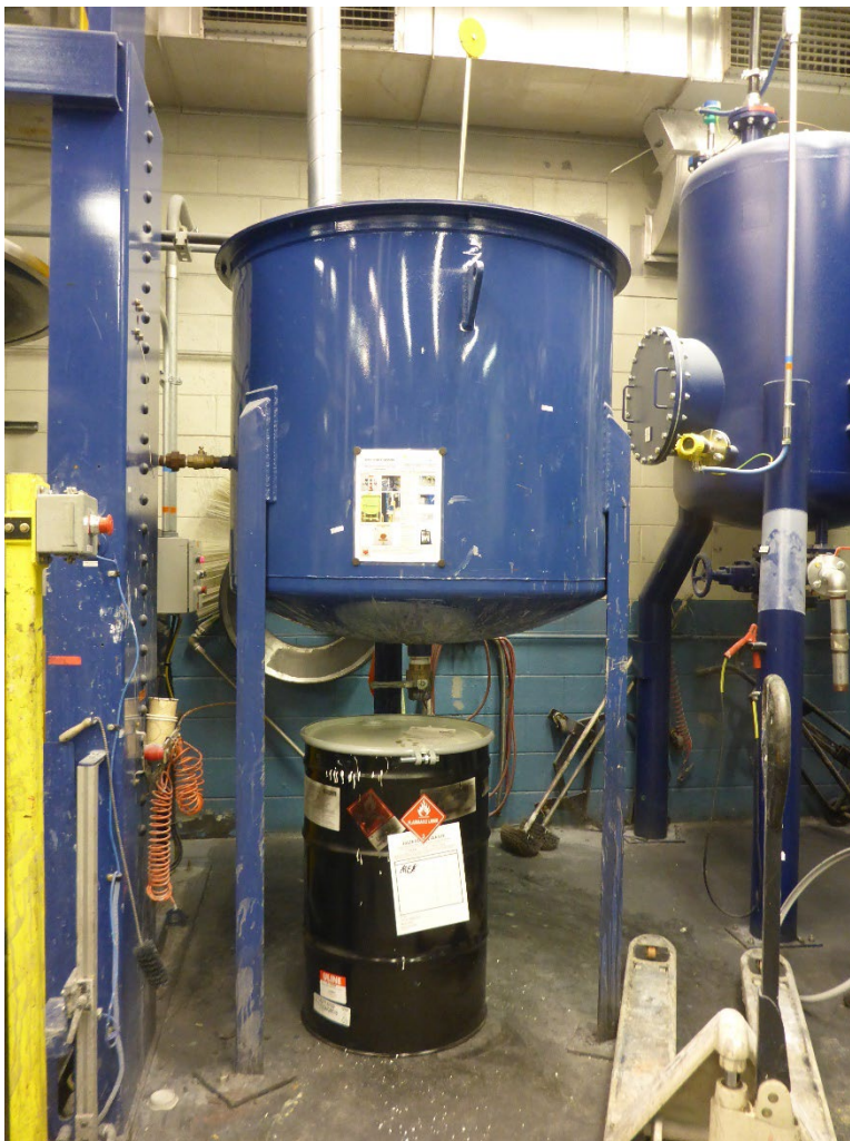
Photo 4: An elevated blue rinse tank used with the CMX-200 Tank Washer and one 55-gallon drum in the CMX-200 Tank Washer SAA in the Mix Room. The drum was closed and labeled hazardous waste Stream A MEK, and it was marked with flammable liquid DOT hazard placard. It is not marked to indicate the contents are toxic.
