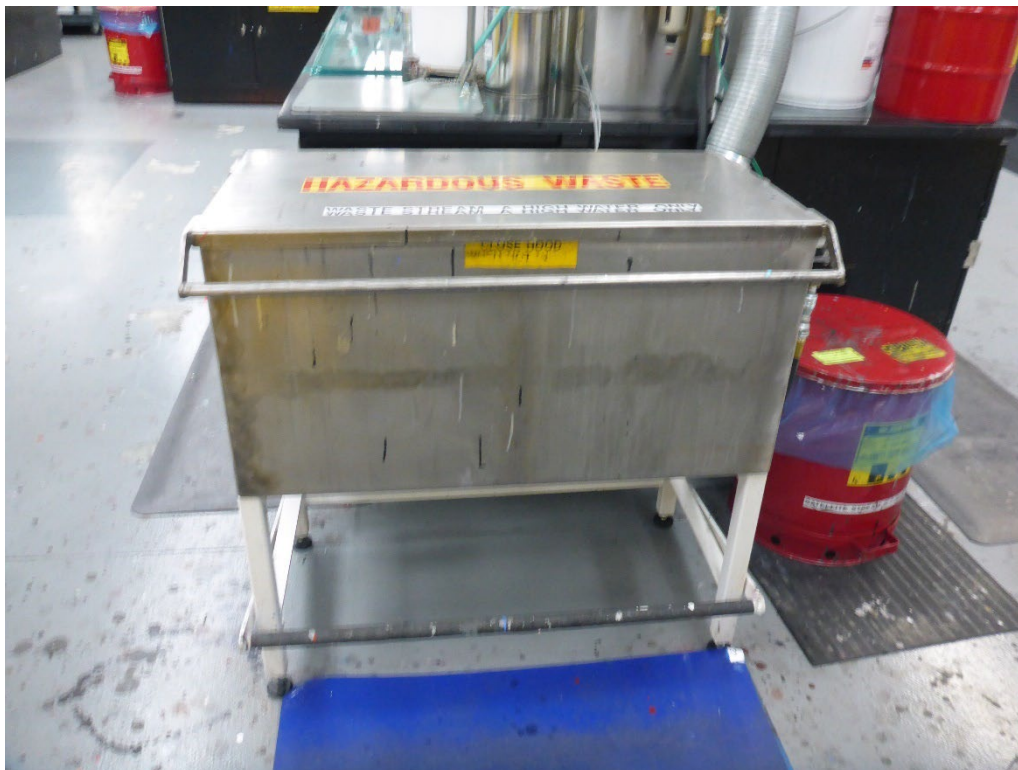
Photo 11: SAA for accumulating hazardous waste Stream A High Water in Liquid Laboratory. The basin is labeled as hazardous waste, but it is not marked with an indication of the hazards of its contents. One 5-gallon bucket of hazardous waste was observed inside the basin, which is connected to the air handling system.
