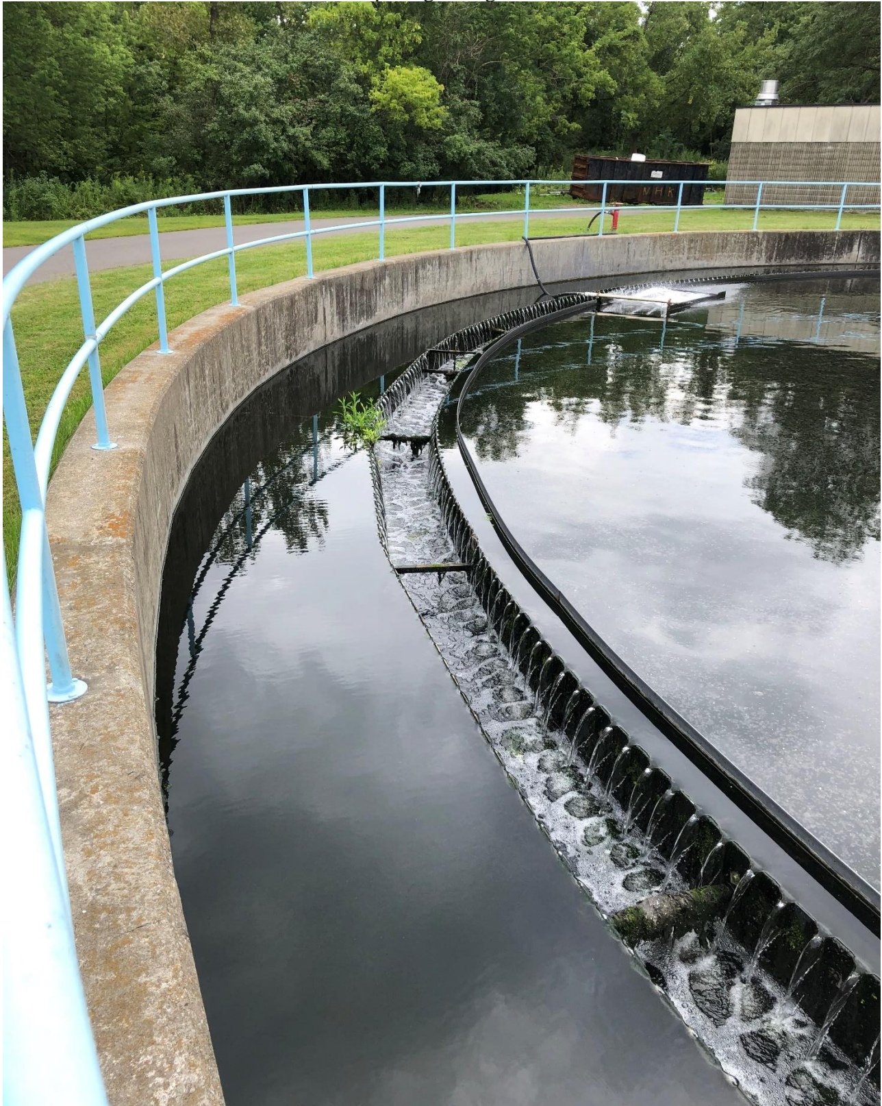
Photo #2: View of a final clarifier with a plant growing in the side.
