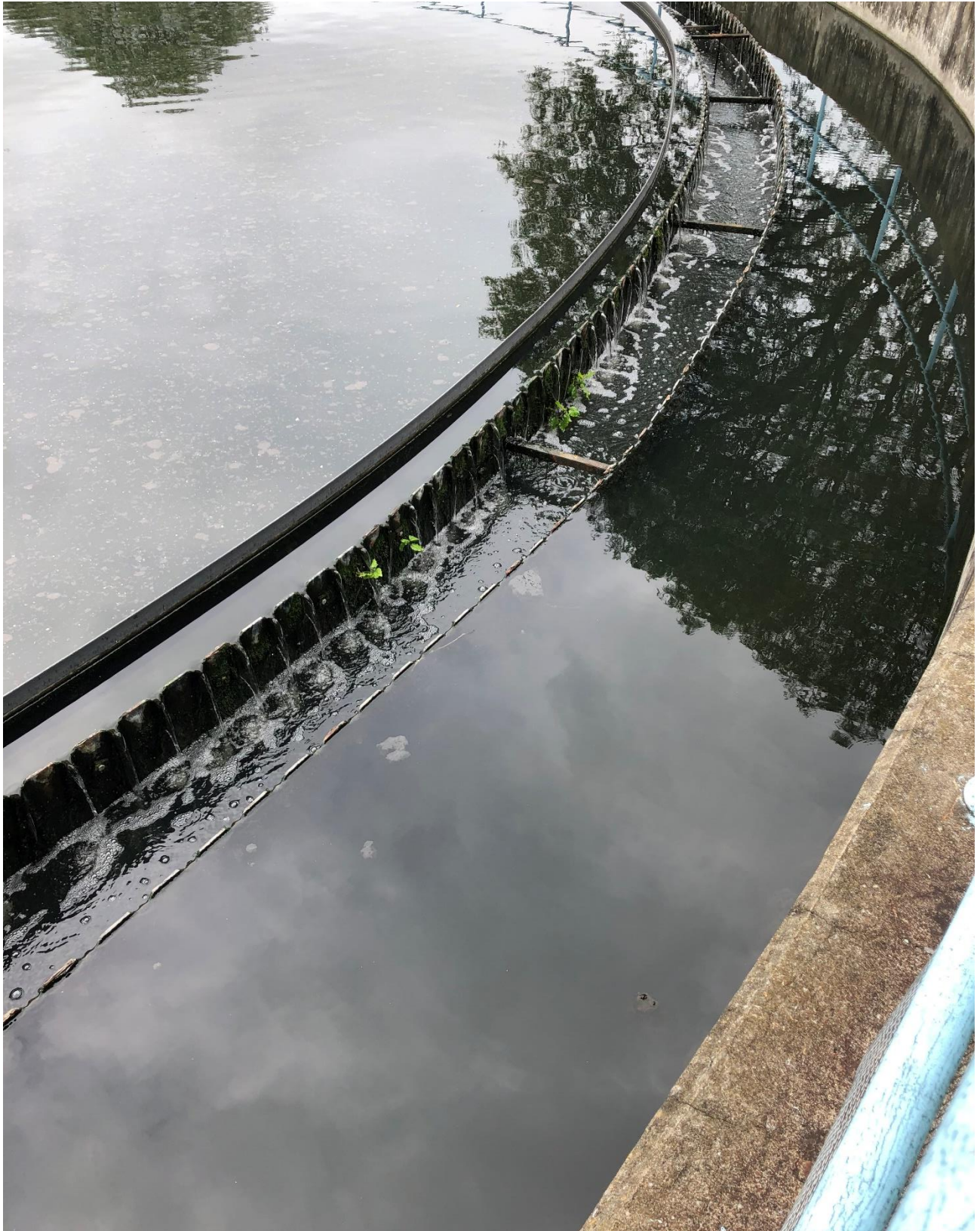
Photo #4: Another view of a final clarifier.
