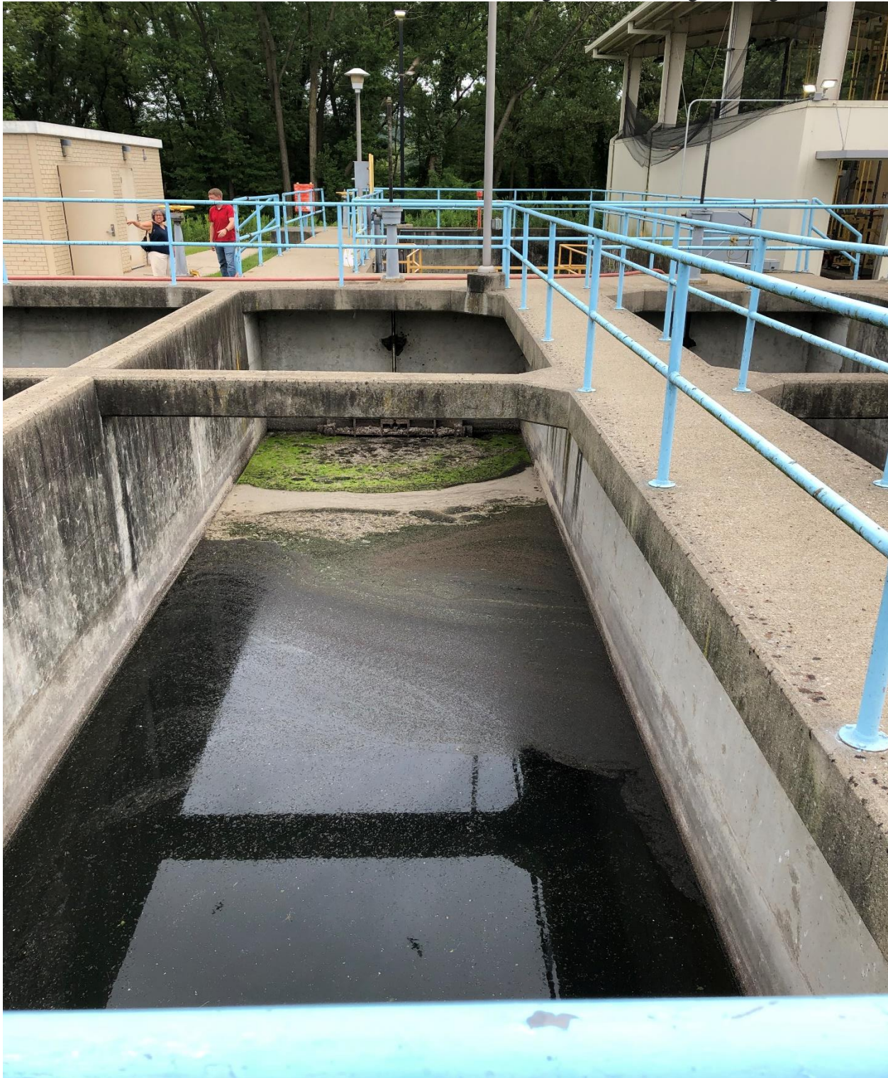
Photo #1: View of chlorine contact tank with solids and algae accumulating at exit gate.
