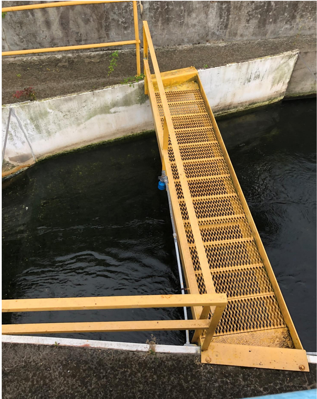
Photo #5: View of the primary flow measuring device, located at the midpoint of the converging section of the Parshall flume.
