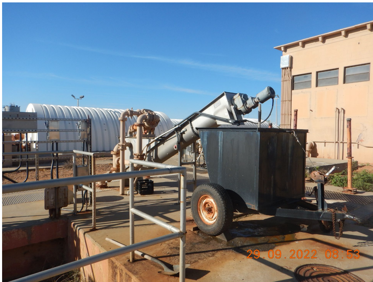
View of the grit screen removal equipment. (DSCN2349) Photographed by D. Esparza
