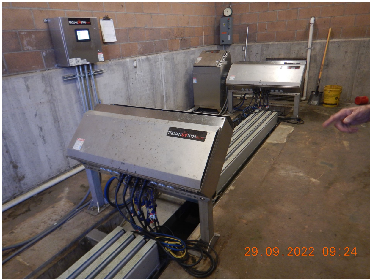
View of the two (2) banks of Trojan ultraviolet (UV) disinfection units included in the 2011 WWTP upgrades. (DSCN2350) Photographed by D. Esparza
