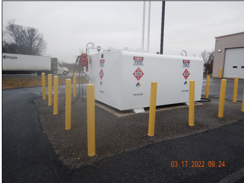
Photograph 7. Township Municipal Building: (DSCN3643.JPG) View, facing west, of the aboveground 500-gallon gas and 1,500-gallon diesel aboveground storage tanks (ASTs). Township representatives stated that they are double-walled.
