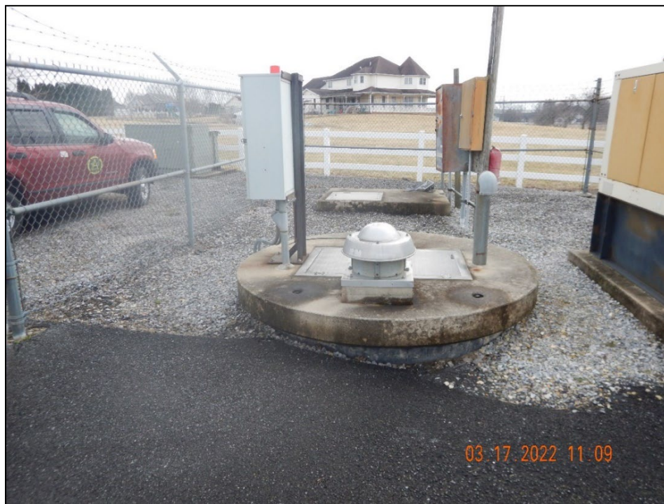
Photograph 36. Lift Station #21: (DSCN3704.JPG) View, facing east, of the Lift Station #21 Jason Drive Pump Station.
