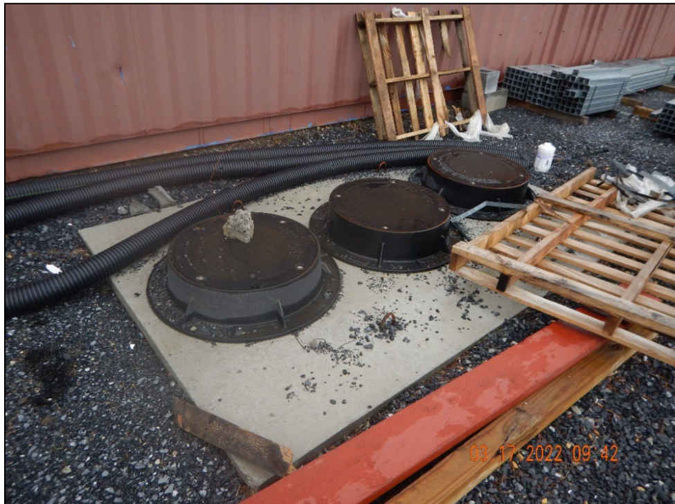
Photograph 16. Township Municipal Building: (DSCN3658.JPG) View of the oil/water separator access outside of the Main Building.
