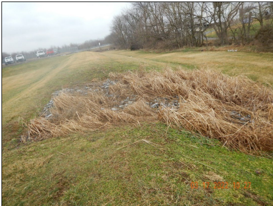
Photograph 28. Vehicle Facility Yard: (DSCN3681.JPG) View, facing west, of the overflow spillway from stormwater basin 3. Vegetation was observed growing in the overflow spillway at the time of the inspection.
