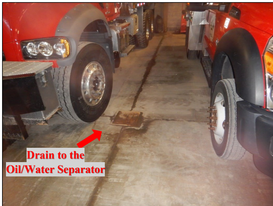
Photograph 12. Township Municipal Building: (DSCN2962.JPG) View of a drain in the first truck and equipment storage garage. The drain leads to the oil/water separator before discharging to the sanitary sewer system.
