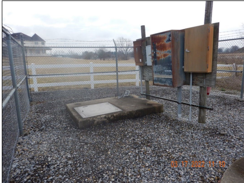
Photograph 37. Lift Station #21: (DSCN3705.JPG) View, facing east, of Lift Station #21 Jason Drive Pump Station, as shown in Photograph 36.
