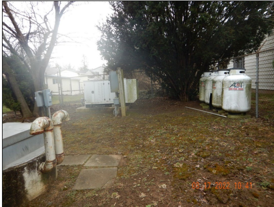
Photograph 31. Lift Station #3: (DSCN3693.JPG) View, facing east, of the Lift Station #3 Grindstone Hill Road (Ryan Lane) Pump Station, as shown in Photograph 30.
