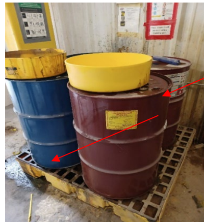
Photo-6 Leak in the SAA (FMJ Area)
