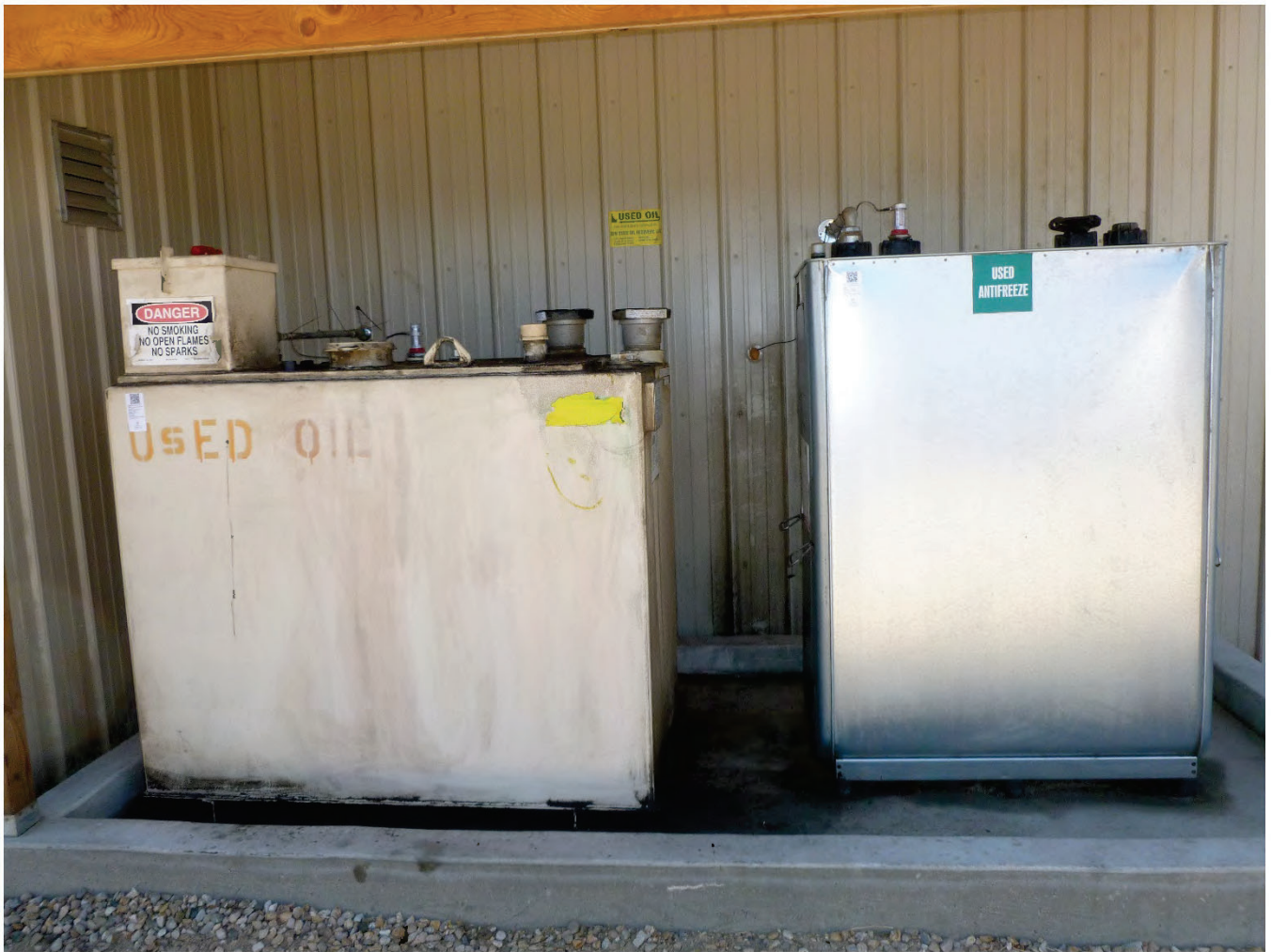
Photo 7 / P1000891 – Used Oil & Antifreeze Tanks
