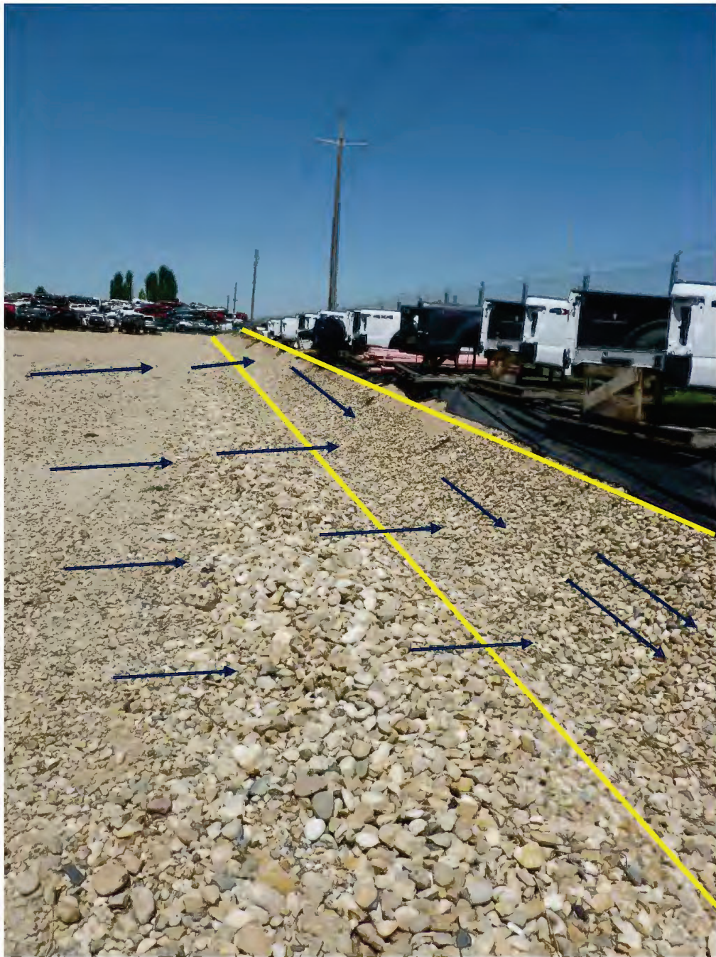
Photo 3 / P1000888 – Rock-lined Ditch
