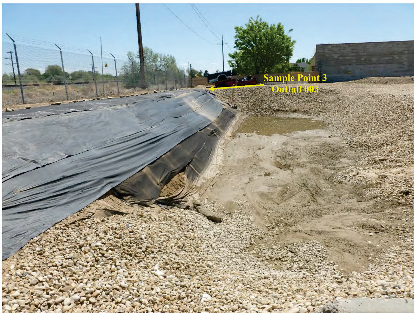
Photo 4 / P1000887 – Retention pond, with liner
