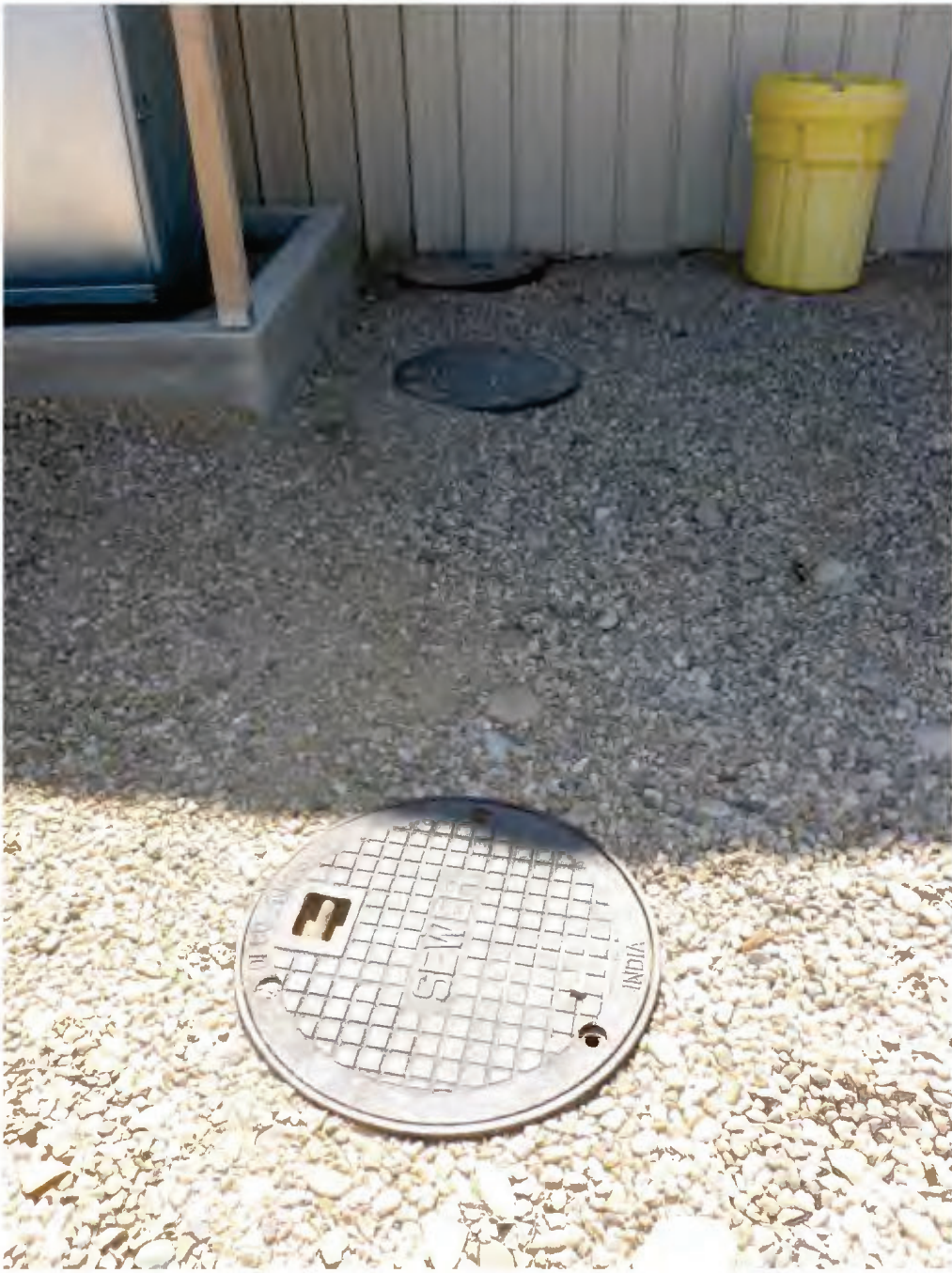
Photo 8 / P1000892 – 3 Chamber Oil/Water Separator
