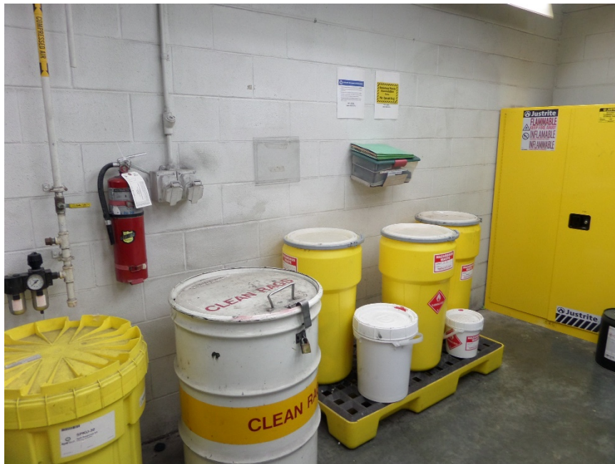
Photograph 8: Hazardous waste containers observed in satellite accumulation area (SAA) 019. All containers were properly closed, labeled, and appeared to be in good condition.
