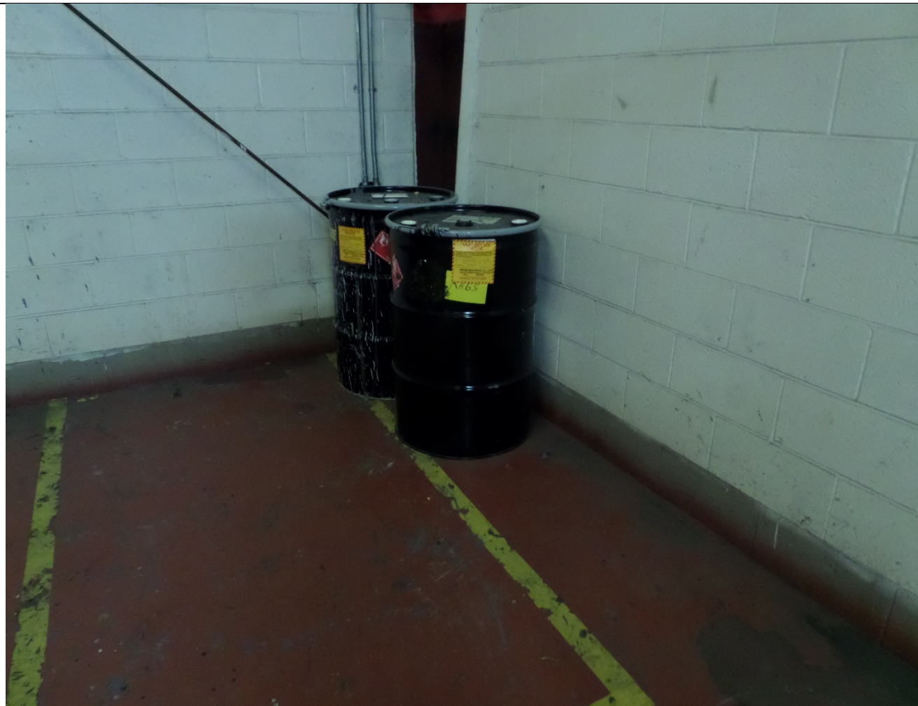
Wilbert. CAA/90-Day or Less Accumulation Area. Observed containers accumulating hazardous waste. Observed the floor epoxy appeared to be deteriorating. Photograph 9 taken at 11:39 a.m.
