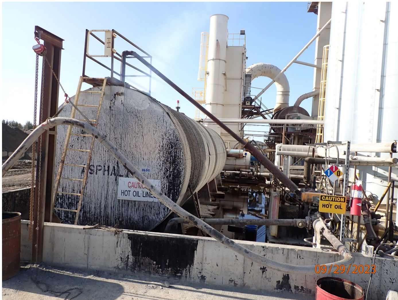
Photo 5 - Asphalt storage tank and secondary containment
