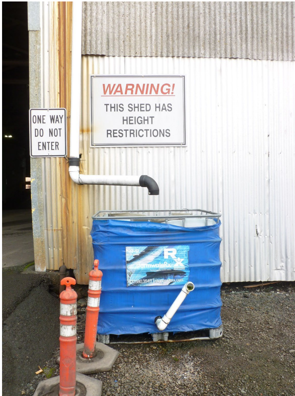
Photo 11 / P1010104 – stormwaterRx™ Zinc Filtration System
